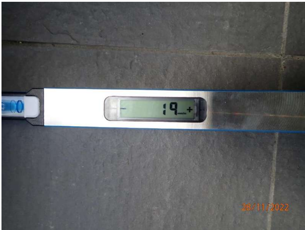
Photograph 96 - Apartment 431B balcony cross fall 1 in 50
