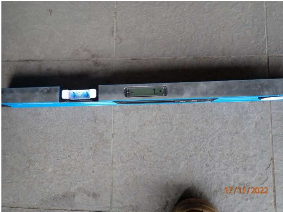
Photograph 11 - Apartment 308A balcony fall 1 in 143
