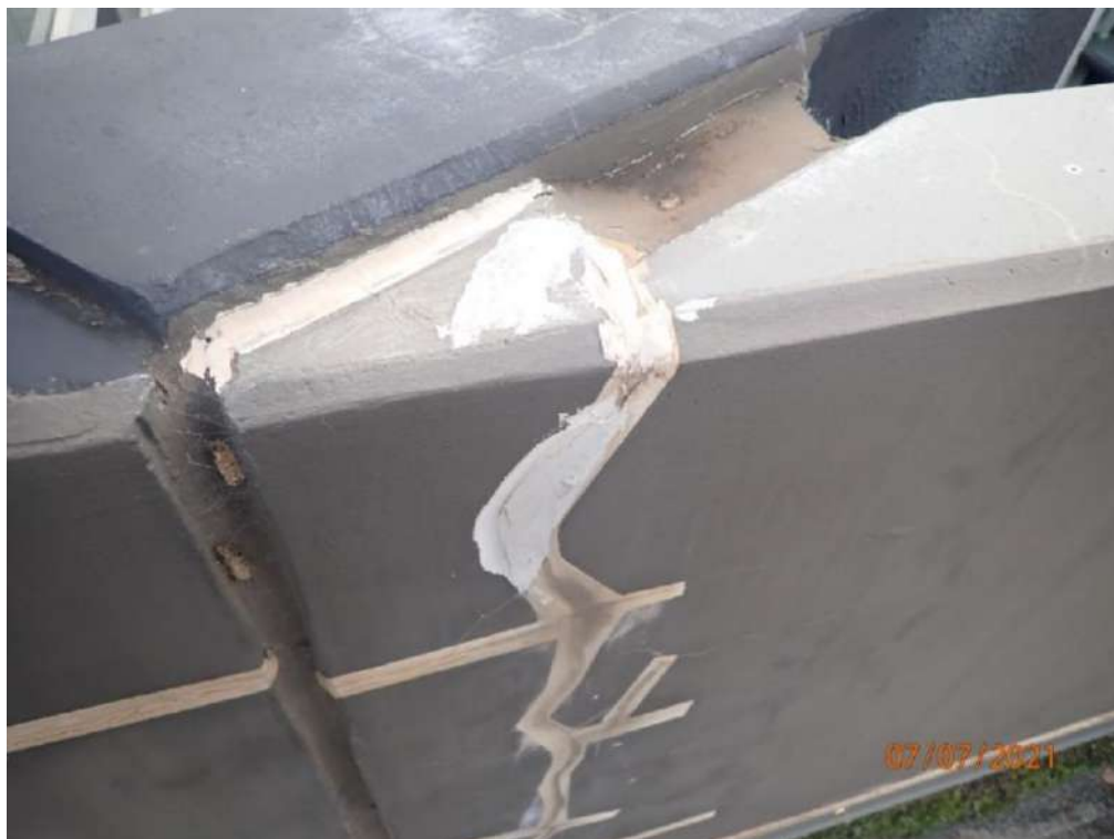
Photograph 106 – Cracking to the concrete wall panels to the north elevation of building A
