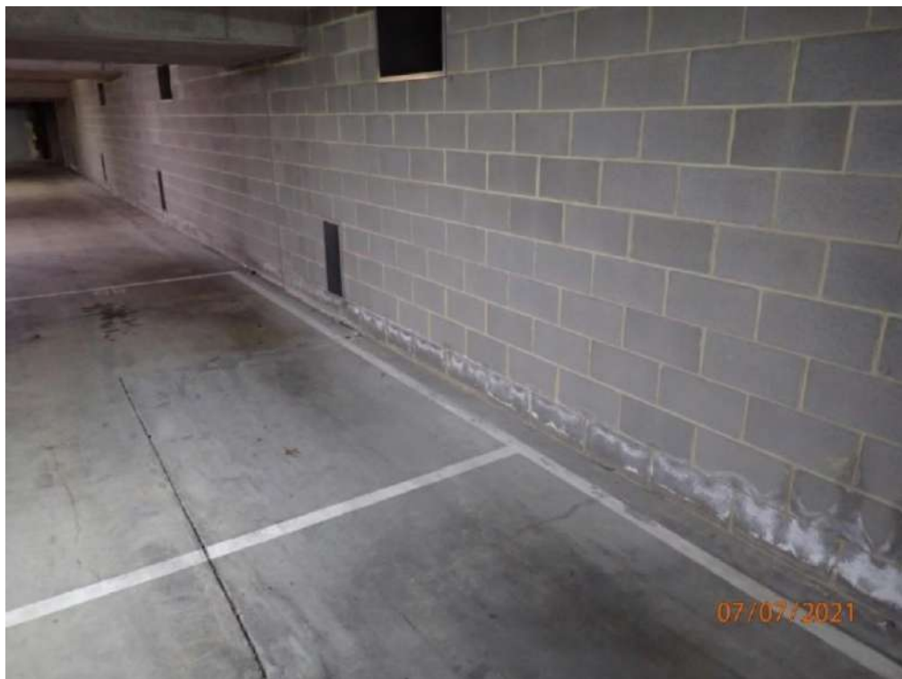
Photograph 86 – Efflorescence to the block walls adjacent the water tanks
