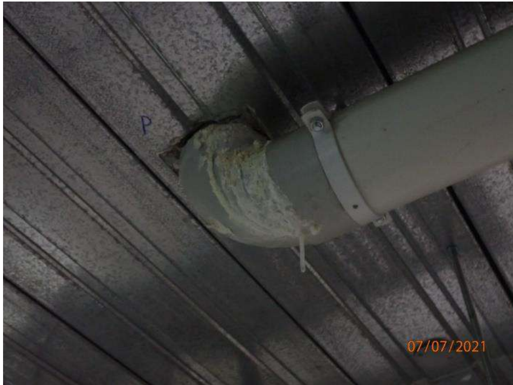
Photograph 15 - Calcification at PVC pipe penetration above carpark 65
