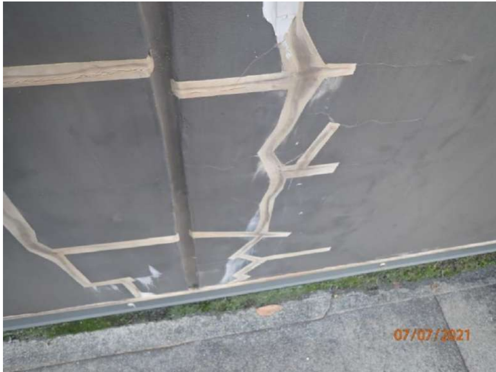
Photograph 107 – Cracking to the concrete wall panels to the north elevation of building A
