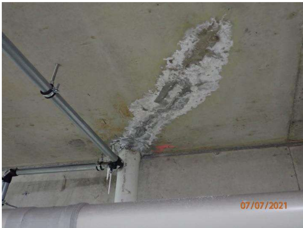
Photograph 62 - Efflorescence, calcium build up and cracking to west end of basement ceiling
