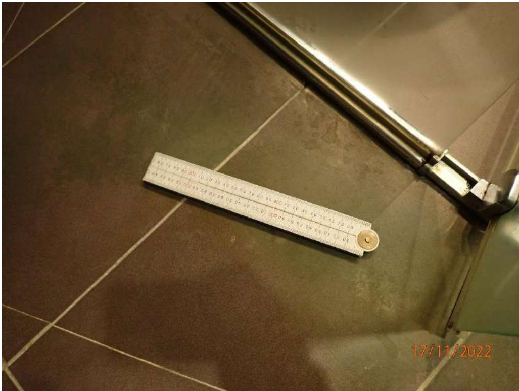
Photograph 31 - Apartment 526B bathroom shower, algae growth on tile surface
