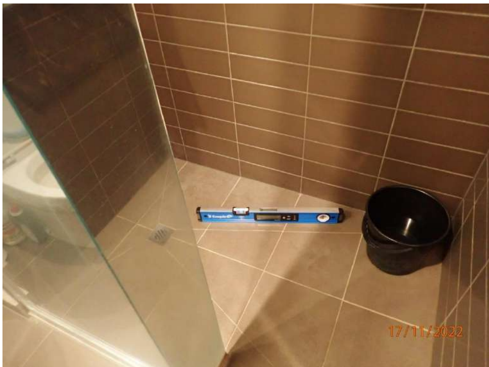
Photograph 6 - Apartment 309A bathroom shower
