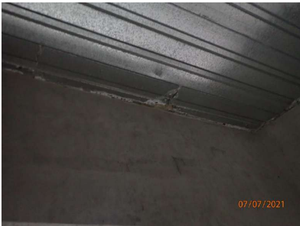
Photograph 4 - Efflorescence and Bondek rusted to carpark 73 southwest corner
