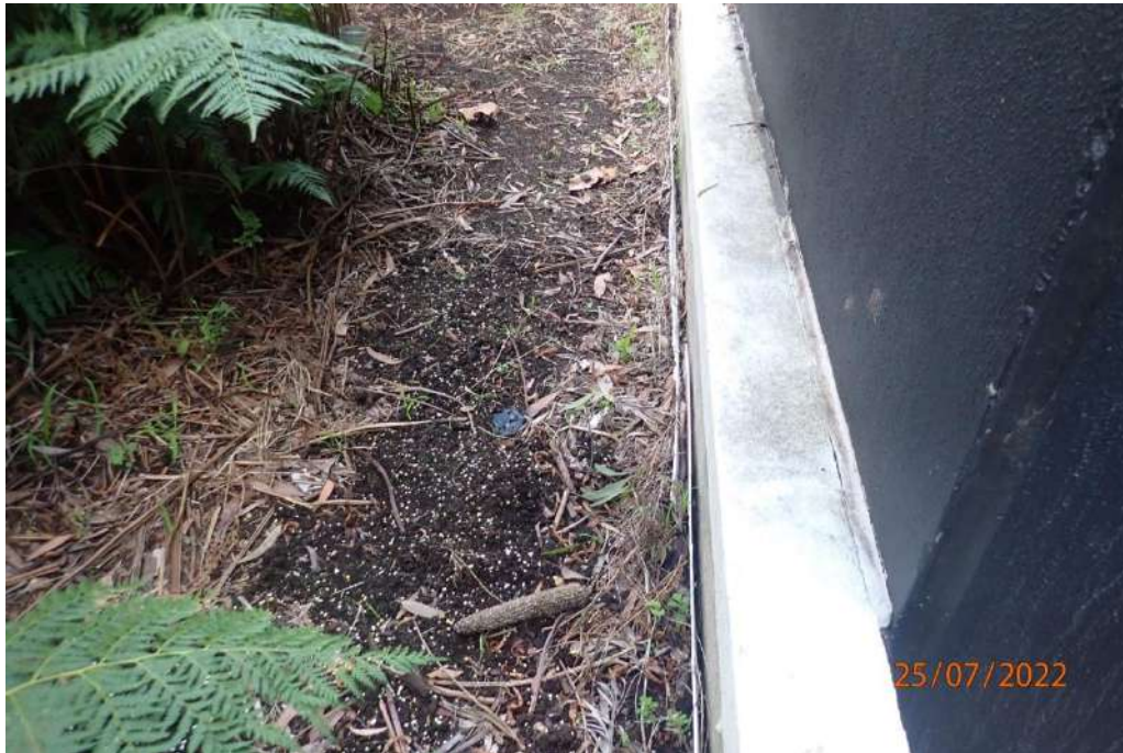
Photograph 147 - Lot 106B/Apartment 116B, west elevation wall and planter box
