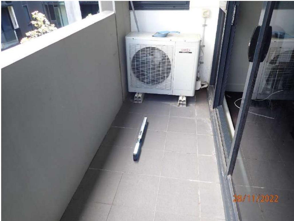
Photograph 89 - Apartment 431B balcony fall
