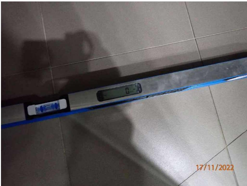
Photograph 34 - Apartment 328B bathroom shower, no fall
