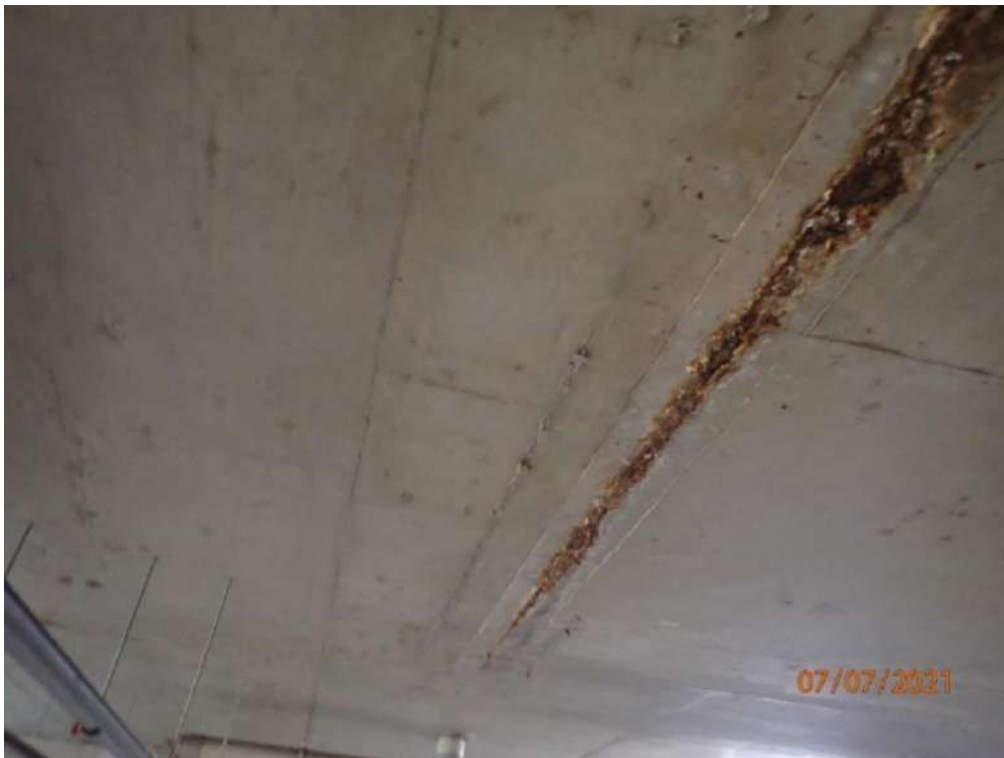
Photograph 82 – Calcification and water staining directly below the stairwell in the basement carpark
