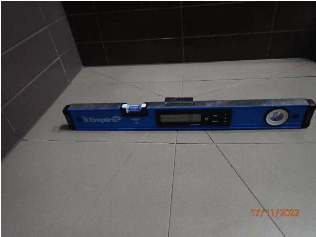
Photograph 37 - Apartment 328B bathroom shower fall
