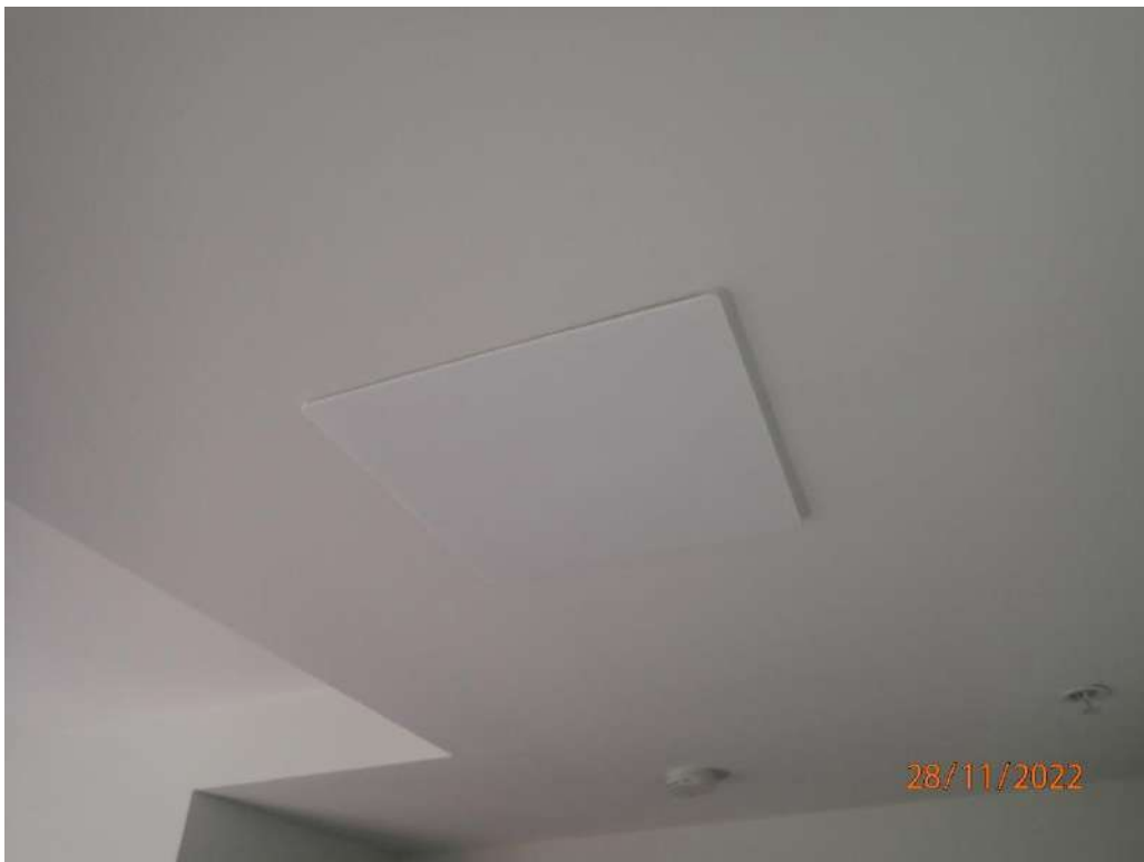
Photograph 66 - Apartment 614B living area ceiling
