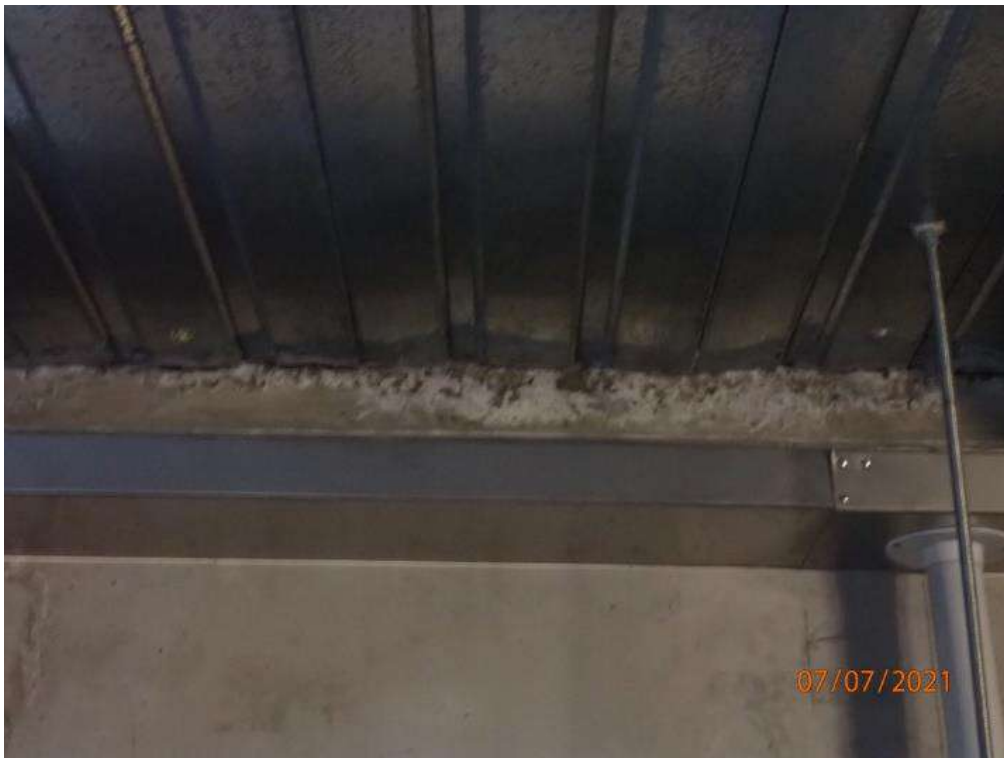
Photograph 46 - Efflorescence and calcium build up
