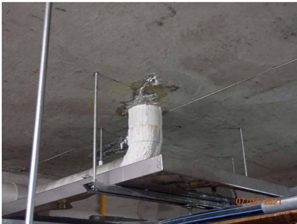
Photograph 56 - Drip tray installed below pipe penetration showing efflorescence and severe calcium build up
