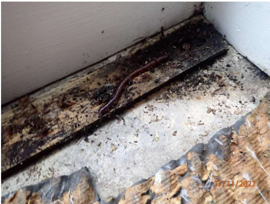
Photograph 54 - Apartment 417B bedroom 2 moisture damage to skirting trim and carpet
