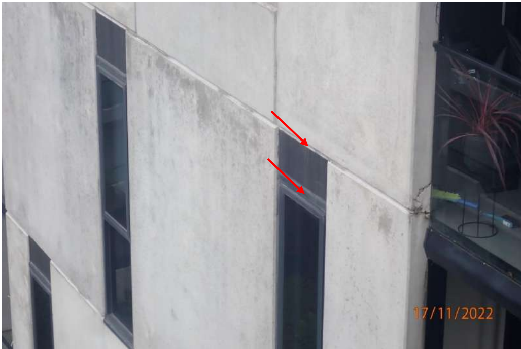
Photograph 133 - Apartment 607B, bedroom window, external view, likely entry points of water ingress
