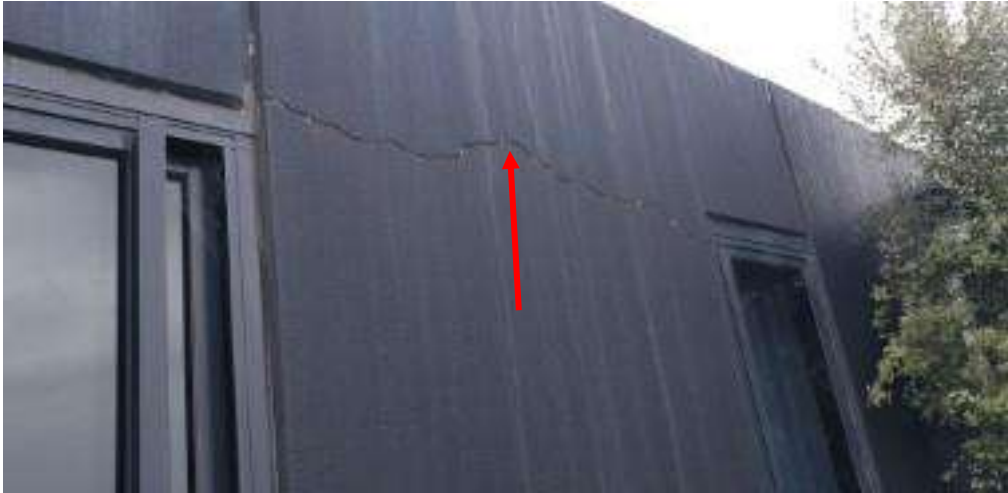
Photograph 219 - Lot 713B/Apartment 712B south wall cracking visible from main balcony(photo taken on Samsung mobile phone on 25 July 2022 by Peter Kyriakou)
