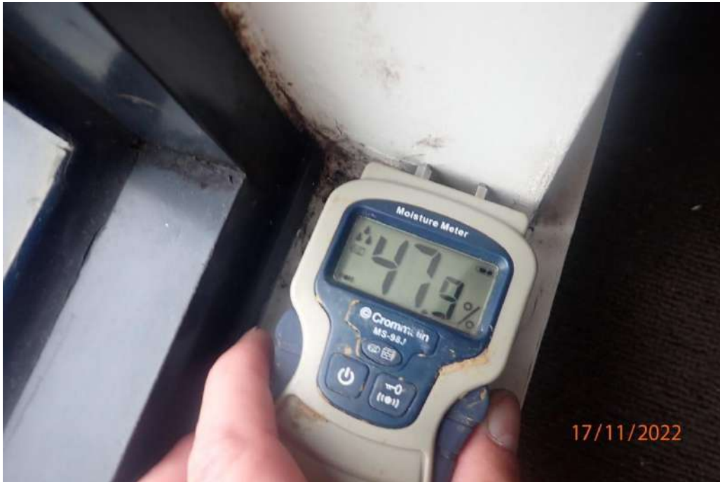
Photograph 131 - Apartment 602B, bedroom window, elevated moisture levels to wall plaster
