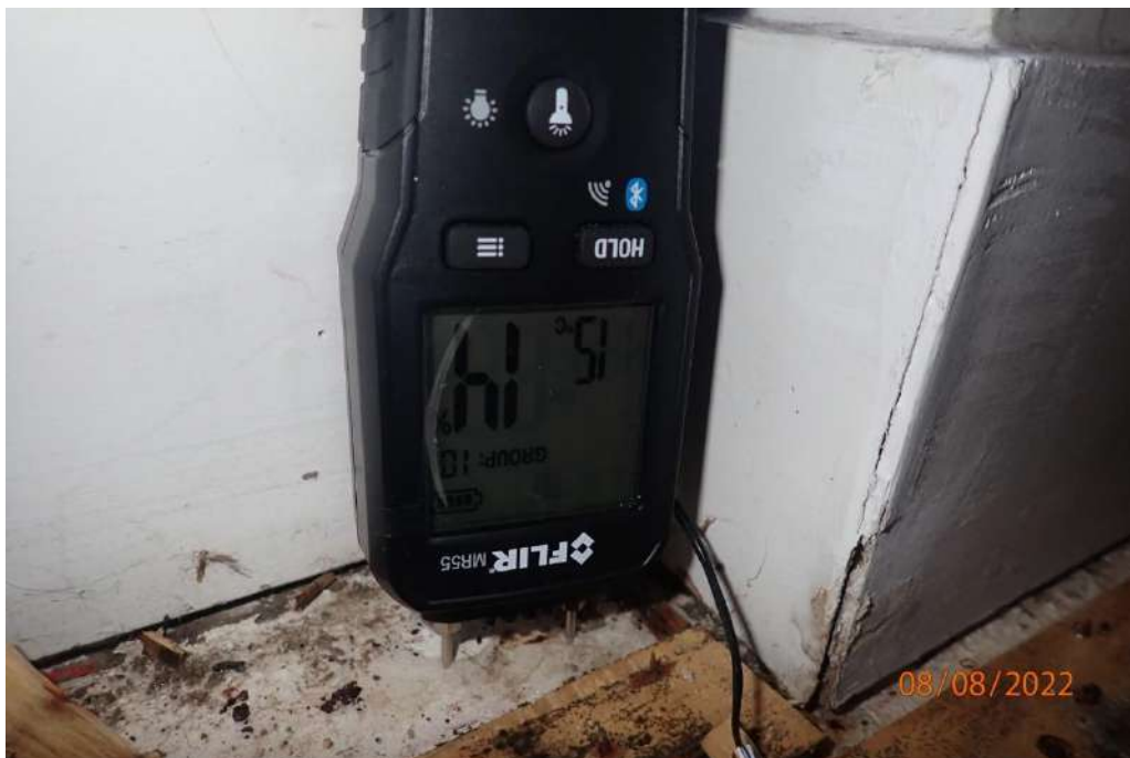
Photograph 204 - 704B/Apartment 703B, west window of the south bedroom, elevated moisture reading of 14% to concrete floor
