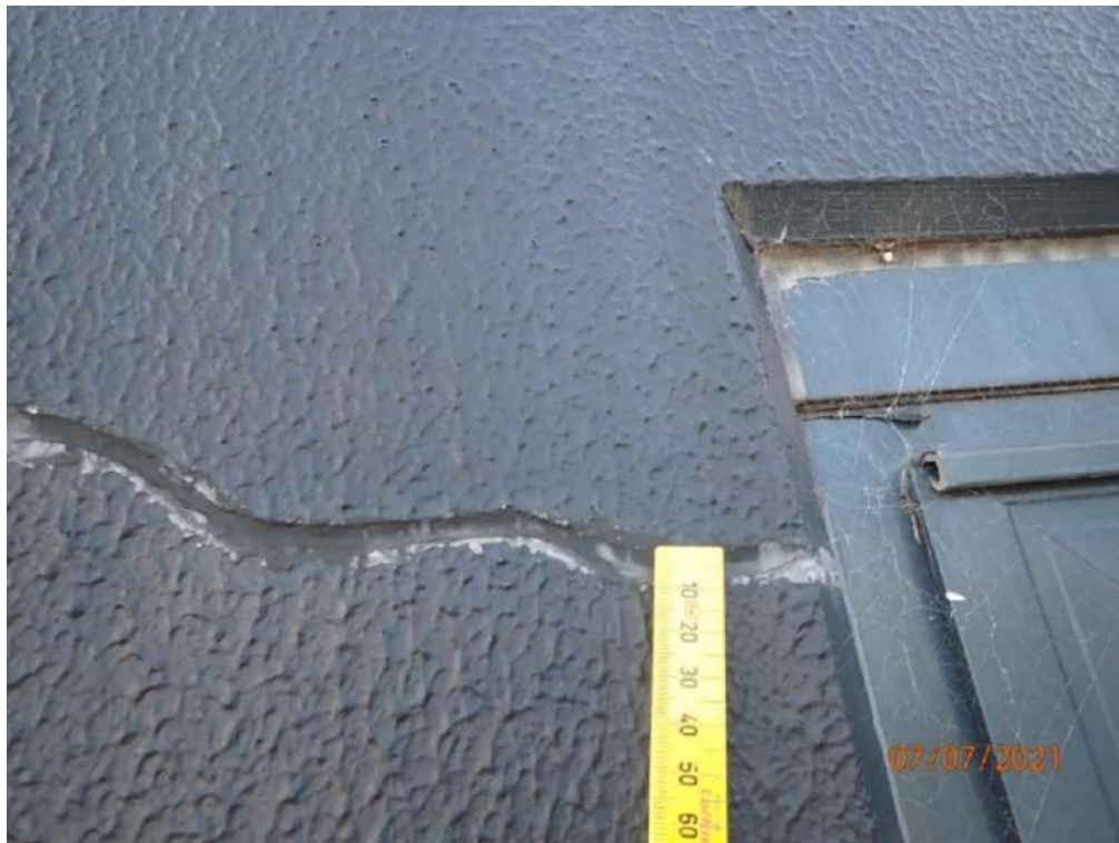
Photograph 94 – Cracking up to 10 mm wide to west elevation of building B
