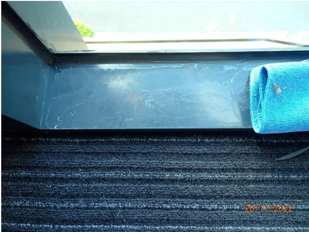
Photograph 83 - Level 4 south passageway aluminium windows, water stains
