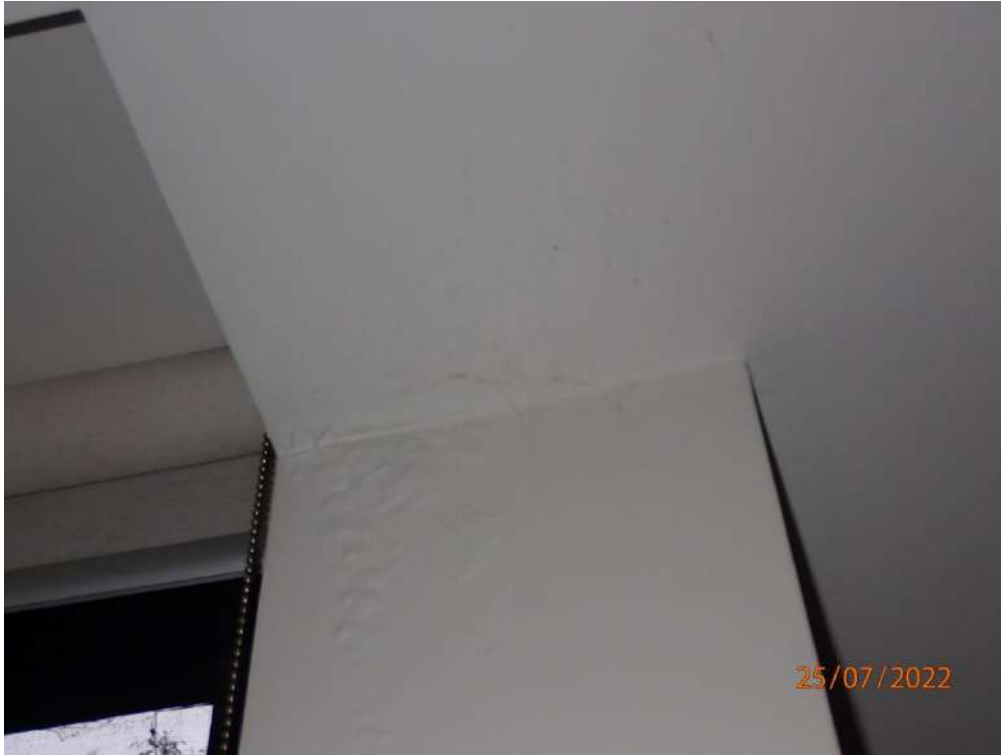
Photograph 157 - Lot 208A/Apartment 208A, bedroom window, moisture damage to wall and ceiling
