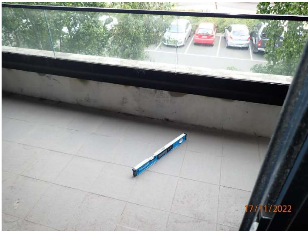
Photograph 12 - Apartment 308A balcony fall
