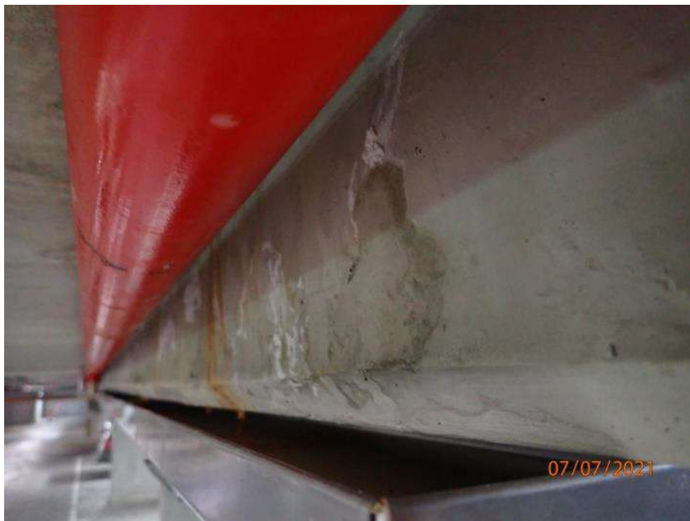
Photograph 48 - Efflorescence and calcium build up
