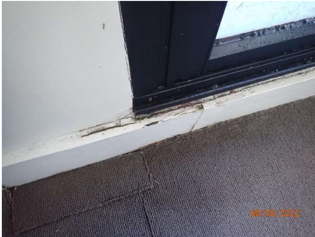
Photograph 211 - 704B/Apartment 703B, living sliding door opening to balcony, damaged skirting trim and carpet
