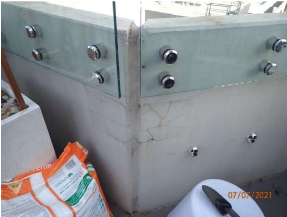
Photograph 114 – Fill is cracking away at tension plates
