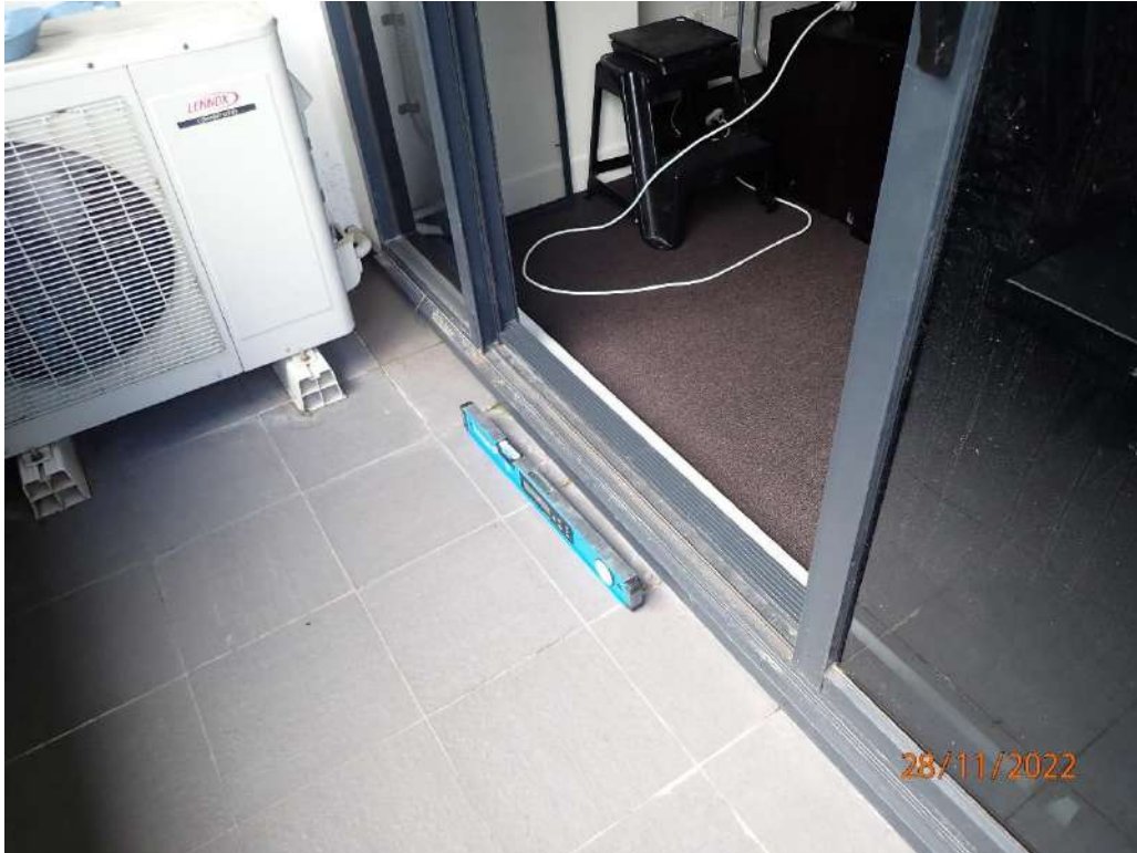
Photograph 91 - Apartment 431B balcony fall
