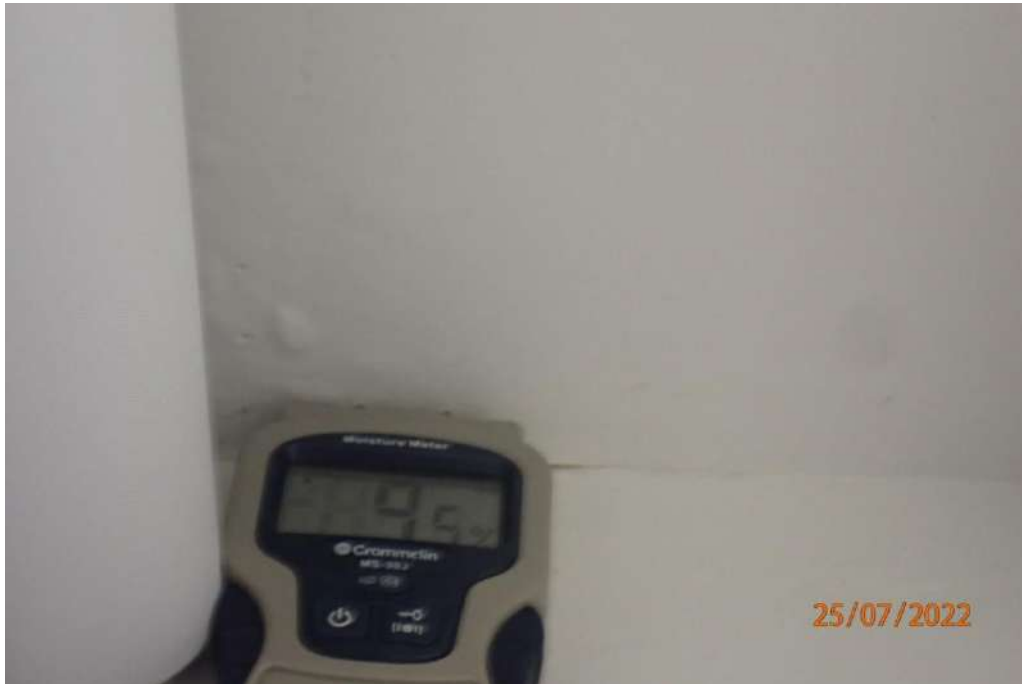
Photograph 163 – Lot 221B/Apartment 231B, northern bedroom, west window reveal moisture reading 9.5%
