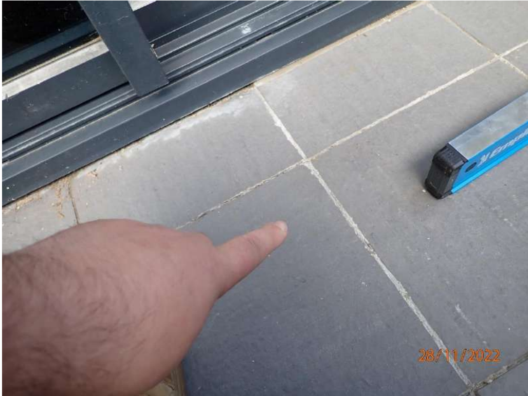
Photograph 97 - Apartment 431B balcony, efflorescence between grout lines
