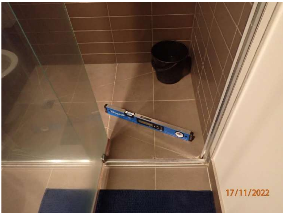
Photograph 2 – Apartment 309A bathroom shower
