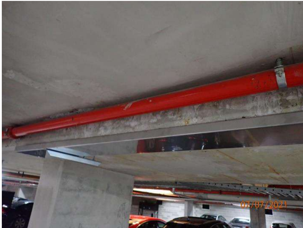
Photograph 47 - Efflorescence and calcium build up
