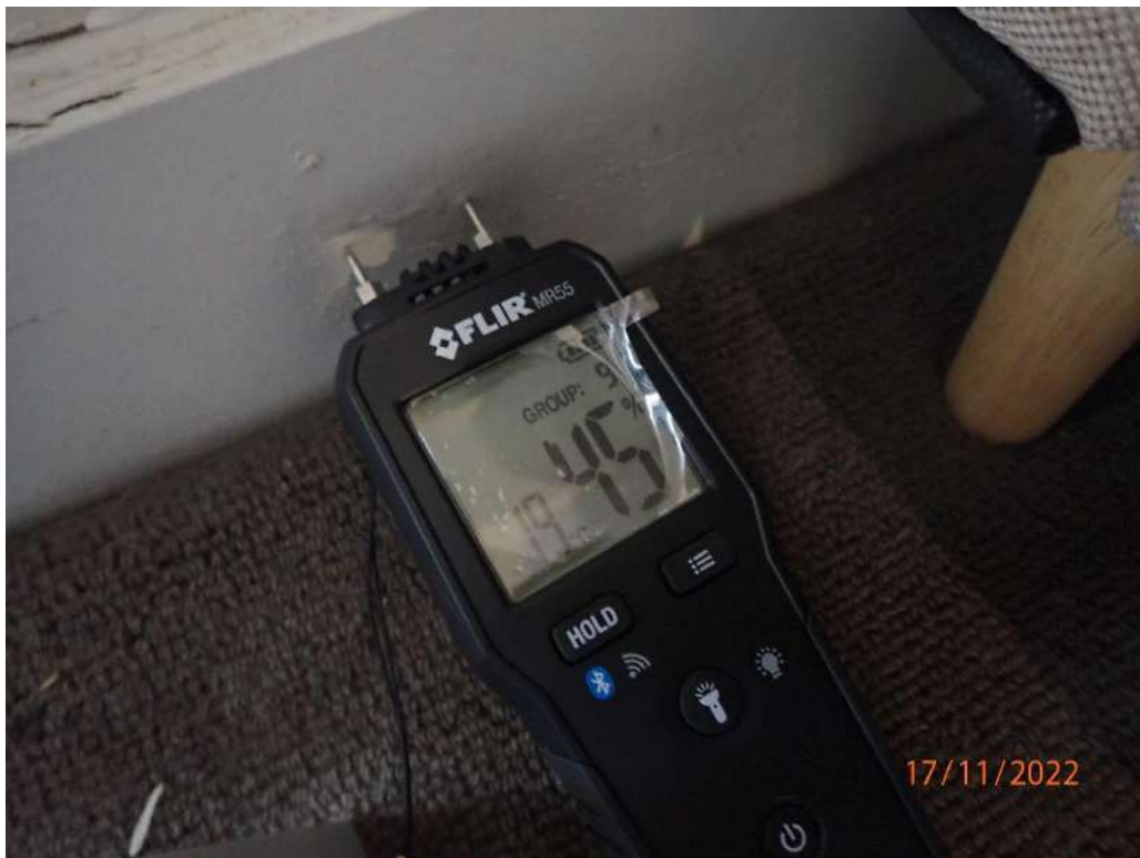
Photograph 58 - Apartment 417B bedroom 2, high moisture levels in skirting trim
