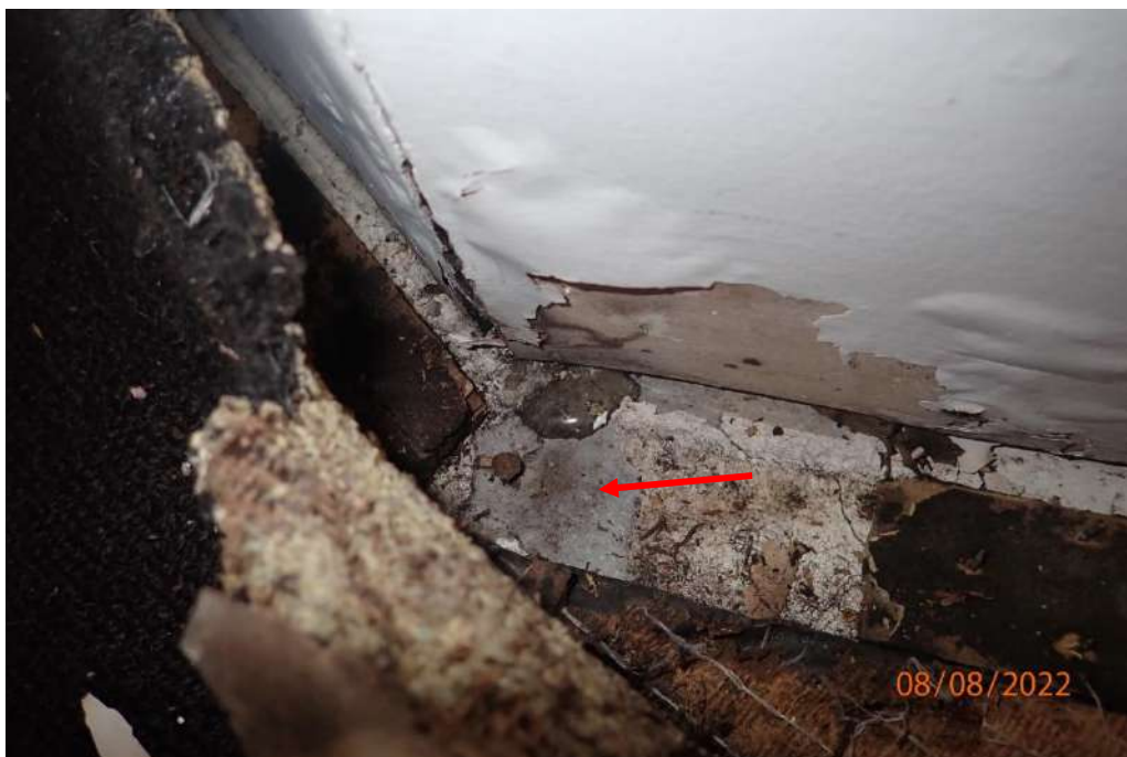
Photograph 190 - Lot 402A/Apartment 402A water ingress to west living area floor
