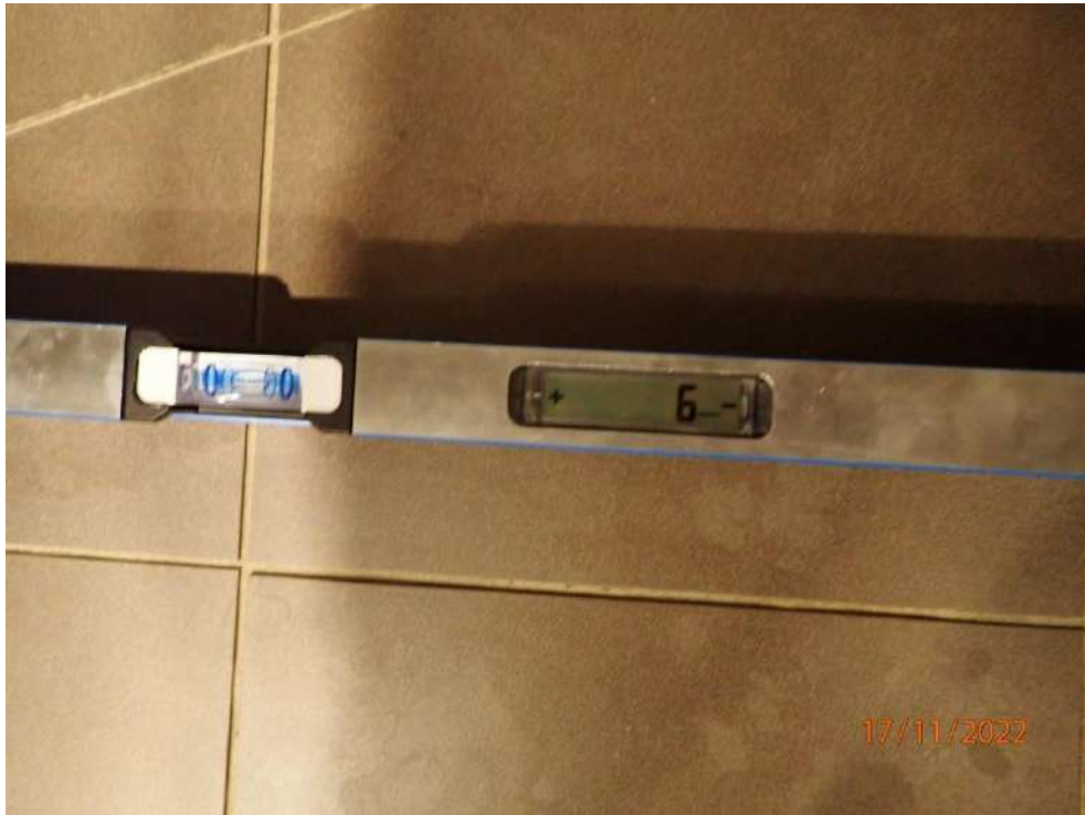
Photograph 5 - Apartment 309A bathroom shower fall 1 in 167
