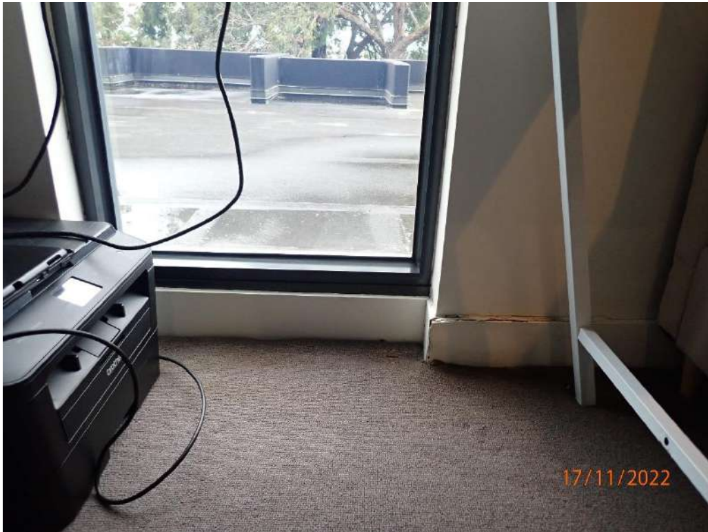
Photograph 51 - Apartment 417B bedroom 2 west facing window
