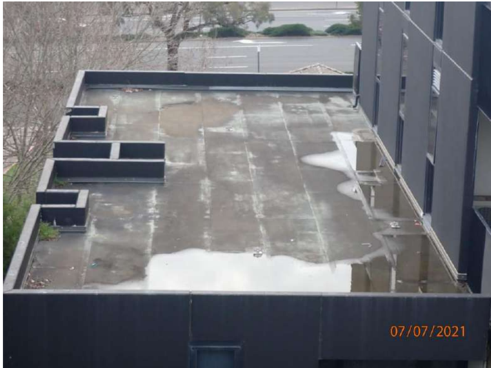
Photograph 125 – Water ponding west elevation of building B
