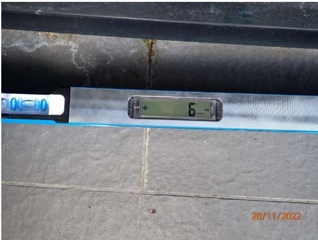
Photograph 92 - Apartment 431B balcony fall 1 in 167
