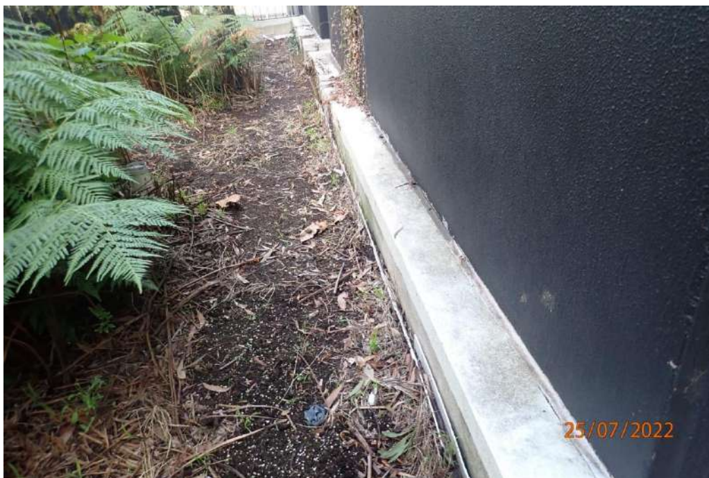
Photograph 146 - Lot 106B/Apartment 116B, west elevation wall and planter box
