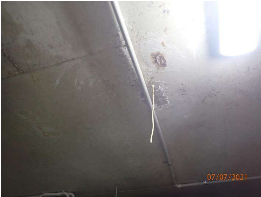
Photograph 50 - Efflorescence, severe calcium build up
