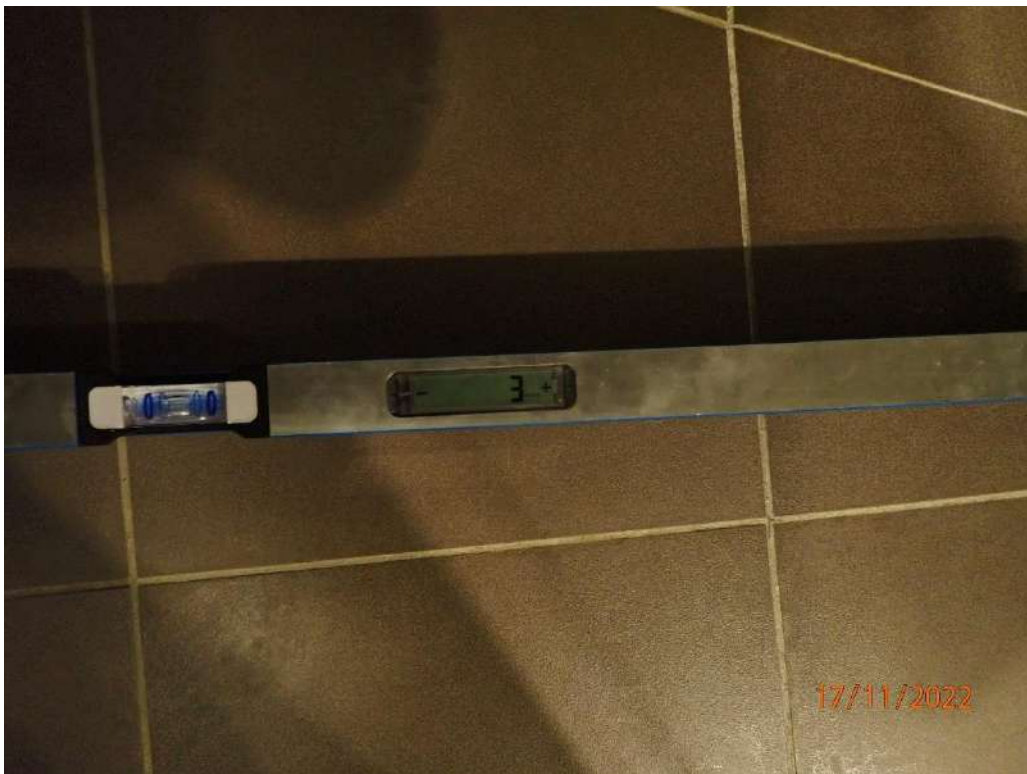
Photograph 28 - Apartment 526B bathroom shower fall 1 in 333
