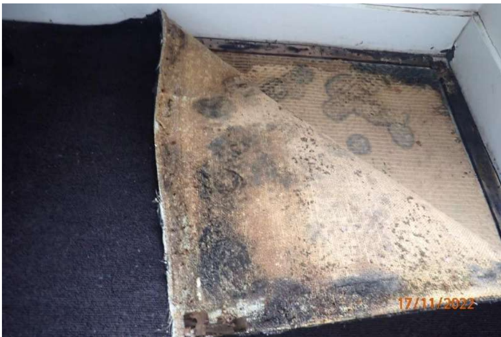
Photograph 116 - Apartment 126B, southeast corner of bedroom 2, water damage and mould growth to carpet and underlay
