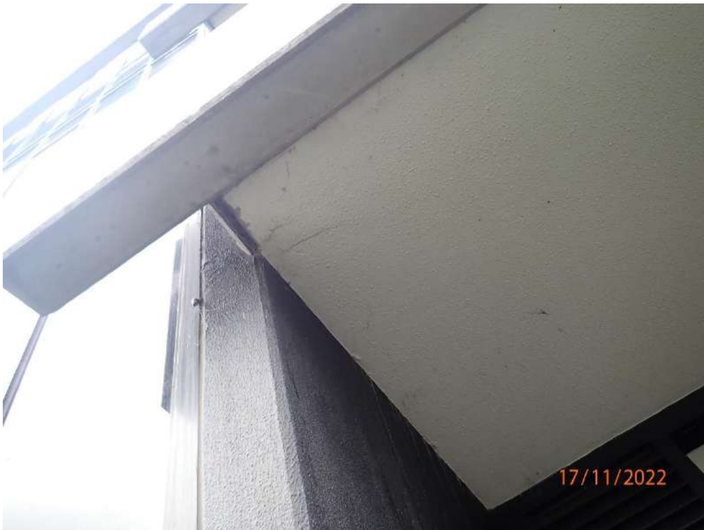
Photograph 24 - Apartment 308A balcony west wall
