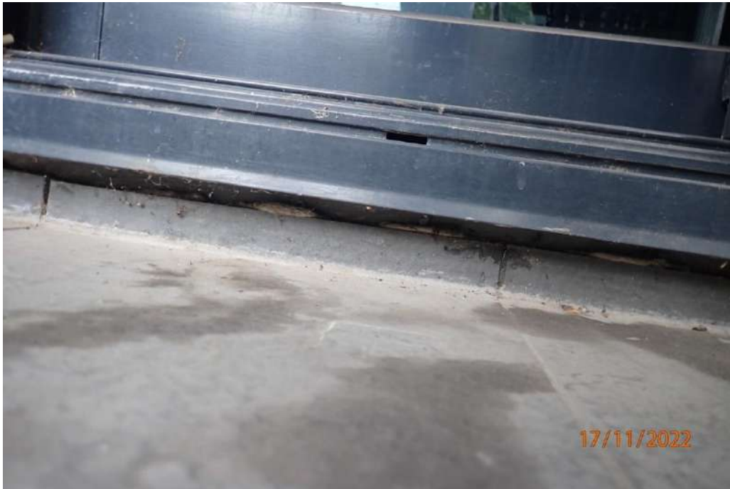
Photograph 107 - Apartment 205A balcony upturn beneath aluminium sliding door and window unit
