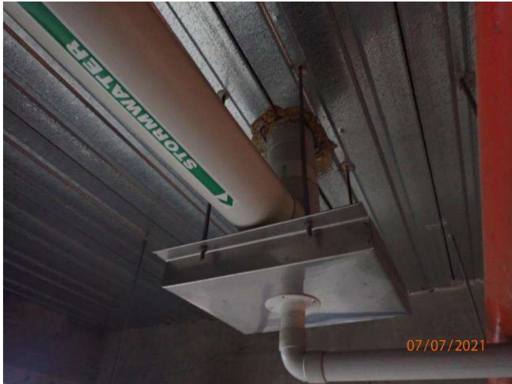
Photograph 43 – Drip tray installed below pipe penetration
