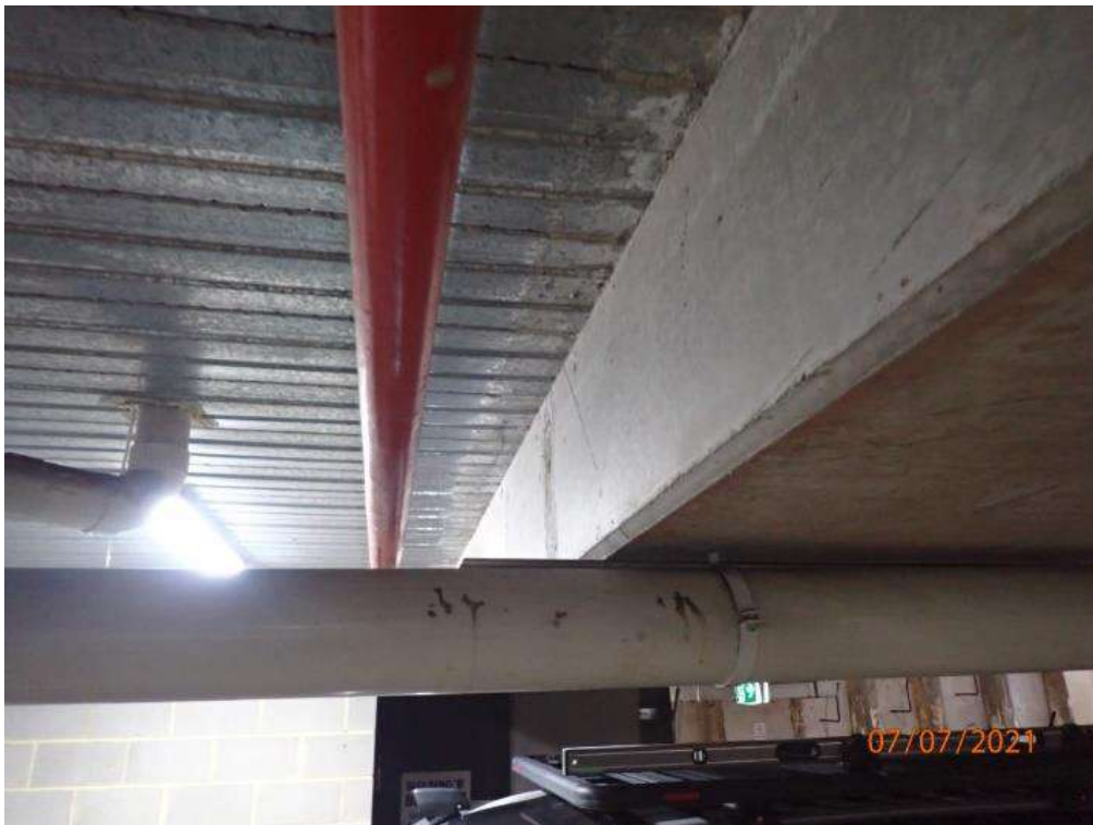
Photograph 64 - Efflorescence and calcium build up to the east end of basement carpark
