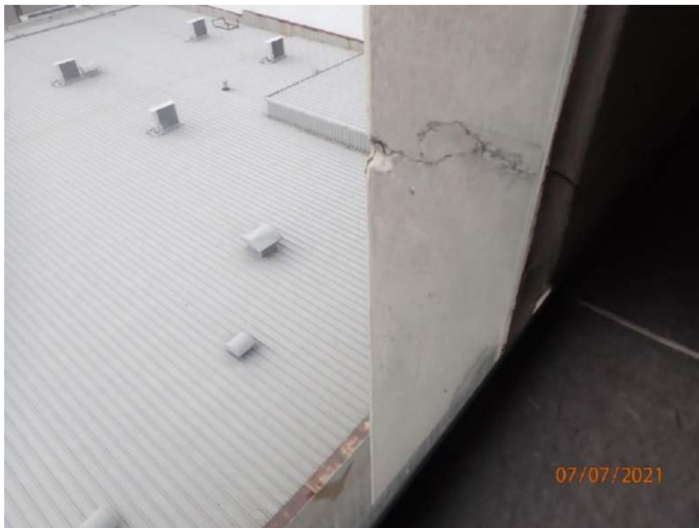
Photograph 100 – Cracking to south elevation of building B
