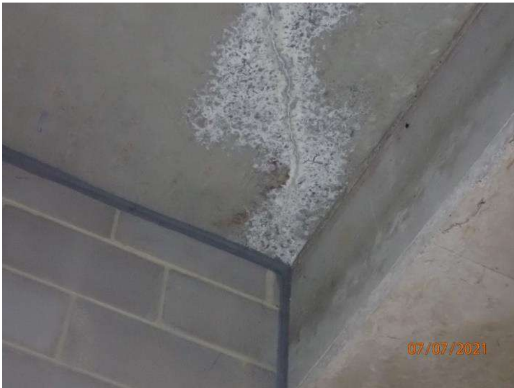
Photograph 12 - Efflorescence and concrete cracked to south elevation above visitor carpark 6
