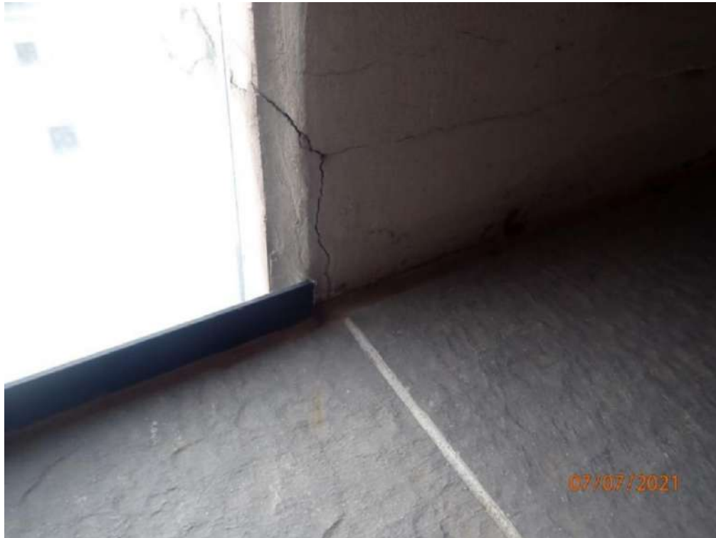
Photograph 99 – Cracking to south elevation of building B
