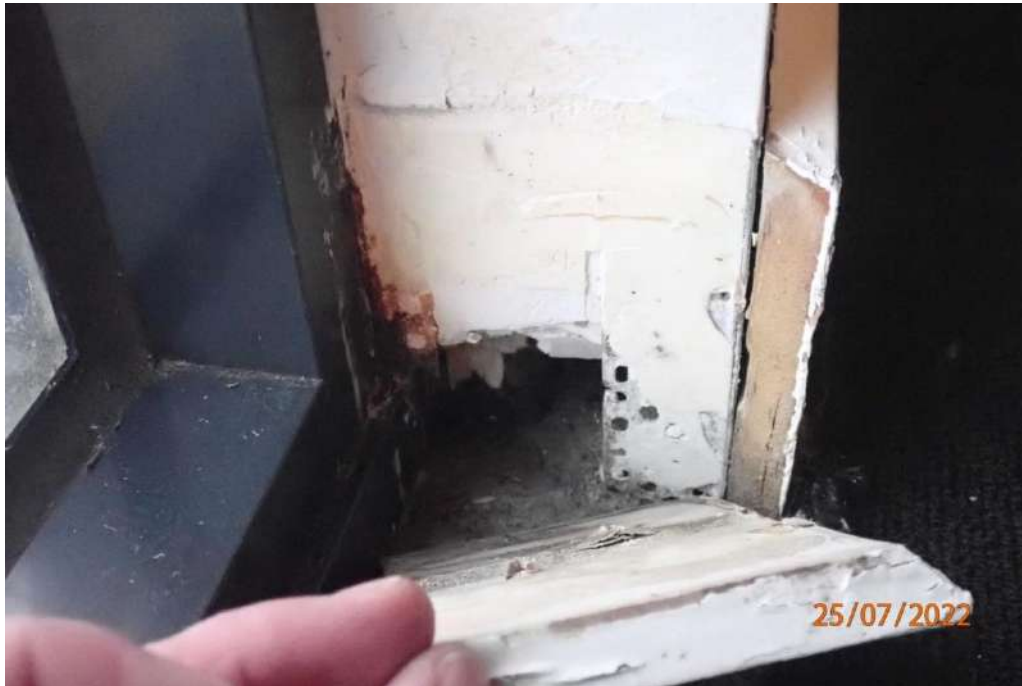
Photograph 175 - Lot 321B/Apartment 333B, damaged skirting trim adjacent to the window on the south wall of the living area
