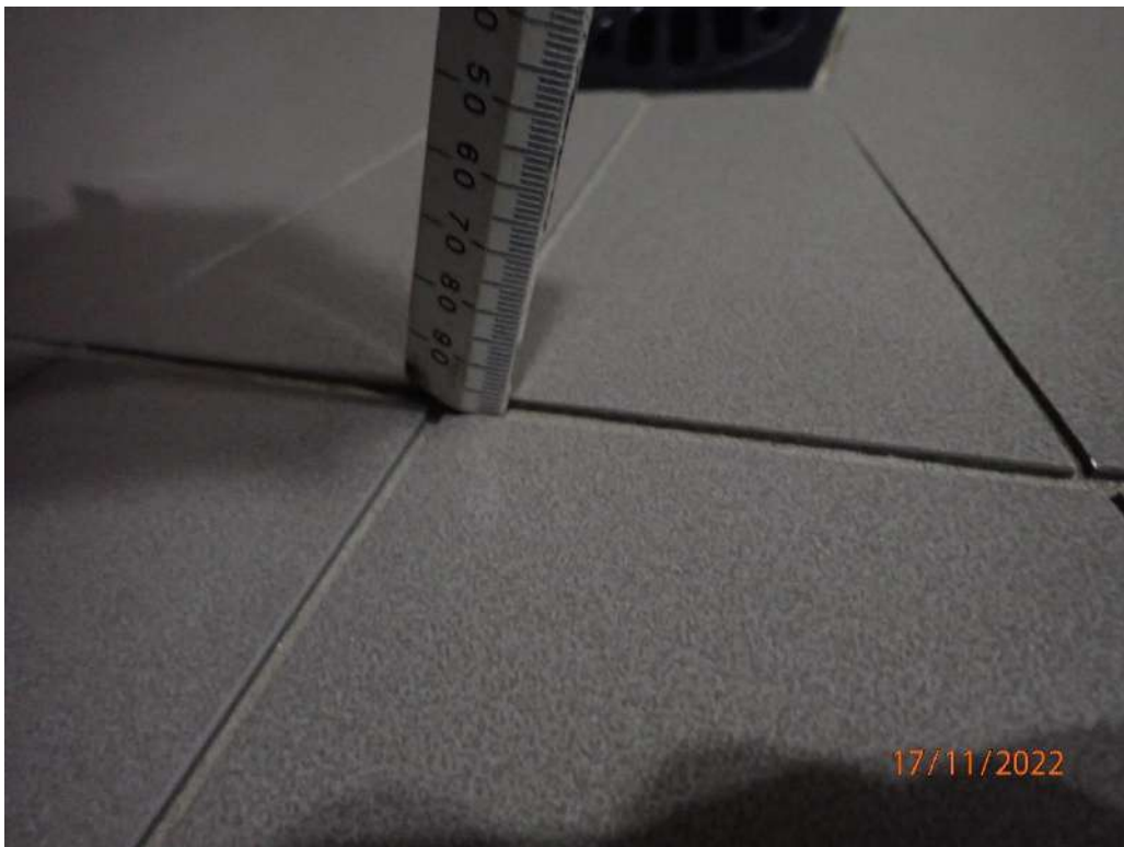
Photograph 40 - Apartment 328B bathroom shower recessed grout lines
