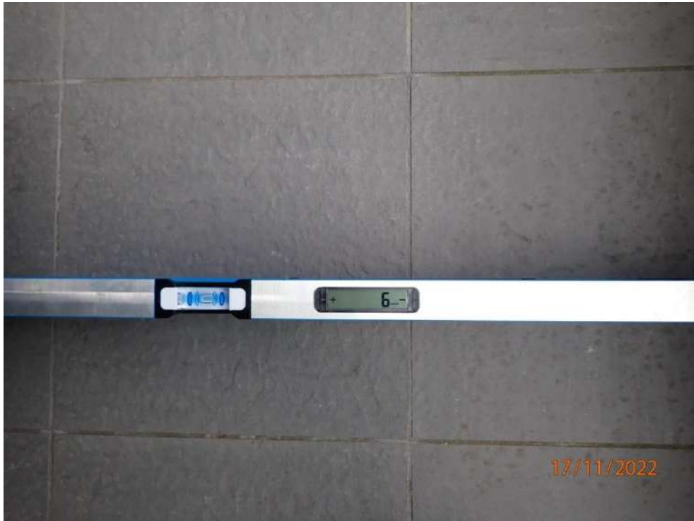
Photograph 15 - Apartment 308A balcony fall 1 in 167
