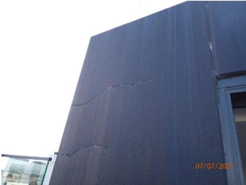
Photograph 93 – Cracking to west elevation of building B
