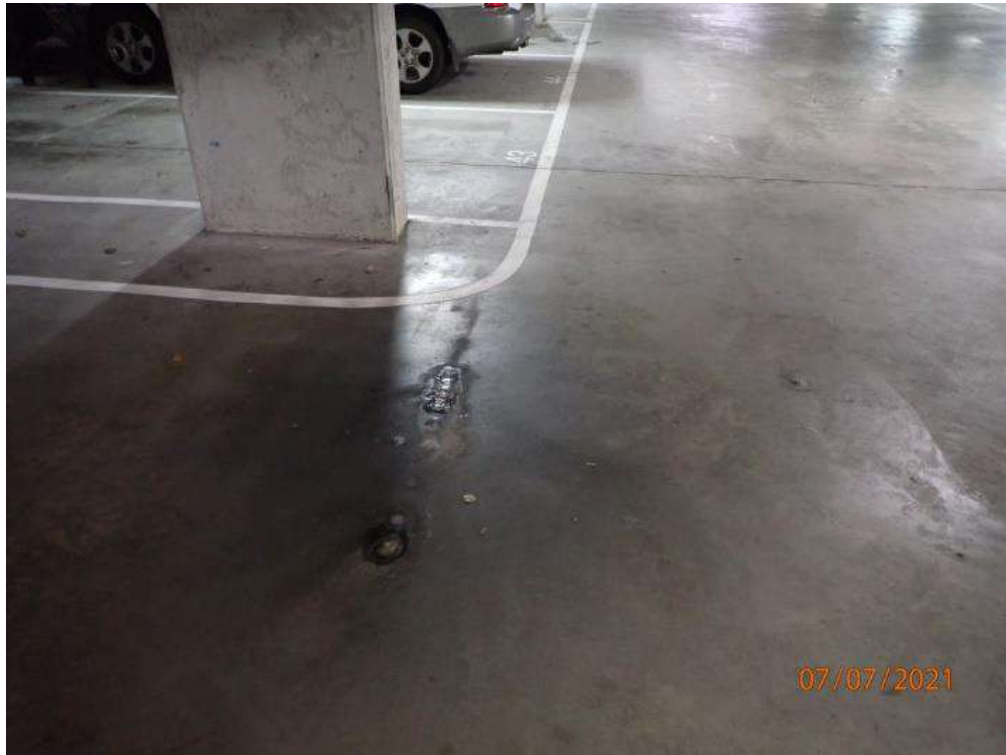
Photograph 59 - Calcium build up to concrete basement floor
