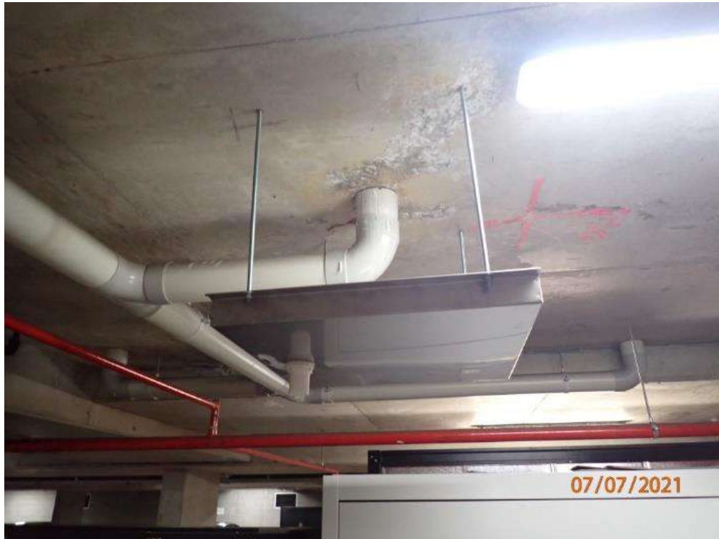
Photograph 39 – Drip tray installed below pipe penetration
