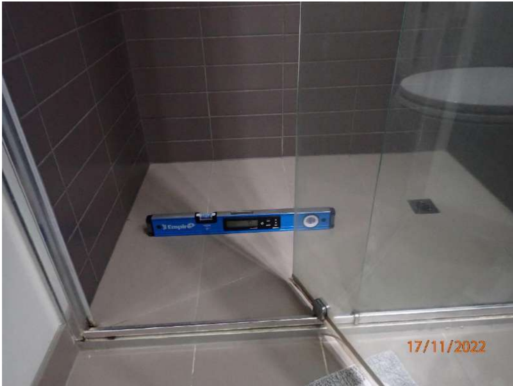
Photograph 33 - Apartment 328B bathroom shower fall
