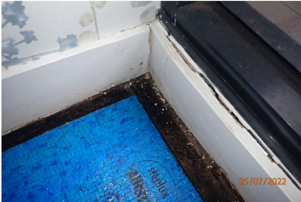
Photograph 181 - Lot 324B/Apartment 336B, north west corner of living area, carpet smooth edge rot and mould; and skirting trim delamination
