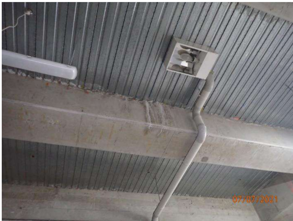
Photograph 66 - Efflorescence and calcium build up to the east end of basement carpark
