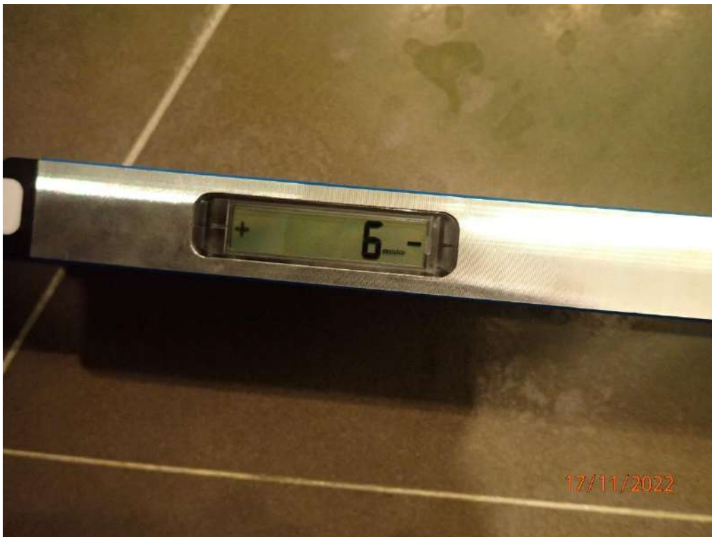
Photograph 30 - Apartment 526B bathroom shower fall 1 in 167
