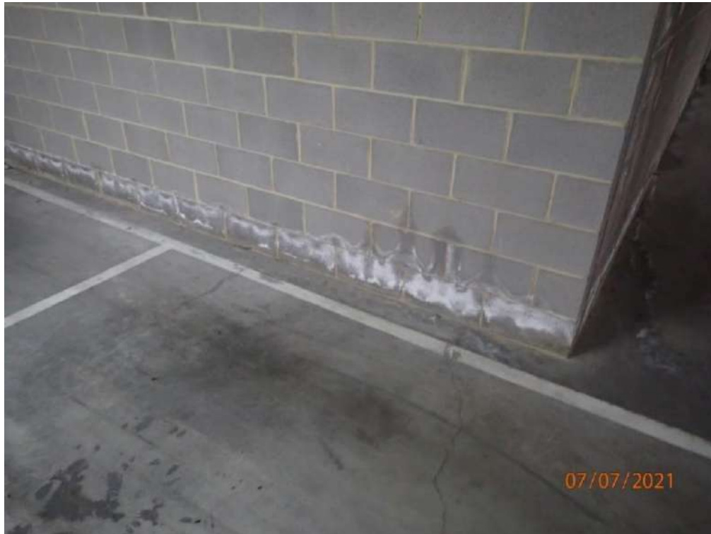
Photograph 85 – Efflorescence to the block walls adjacent the water tanks
