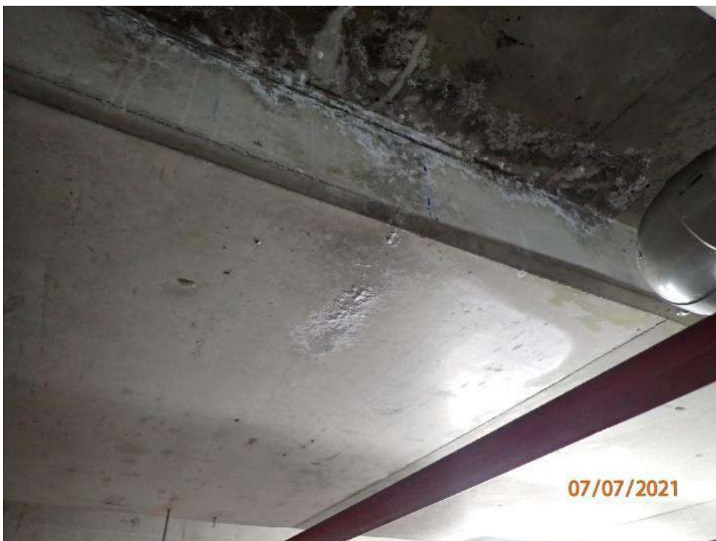
Photograph 42 – Efflorescence and calcium build up
