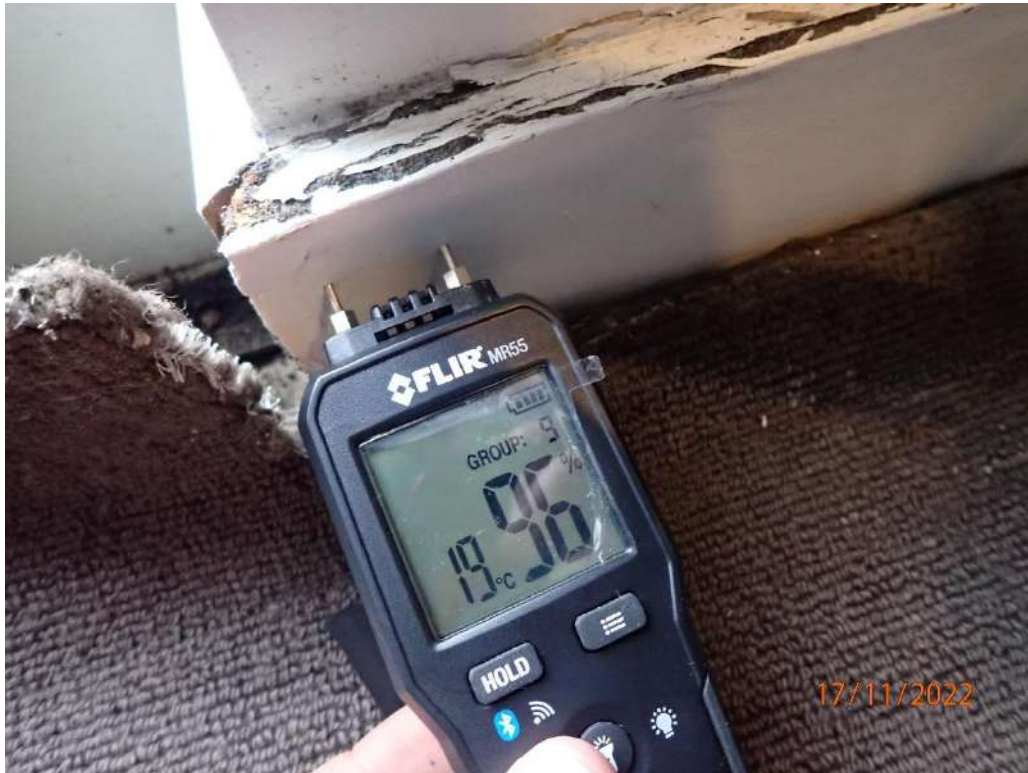
Photograph 57 - Apartment 417B bedroom 2, high moisture levels in skirting trim
