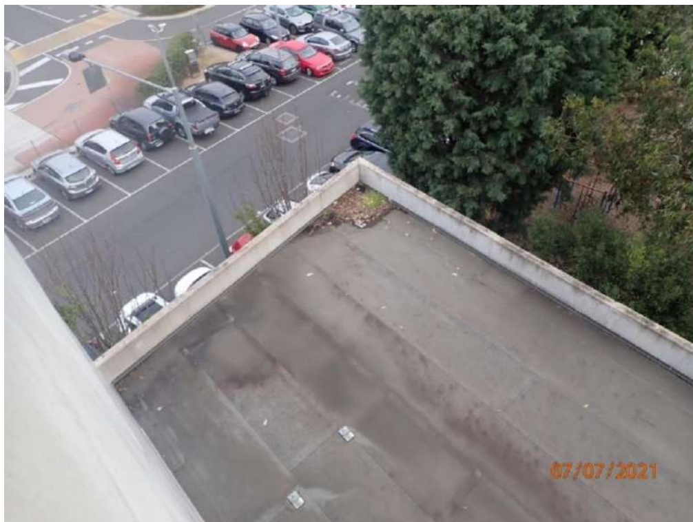
Photograph 126 – Water staining and leaves gathering at external edges of roof to west elevation of building A
