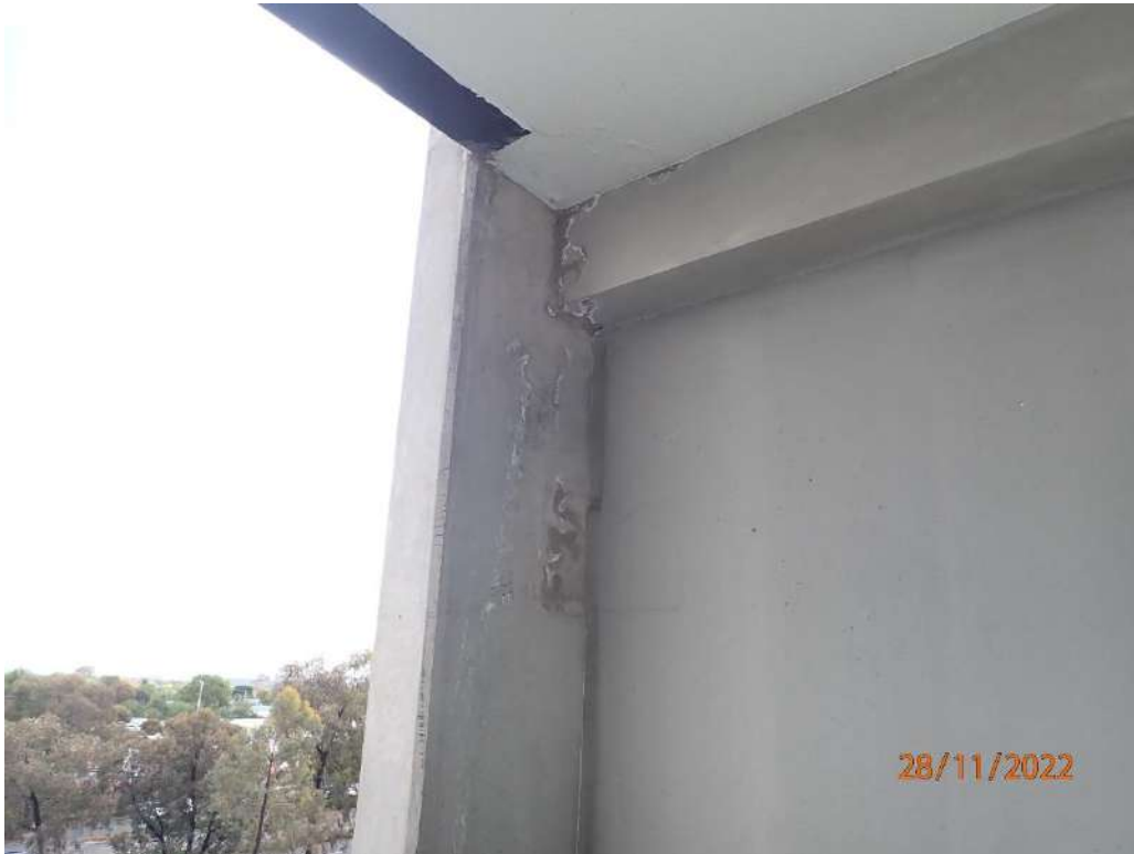
Photograph 75 – Apartment 518B, northeast balcony wall
