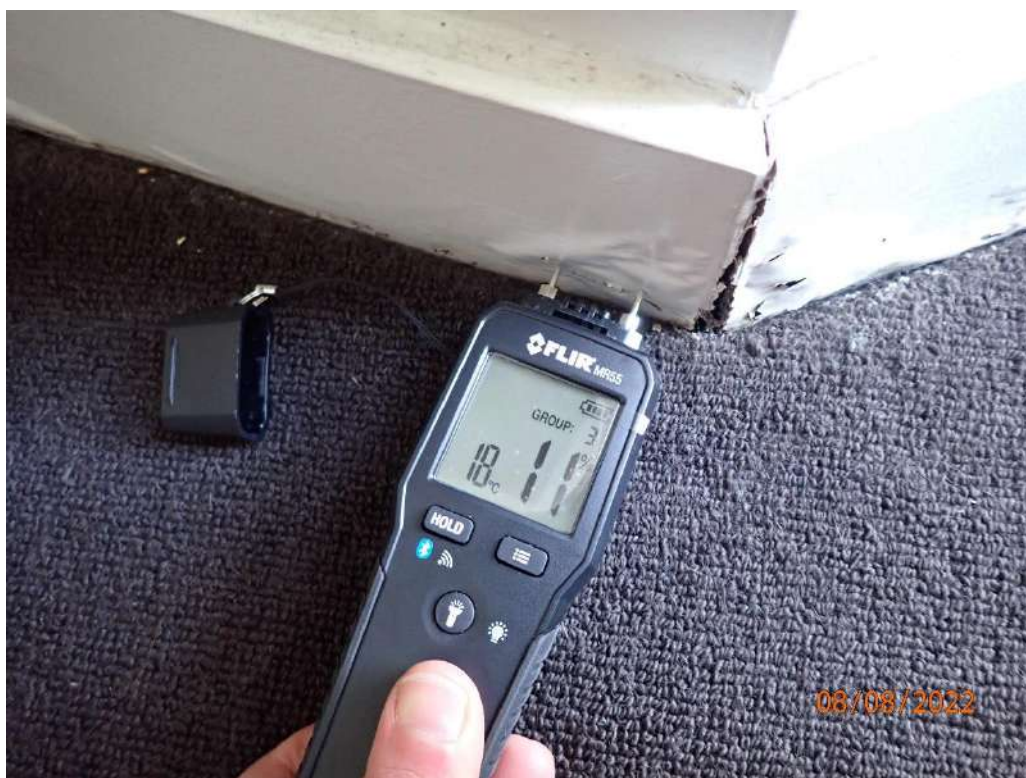
Photograph 186 - Lot 402A/Apartment 402A living area west wall skirting trim moisture reading
