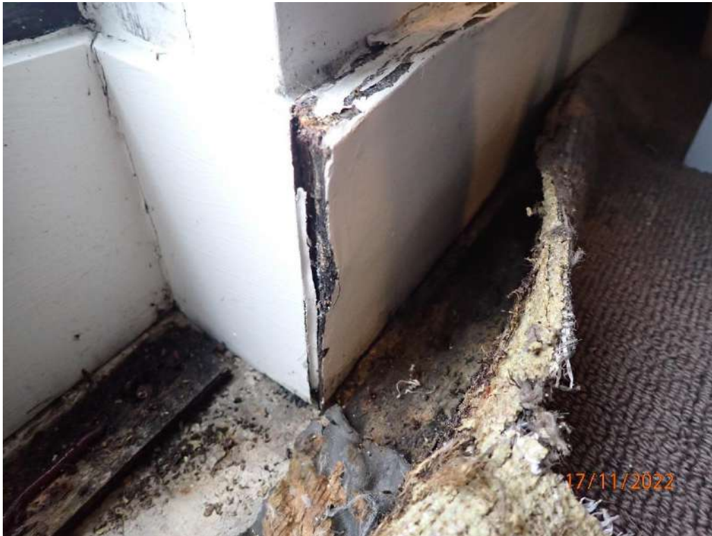
Photograph 55 - Apartment 417B bedroom 2 moisture damage to skirting trim and carpet
