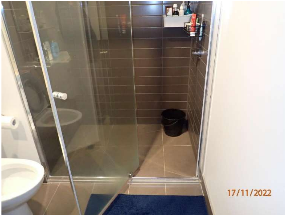
Photograph 1 – Apartment 309A bathroom shower
