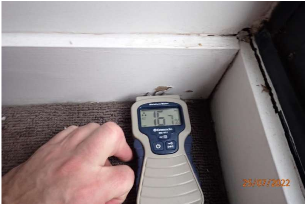
Photograph 197 - Lot 607B/Apartment 605B, south end of west wall opening to the balcony, elevated moisture reading 16.7%
