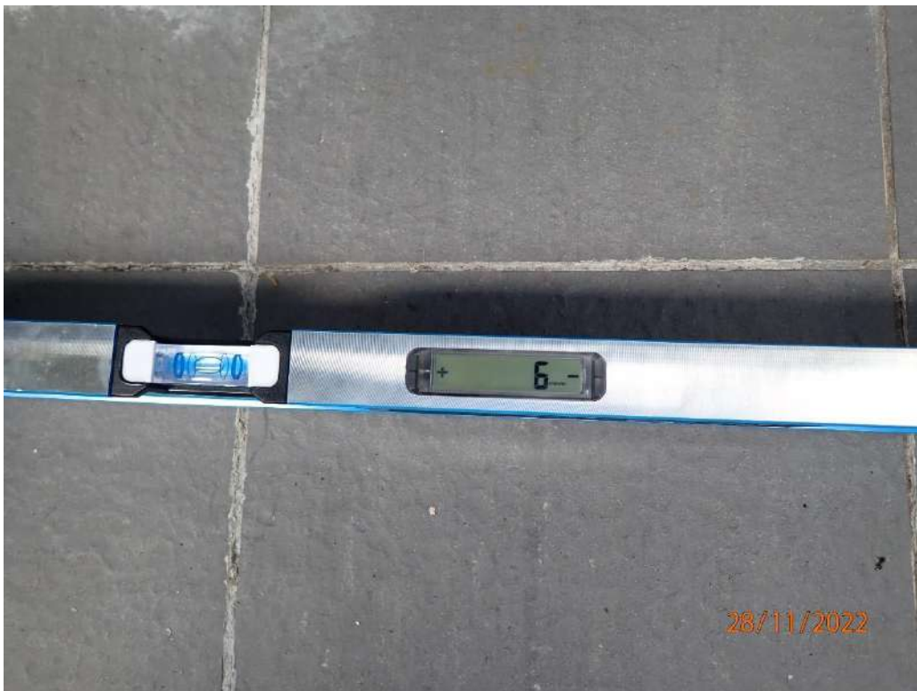
Photograph 94 - Apartment 431B balcony fall 1 in 167
