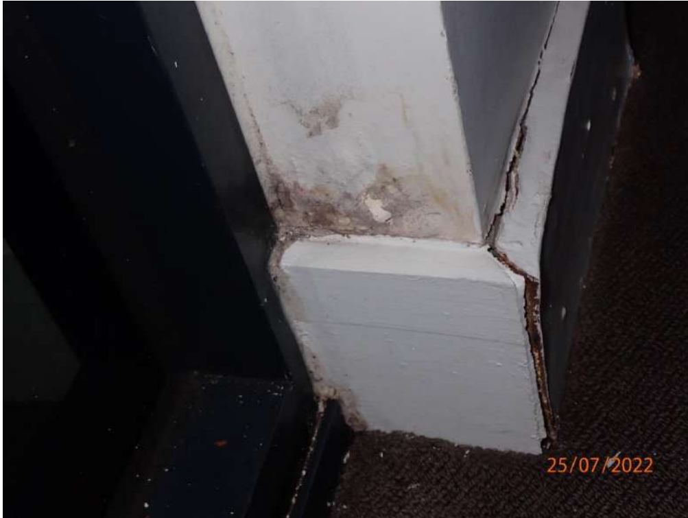
Photograph 159 - Lot 208A/Apartment 208A, bedroom window, moisture damage to skirting trim and window reveal
