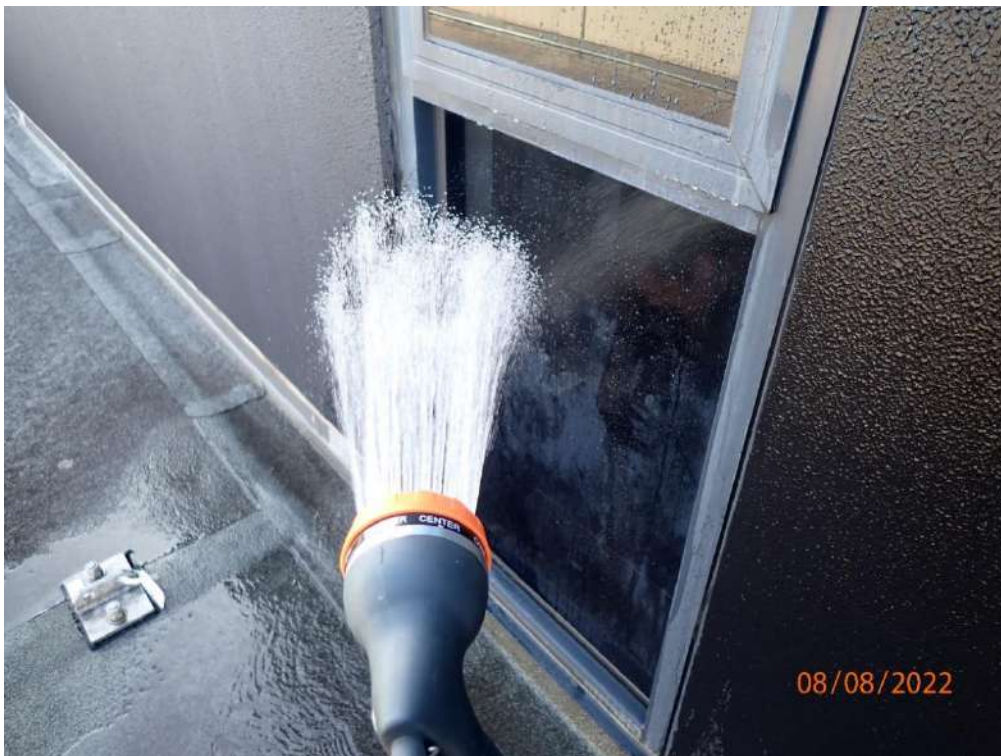
Photograph 208 - 704B/Apartment 703B, water testing external west window of the south bedroom
