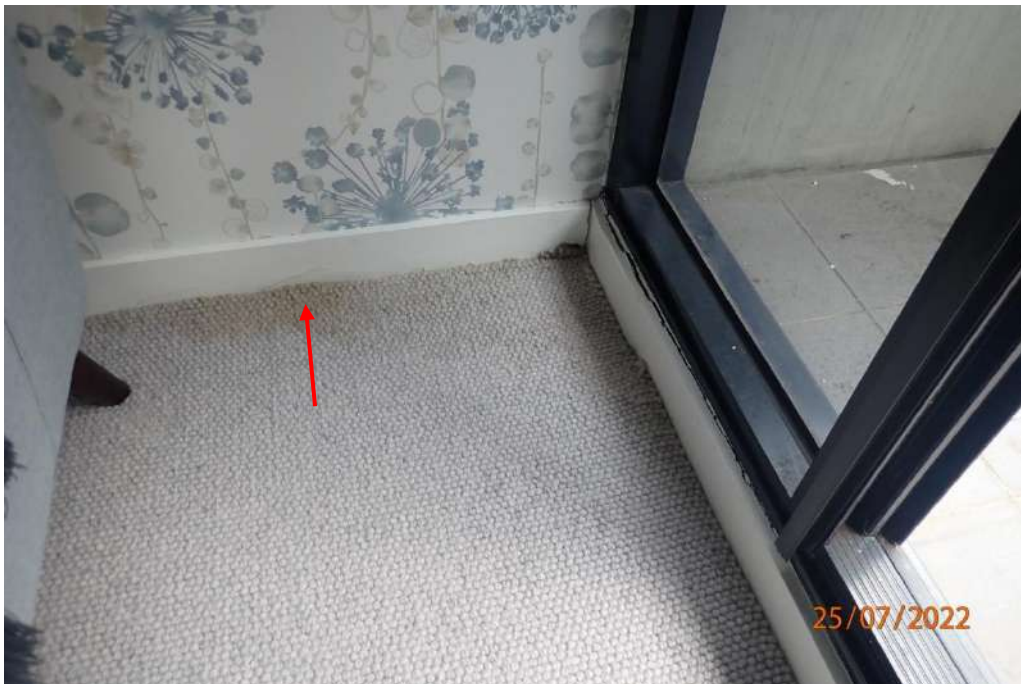
Photograph 178 – Lot 324B/Apartment 336B, north west corner of living area, carpet staining
