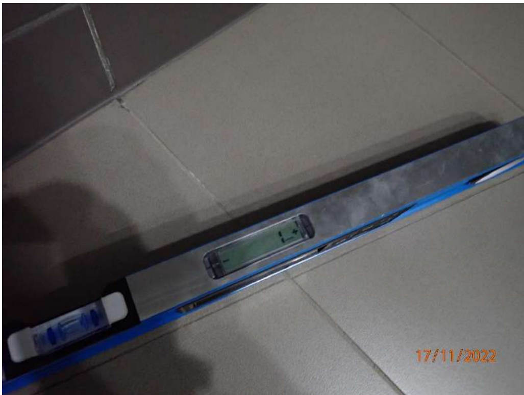
Photograph 36 - Apartment 328B bathroom shower fall 1 in 1,000
