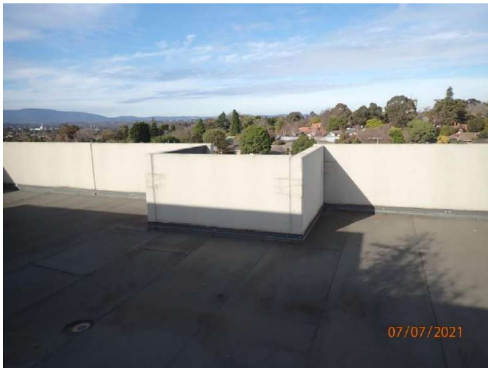
Photograph 112 – Fill is cracking away at tension plates
