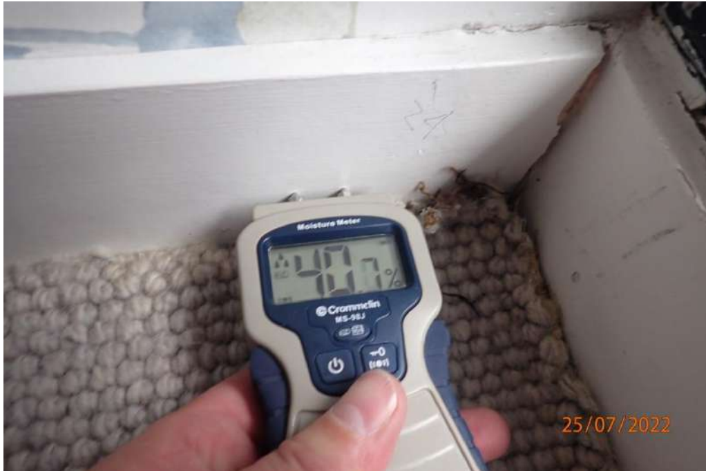
Photograph 180 - Lot 324B/Apartment 336B, north west corner of living area, skirting trim moisture reading 40.7%
