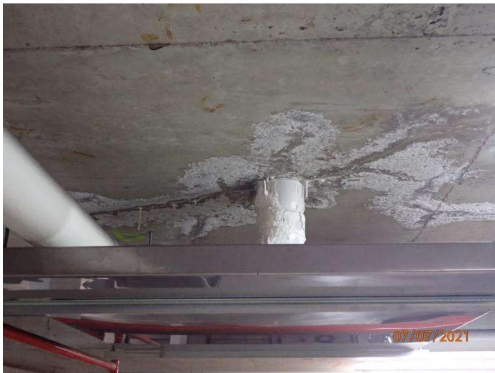
Photograph 60 – Drip tray installed below efflorescence, calcium build up and cracking to ceiling
