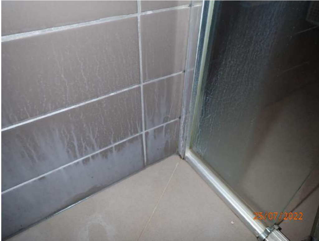
Photograph 167 - Lot 306A/Apartment 306A, adjacent to affected wall from within shower
