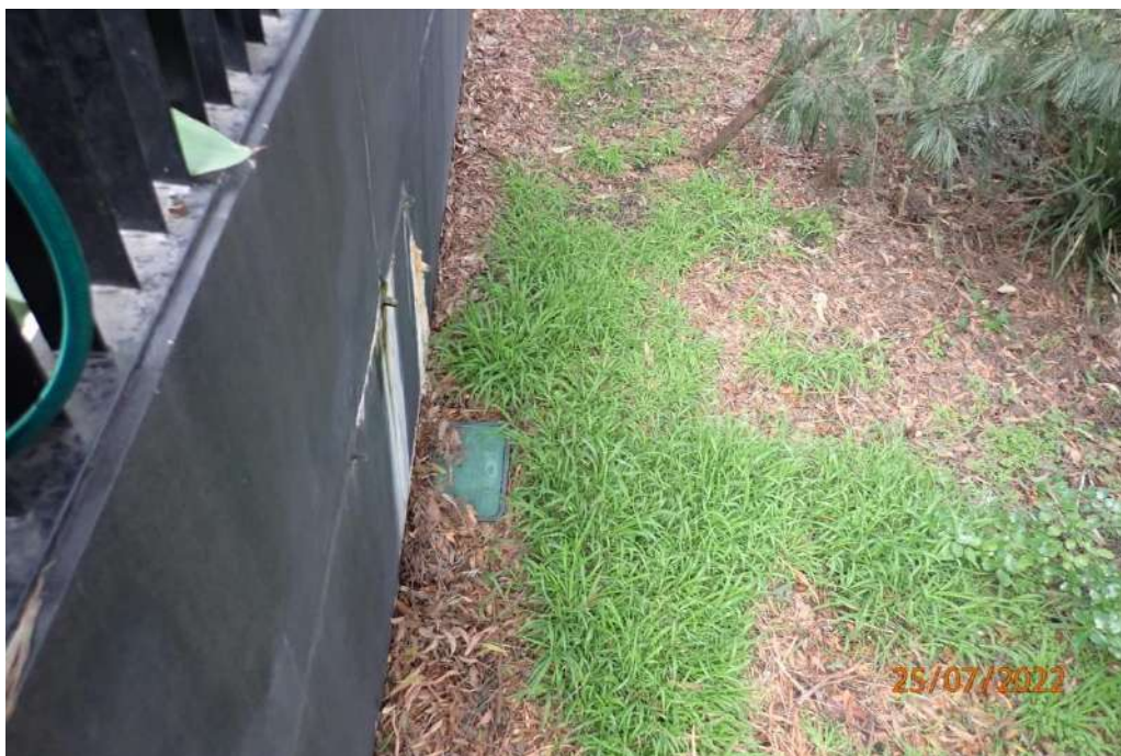
Photograph 148 - Lot 109A/Apartment 109A, planter box overflow outlet
