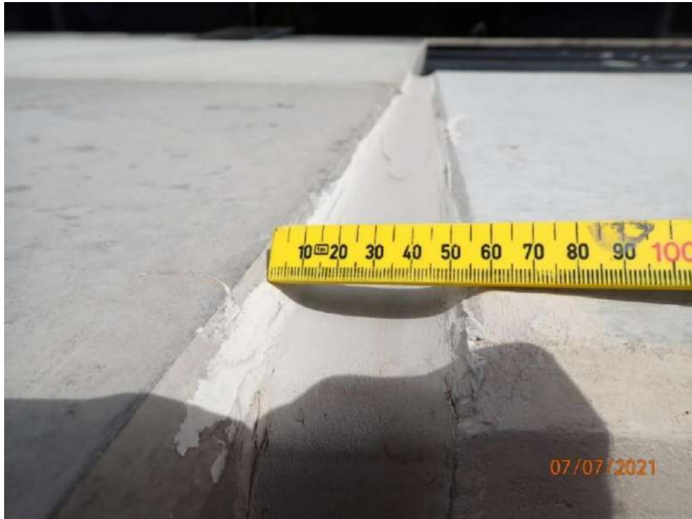
Photograph 115 – Gaps between concrete wall panels exceeding 50 mm to building B
