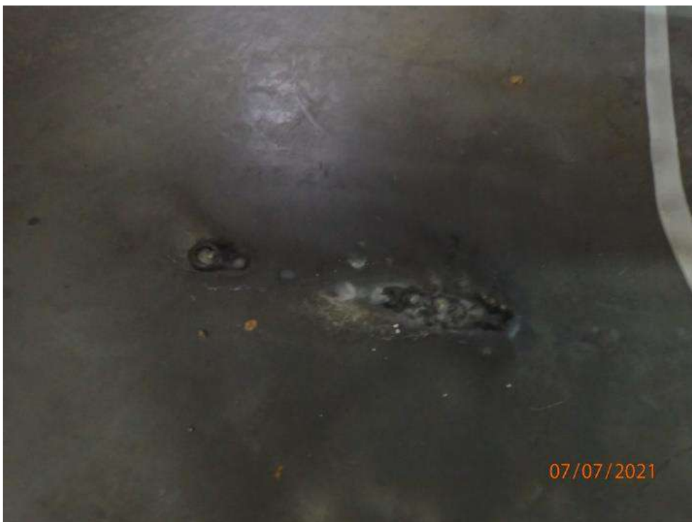
Photograph 20 - Calcium deposits to ground concrete slab below concrete beam above carpark 43
