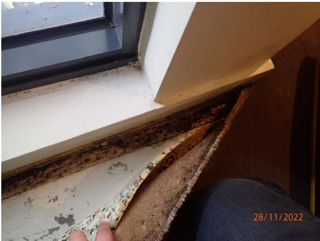
Photograph 68 - Apartment 109A bedroom 2 initial moisture damage to timber smooth edge
