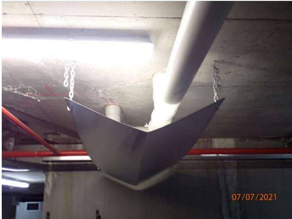
Photograph 57 – Drip tray installed below pipe penetration
