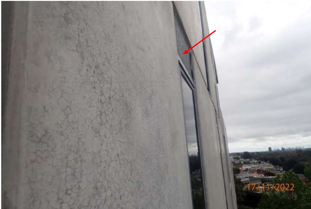
Photograph 127 - Apartment 607B, bedroom window, external view, possible entry point of water ingress
