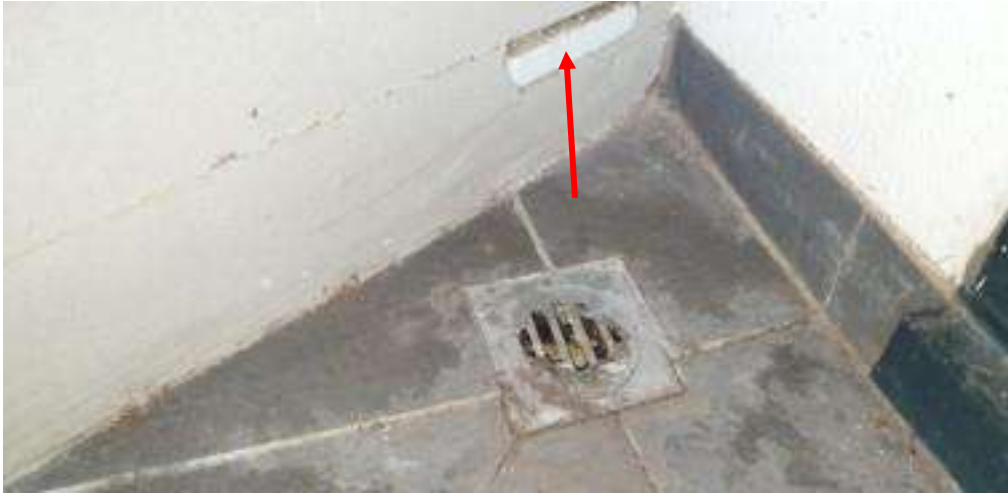
Photograph 217 - Lot 713B/Apartment 712B bedroom balcony wall missing render (photo taken on Samsung mobile phone on 25 July 2022 by Peter Kyriakou)
