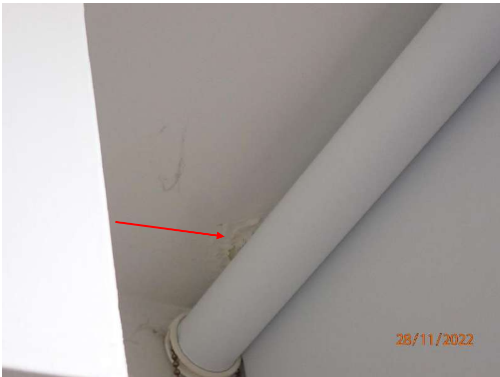
Photograph 100 - Apartment 604B, living area pelmet, water damage to plaster in view
