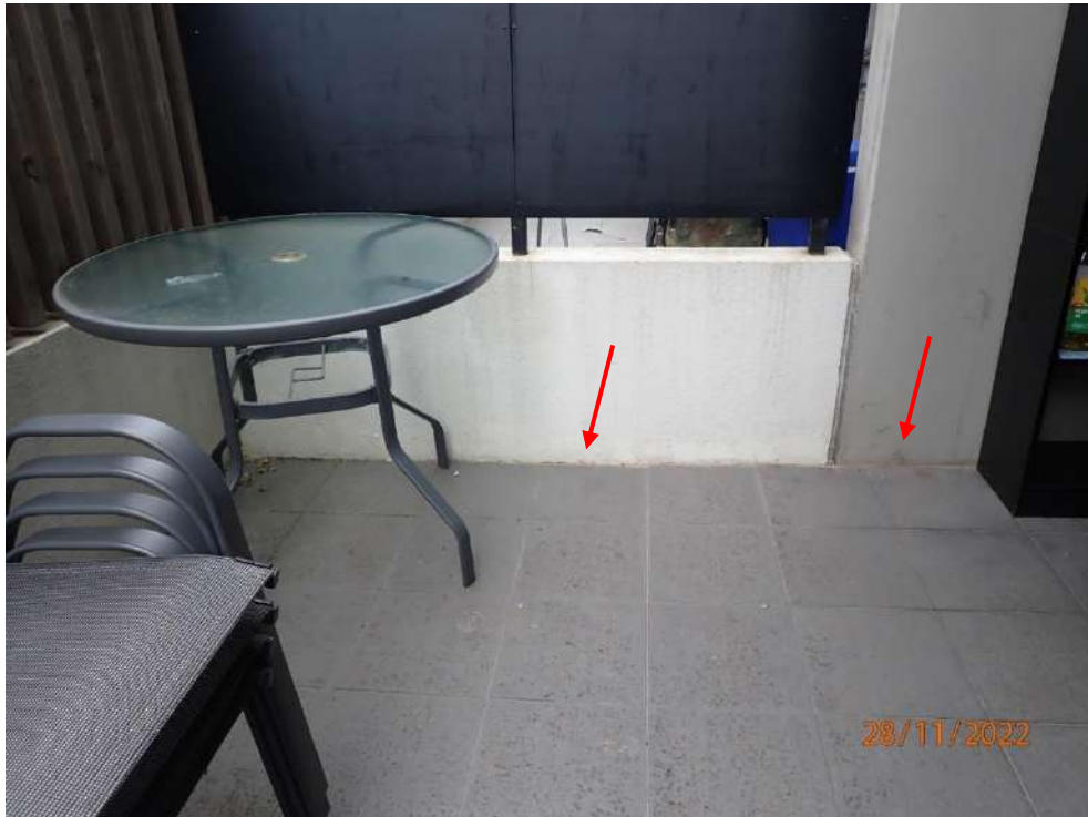
Photograph 103 - Apartment 123B balcony, omission of waterproofing upturns
