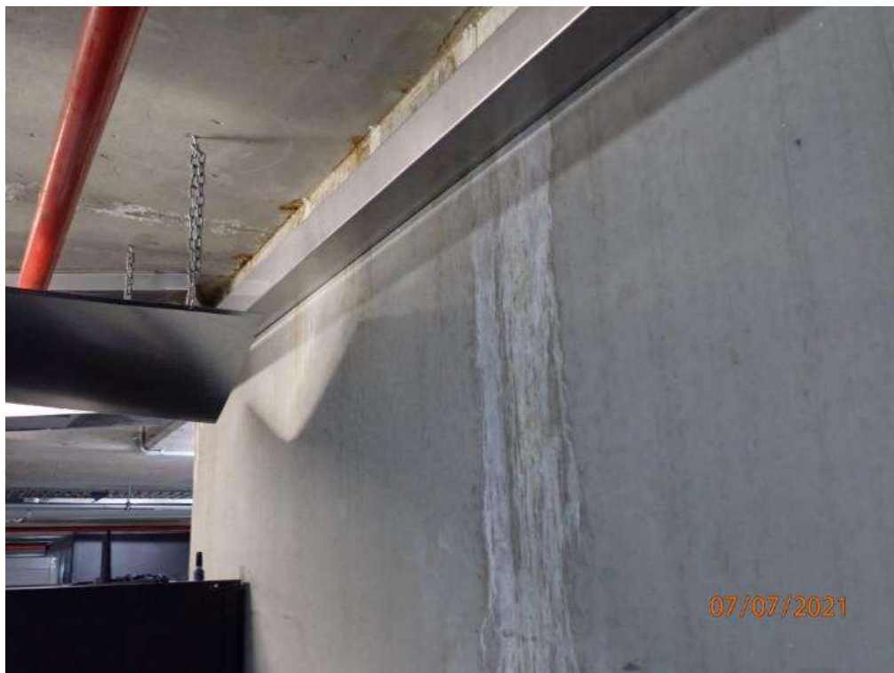
Photograph 58 - Drip tray installed below efflorescence, severe calcium build up and rust deposits
