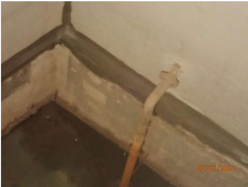
Photograph 92 – Water tanks not cleaned out ready for water testing
