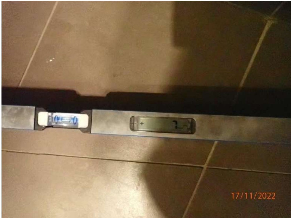
Photograph 7 - Apartment 309A bathroom shower fall 1 in 143
