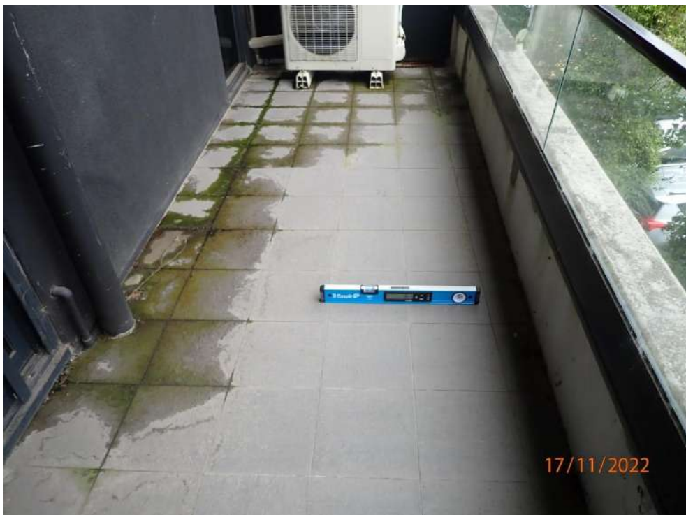
Photograph 14 - Apartment 308A balcony fall
