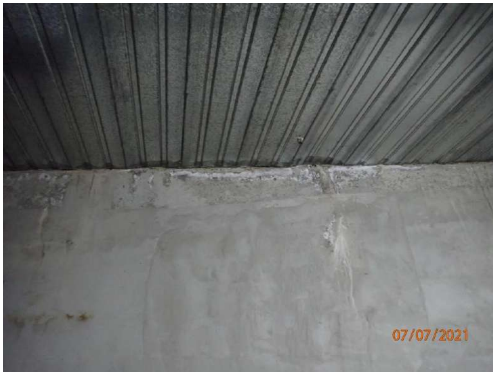
Photograph 2 - Efflorescence and Bondek rusted to southwest corner of bin room
