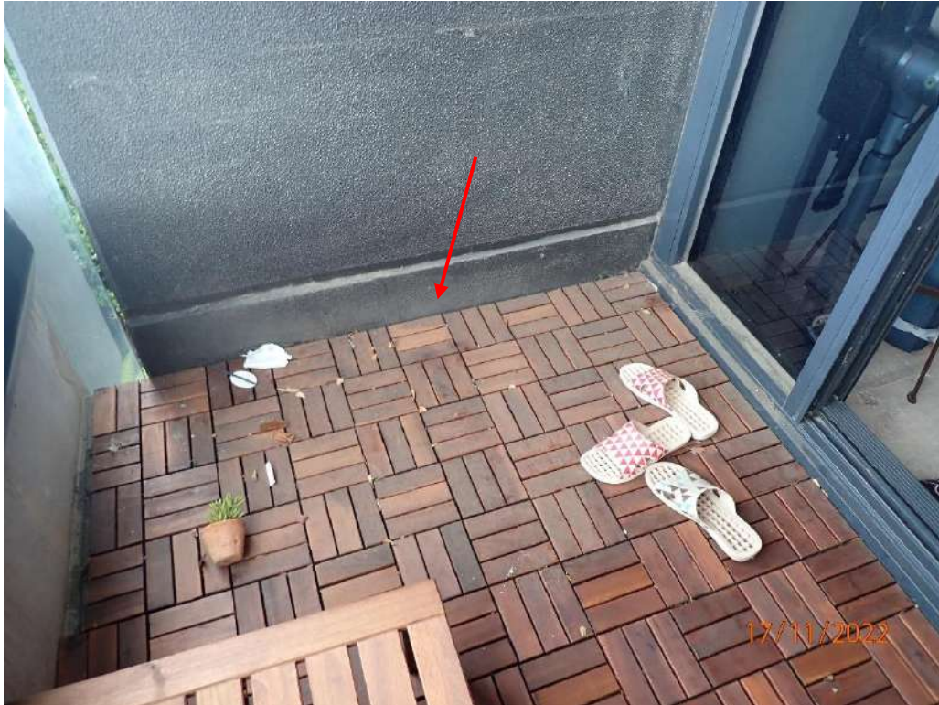
Photograph 25 – Apartment 410A, balcony floor/wall junction above affected area to Apartment 309A missing upturn detail
