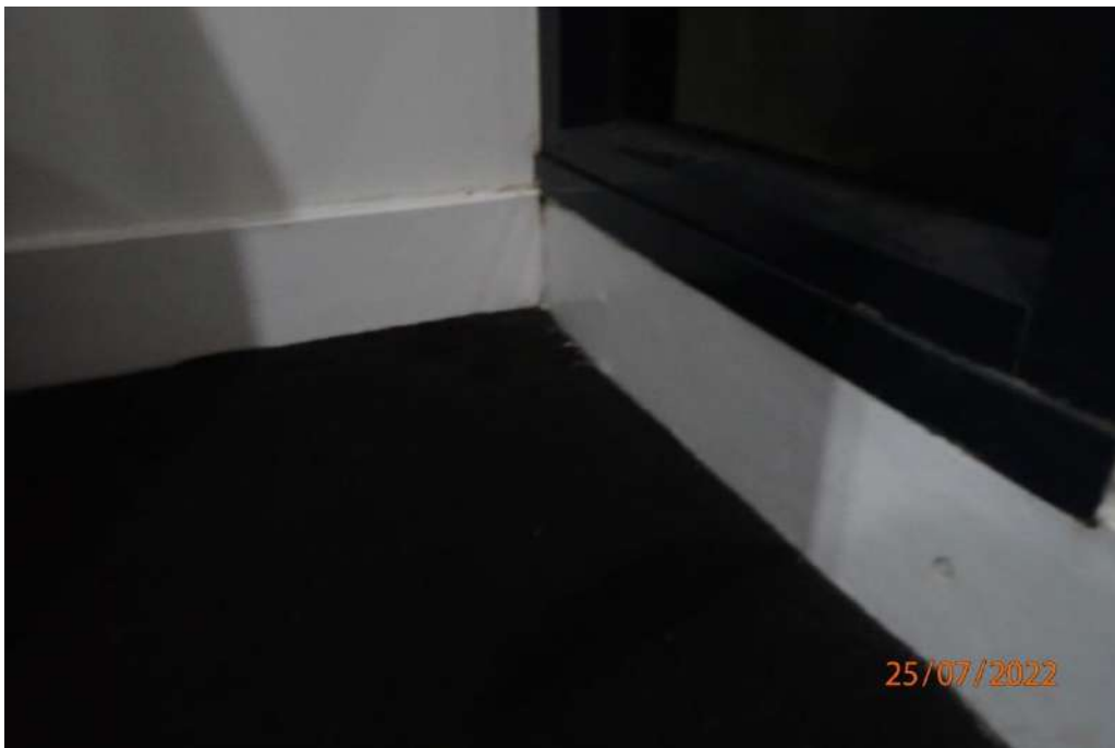
Photograph 142 - Lot 106B/Apartment 116B, northwest corner of bedroom skirting trim
