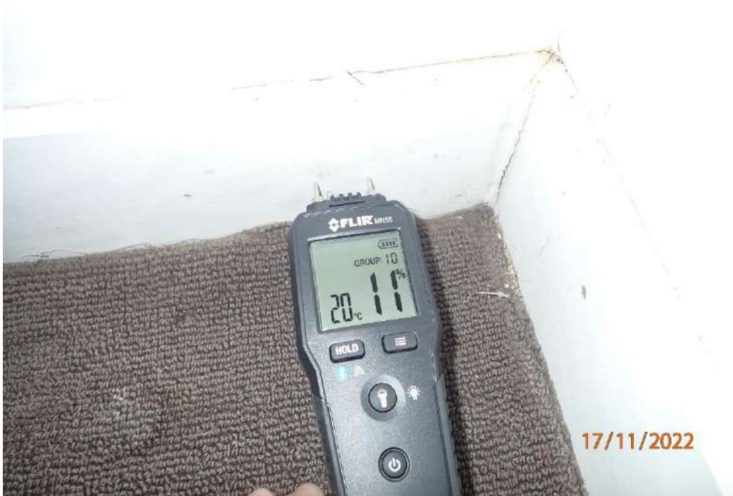
Photograph 64 - Apartment 417B, northwest corner of the living area, low to moderate moisture readings in skirting trim
