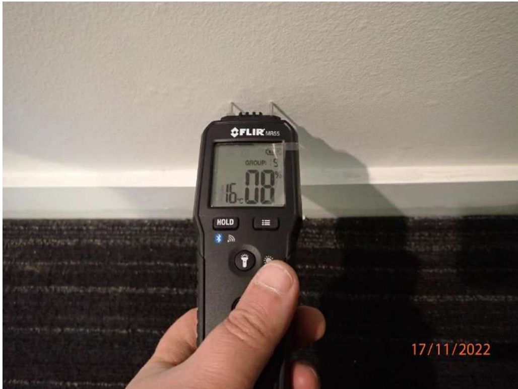
Photograph 43 - Common passageway outside Apartment 328B, moderate to low moisture levels
