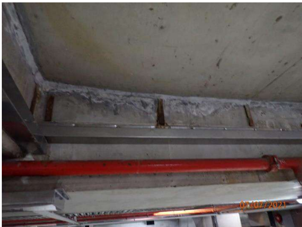
Photograph 22 - Efflorescence, severe calcification build-up and rusty steel components to concrete beams and pipe penetrations near carpark 48 including surrounding carparks
