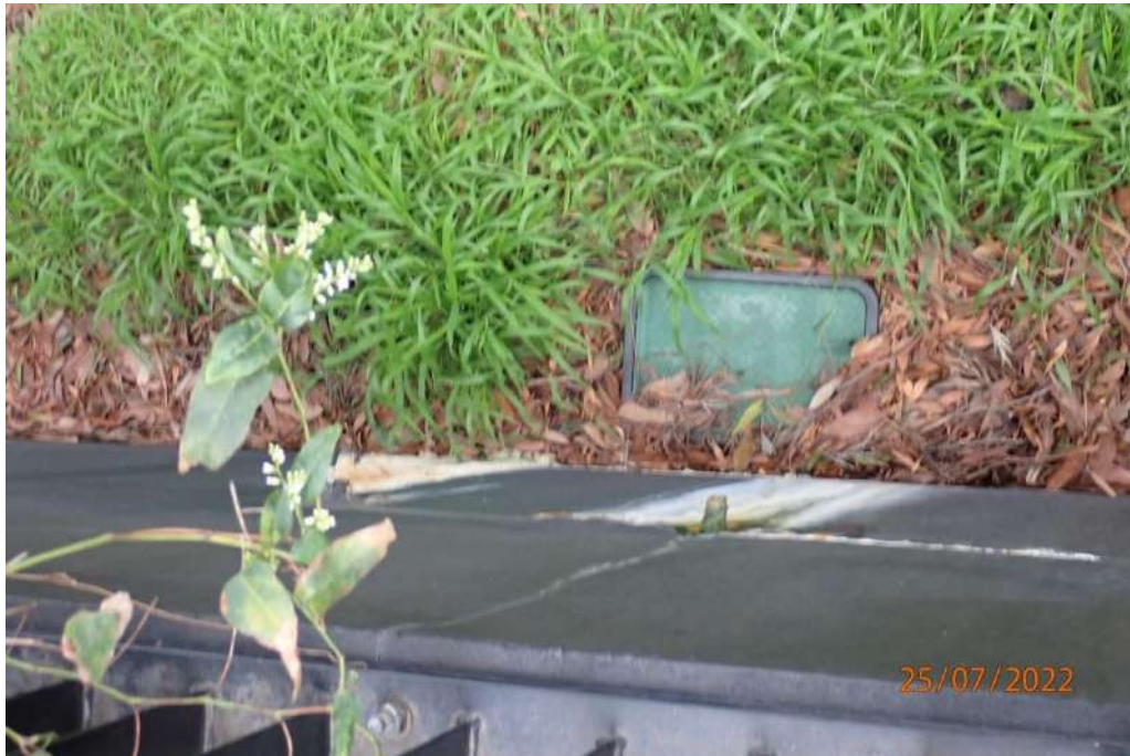
Photograph 149 - Lot 109A/Apartment 109A, planter box overflow outlet
