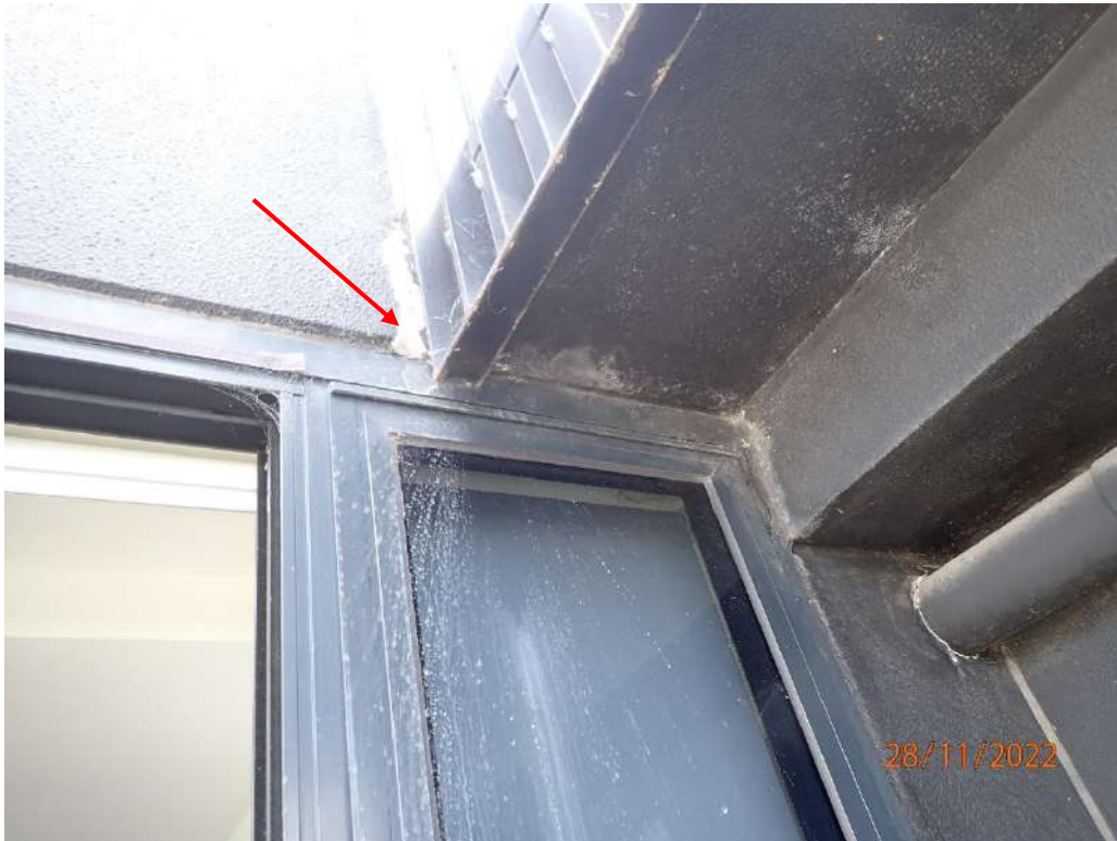
Photograph 101 - Apartment 604B, possible area of water ingress adjacent to pelmet area
