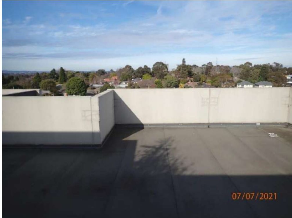
Photograph 111 – Fill is cracking away at tension plates
