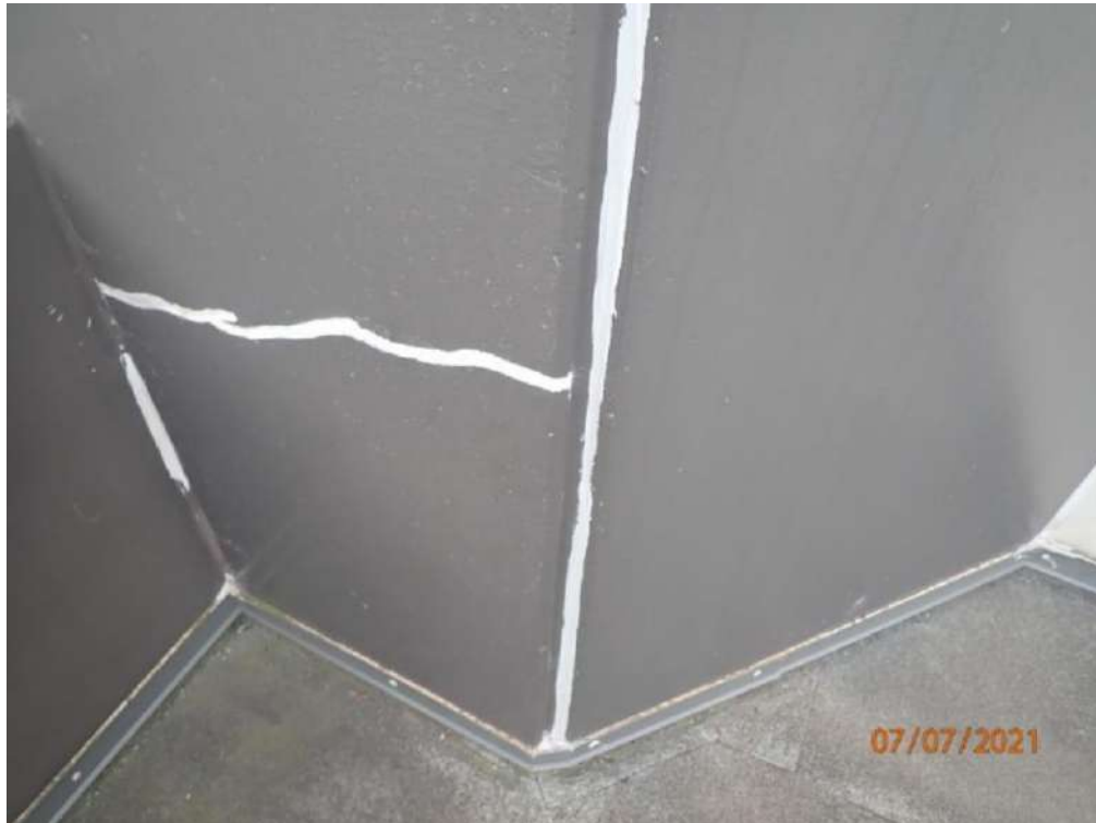
Photograph 101 – Filled cracking to concrete wall panels to north elevation of building A
