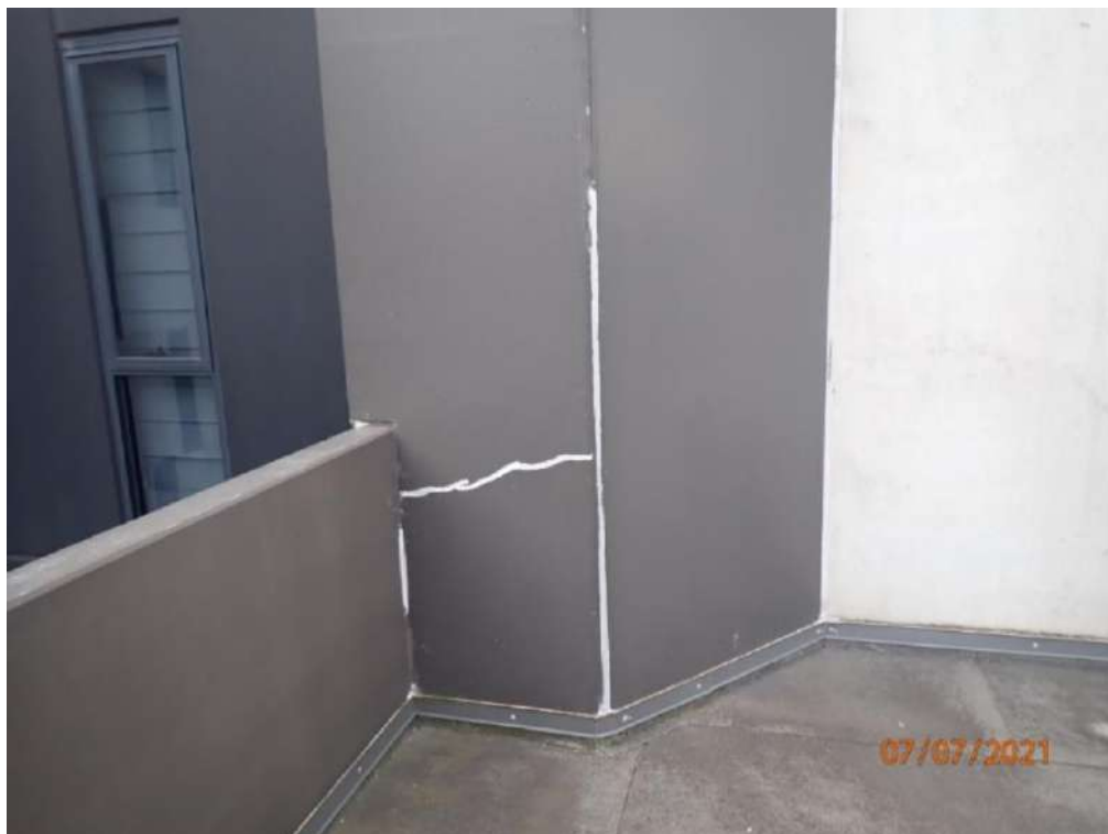
Photograph 102 – Filled cracking to concrete wall panels to north elevation of building A
