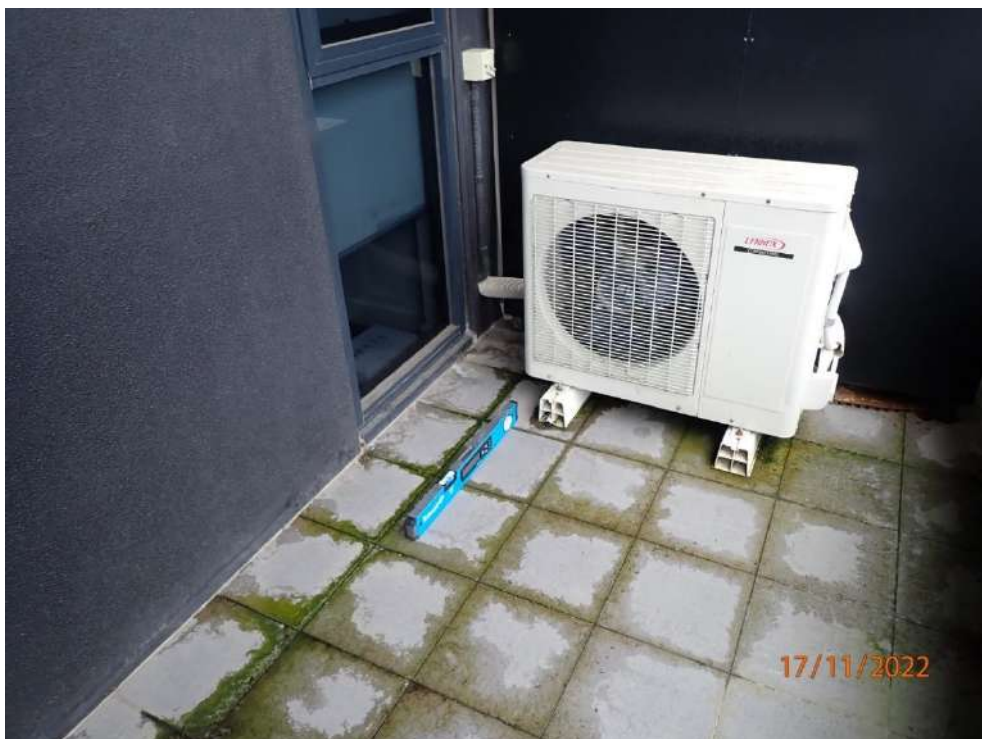
Photograph 16 - Apartment 308A balcony fall
