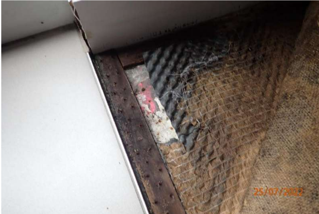
Photograph 199 - Lot 607B/Apartment 605B, north end of west wall opening to the balcony, damage to carpet
