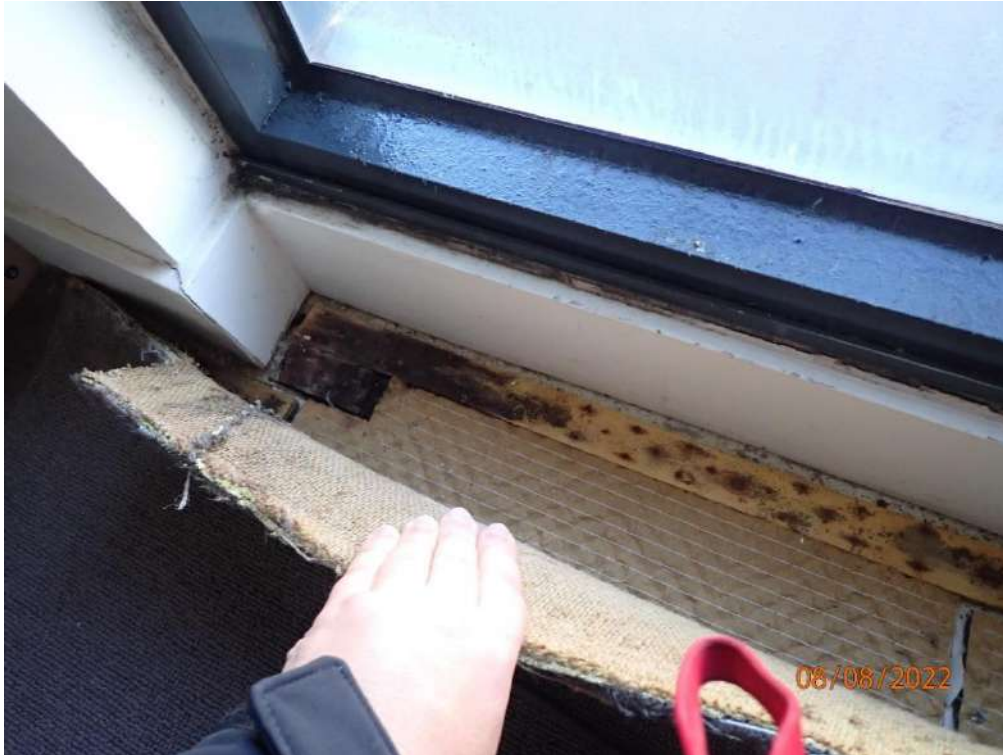
Photograph 205 - 704B/Apartment 703B, west window of the south bedroom, damage to carpet and smooth edge
