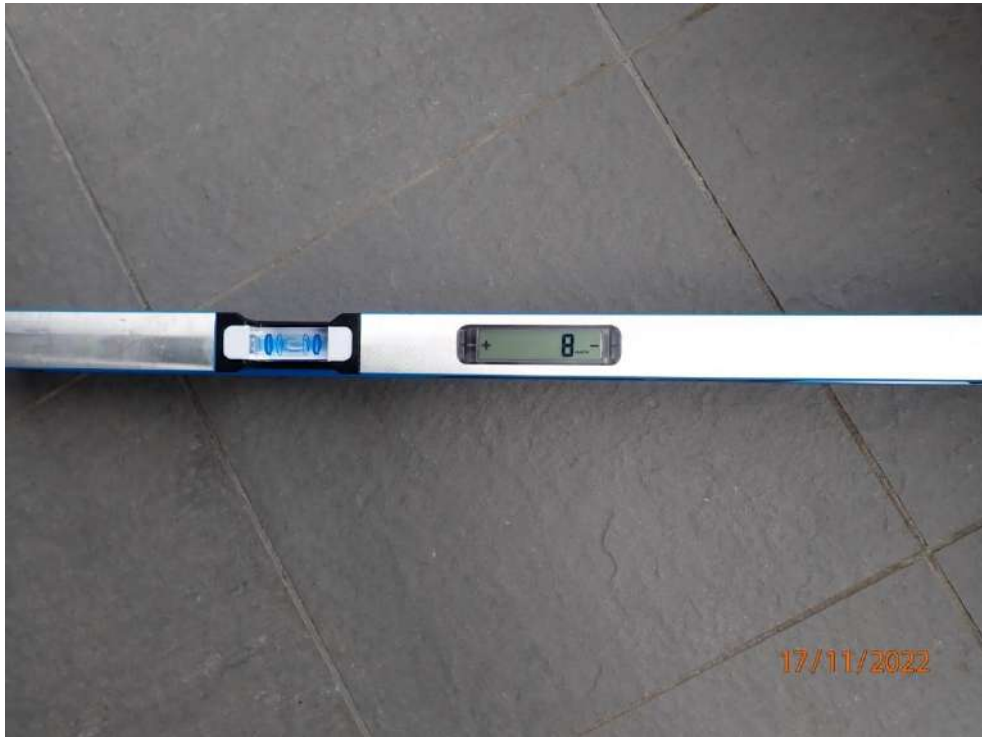
Photograph 13 - Apartment 308A balcony fall 1 in 125
