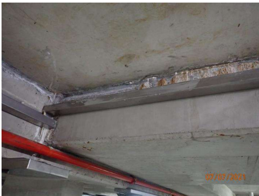
Photograph 28 - Efflorescence, severe calcification build-up and rusty steel components to concrete beams and pipe penetrations near carpark 48 including surrounding carparks
