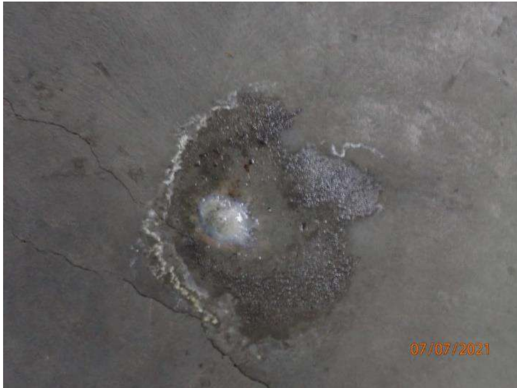
Photograph 17 - Calcium deposits to concrete slab of carpark 65
