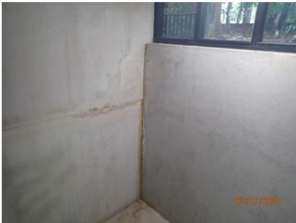
Photograph 78 - Efflorescence, water staining and cracking of concrete to staircase 01 adjacent planter box
