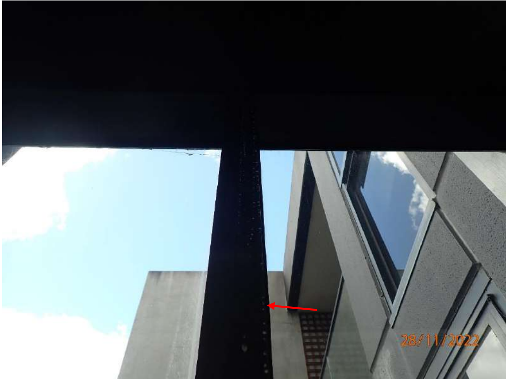
Photograph 85 - Level 4 south passageway aluminium windows, water stains
