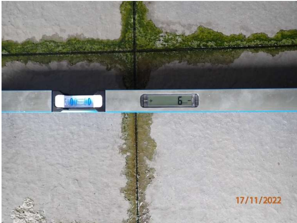
Photograph 17 - Apartment 308A balcony fall 1 in 167
