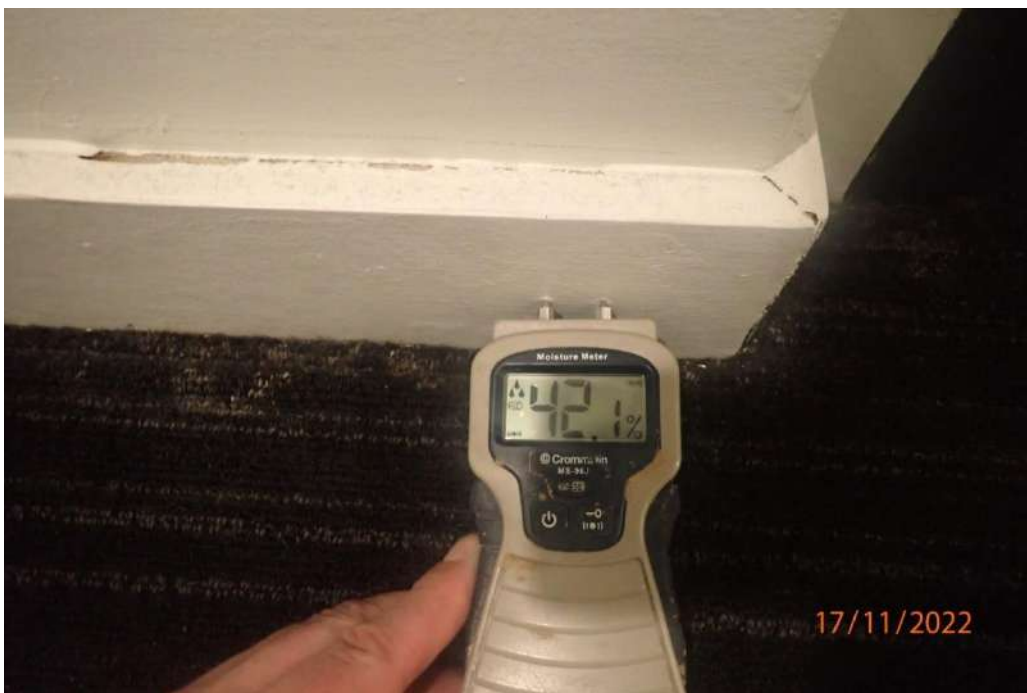
Photograph 118 - Apartment 521B external passageway, elevated moisture levels in skirting trim
