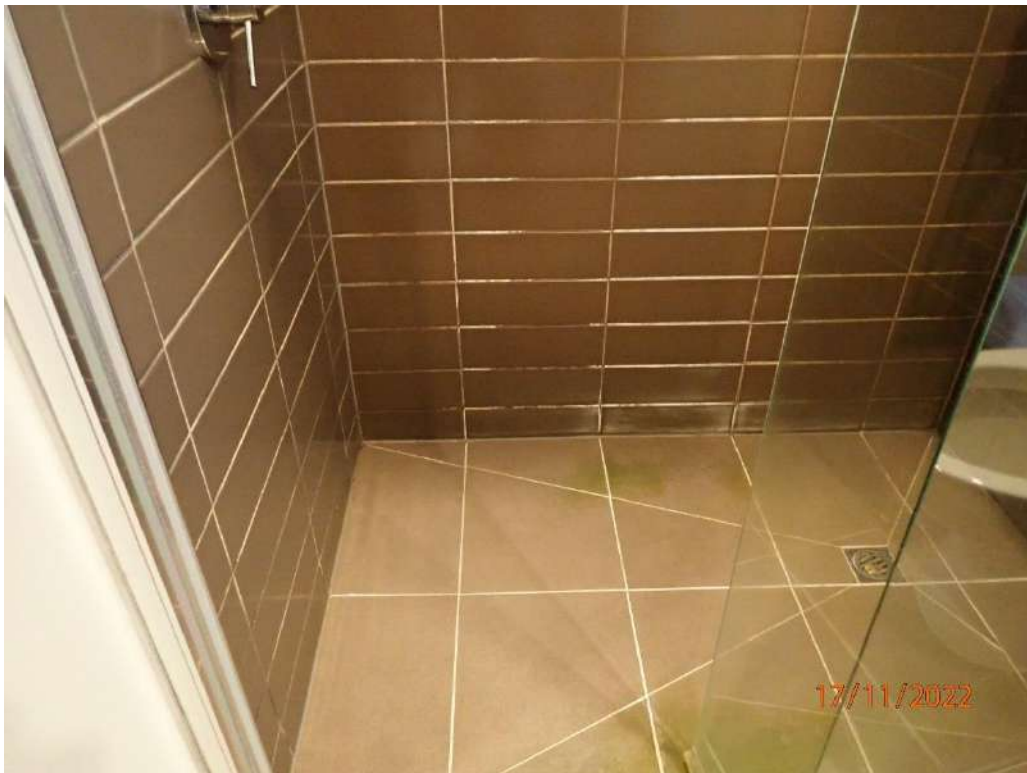
Photograph 26 – Apartment 526B bathroom shower
