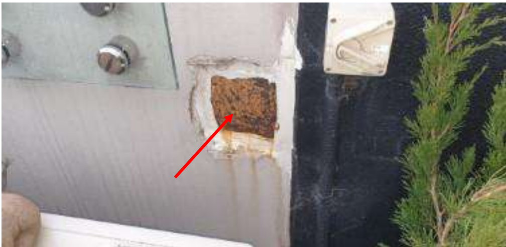
Photograph 218 - Lot 713B/Apartment 712B main balcony wall cast in plates (photo taken on Samsung mobile phone on 25 July 2022 by Peter Kyriakou)
