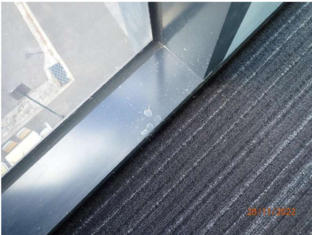
Photograph 84 - Level 4 south passageway aluminium windows, water stains
