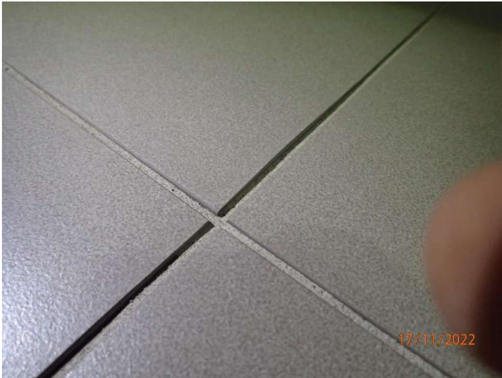
Photograph 39 - Apartment 328B bathroom shower recessed grout lines
