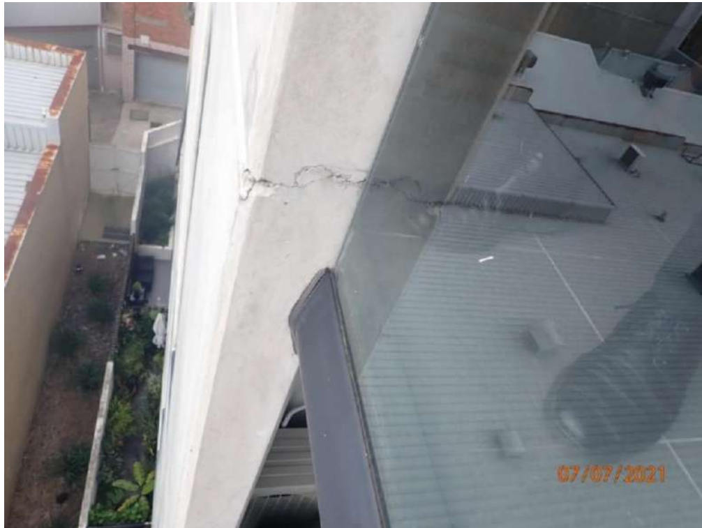
Photograph 97 – Cracking at expansion joints to south elevation of building B
