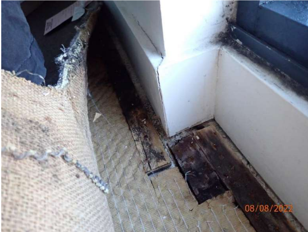
Photograph 207 - 704B/Apartment 703B, west window of the south bedroom, damage to carpet and smooth edge
