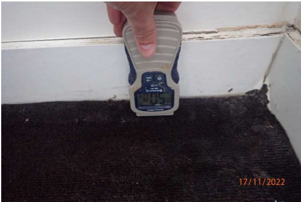
Photograph 114 - Apartment 126B, southeast corner of bedroom 2, high moisture elevation in carpet and underlay
