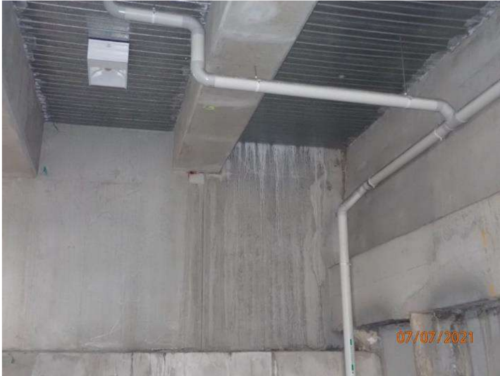
Photograph 67 - Efflorescence and calcium build up to the east end of basement carpark
