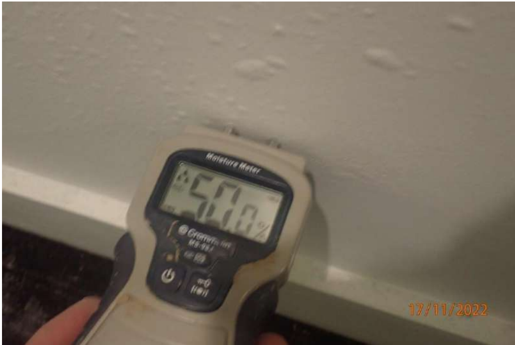
Photograph 121 - Apartment 521B external passageway, elevated moisture levels in wall plaster
