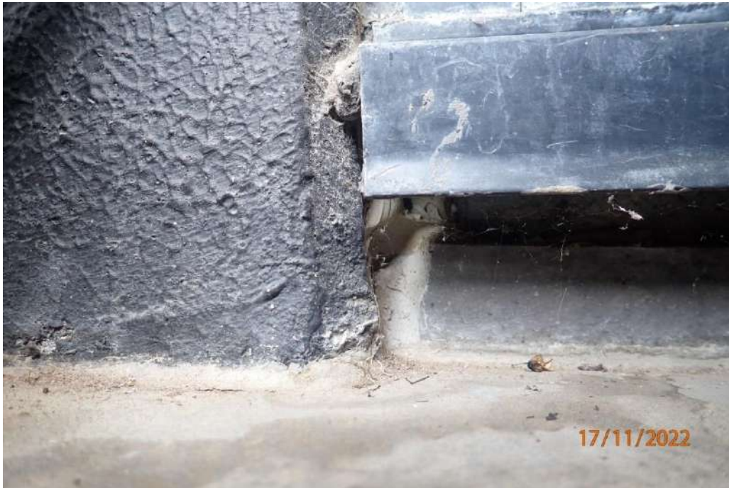
Photograph 109 - Apartment 205A balcony upturn beneath aluminium sliding door and window unit
