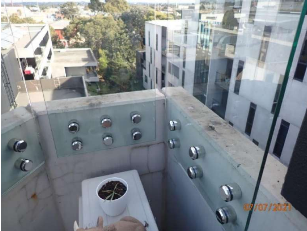
Photograph 113 – Fill is cracking away at tension plates
