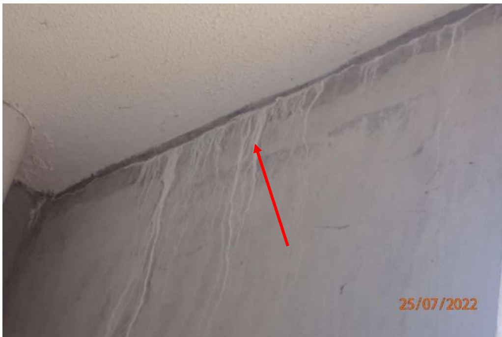
Photograph 192 - Lot 418B/Apartment 428B, north east balcony soffit, efflorescence visible from Lot 321B/Apartment 333B
