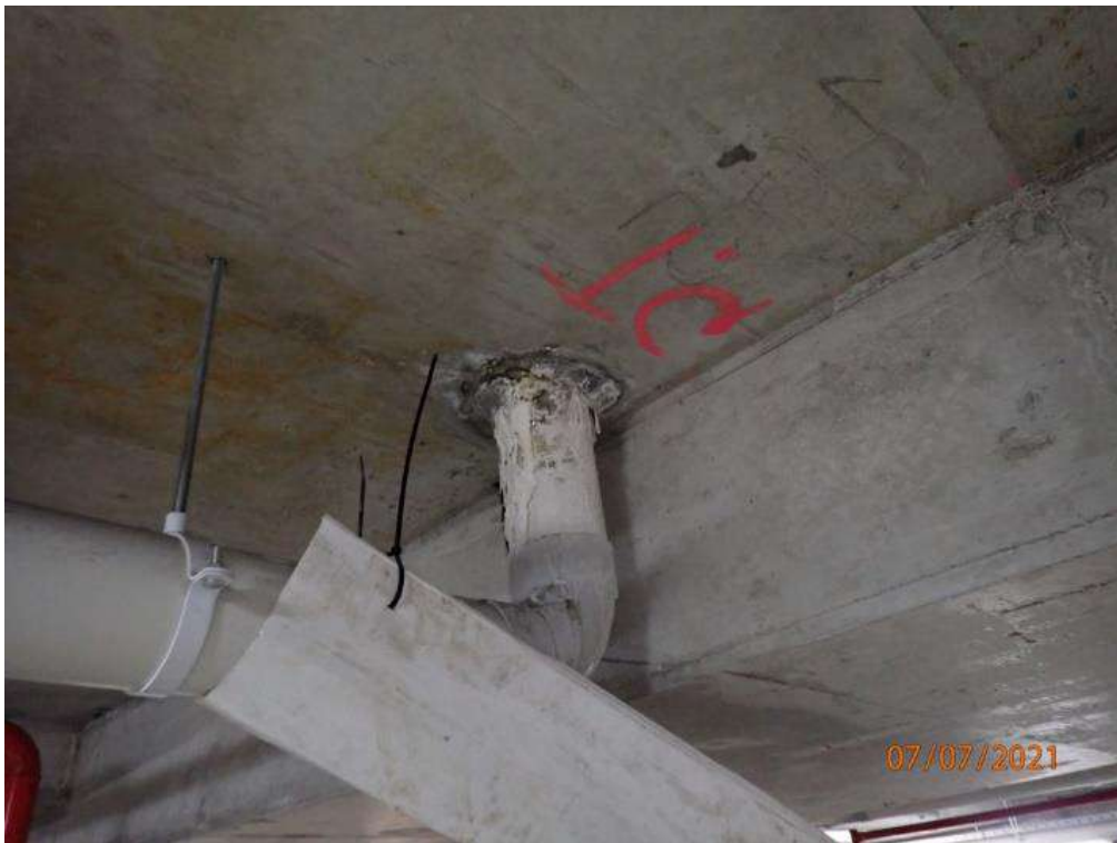
Photograph 34 – Efflorescence and calcification build-up at pipe penetrations
