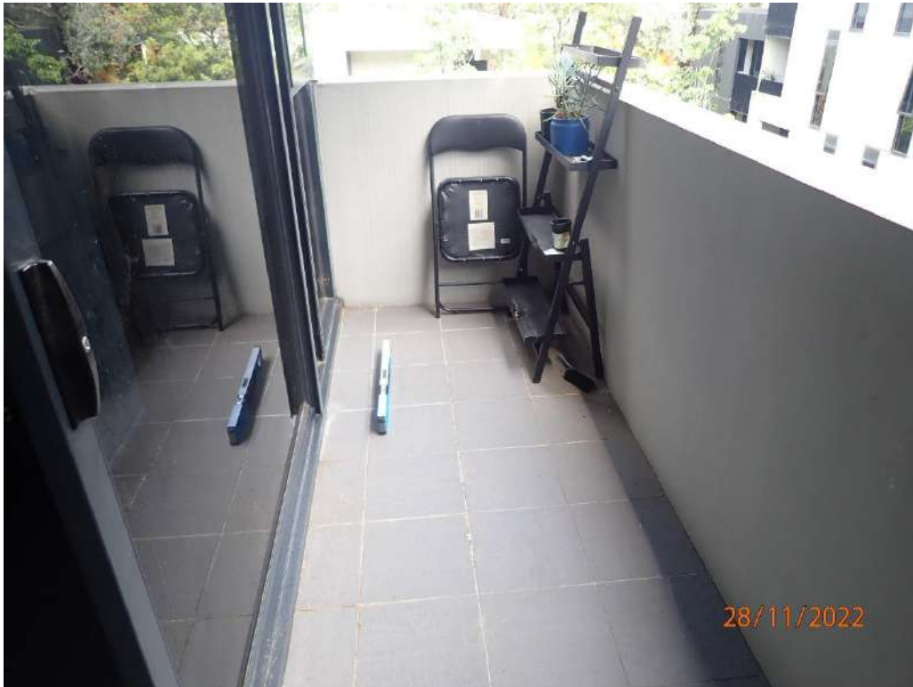
Photograph 93 - Apartment 431B balcony fall
