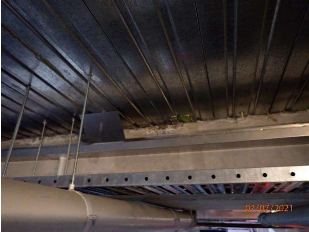
Photograph 45 – Efflorescence and calcium build up
