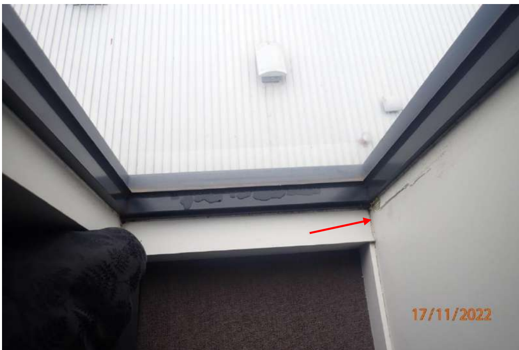
Photograph 124 – Apartment 607B, bedroom window, plaster damage
