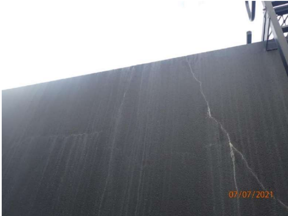
Photograph 105 – Cracking to concrete wall panels to north elevation of building A
