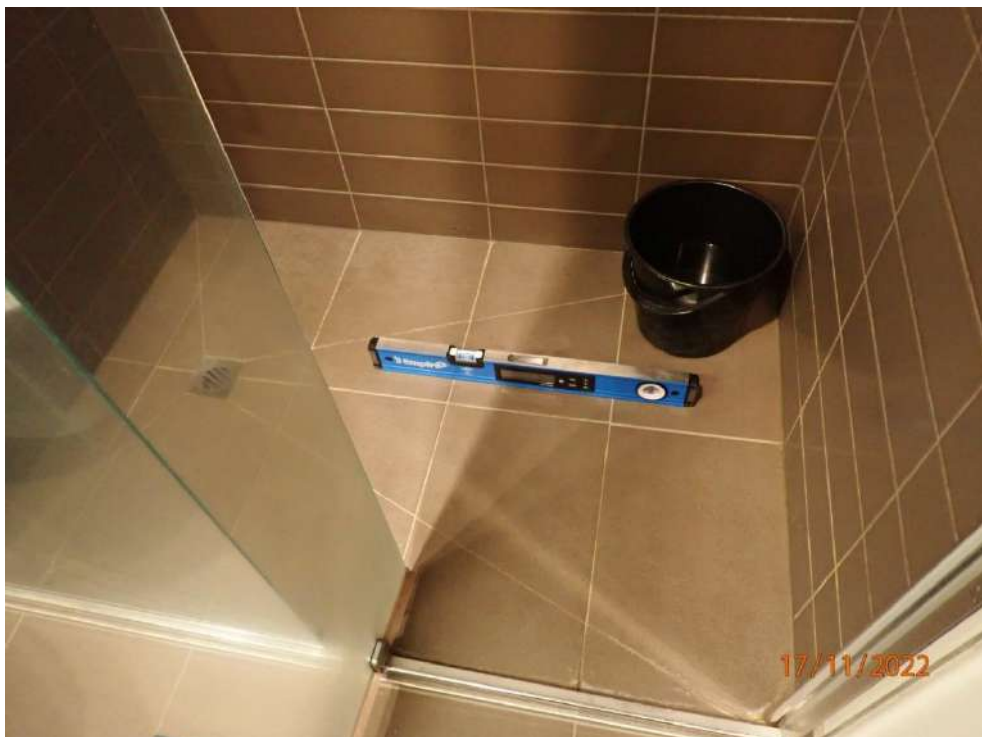
Photograph 4 - Apartment 309A bathroom shower
