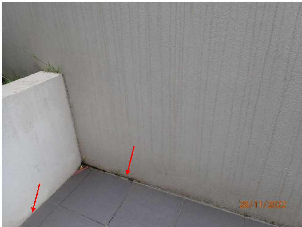
Photograph 102 – Apartment 123B balcony, omission of waterproofing upturns
