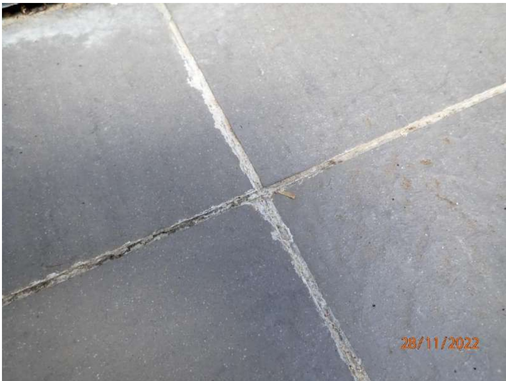
Photograph 98 - Apartment 431B balcony, efflorescence between grout lines
