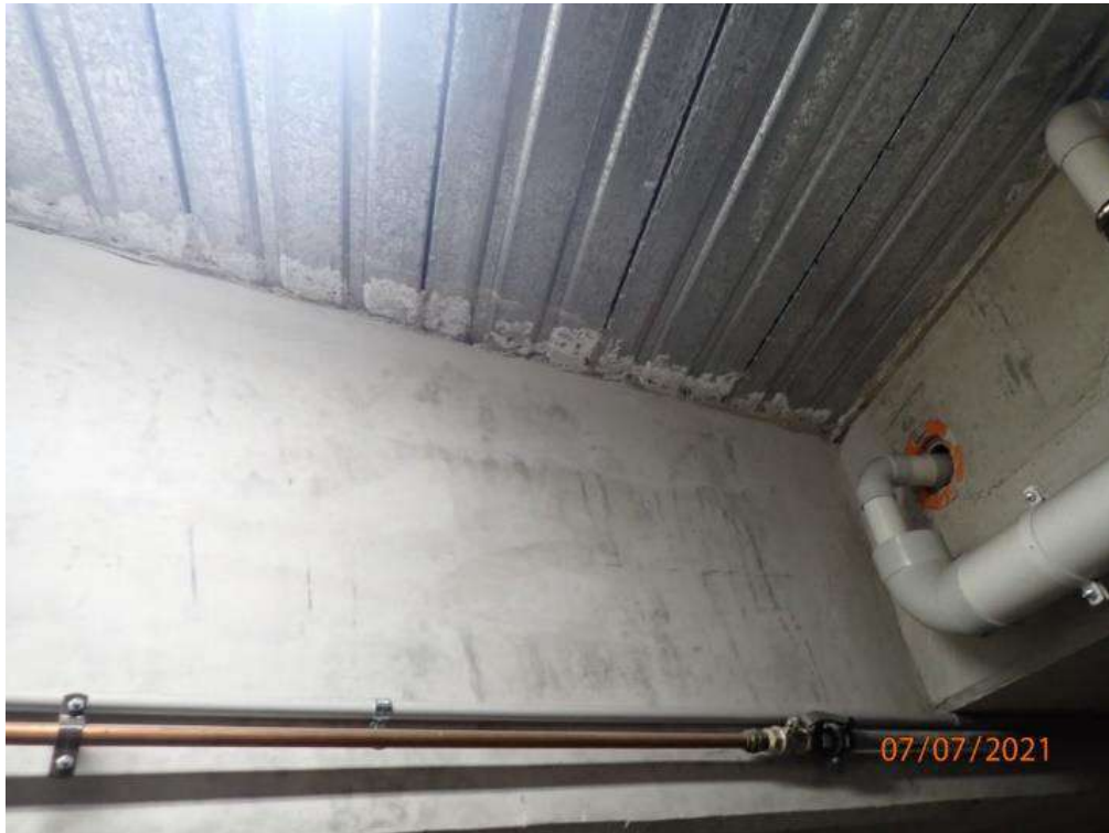
Photograph 3 - Efflorescence and Bondek rusted to carpark 73 southwest corner
