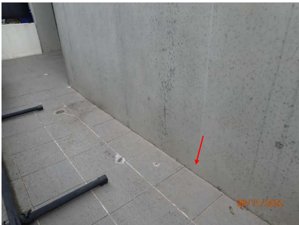
Photograph 104 - Apartment 123B balcony, omission of waterproofing upturns
