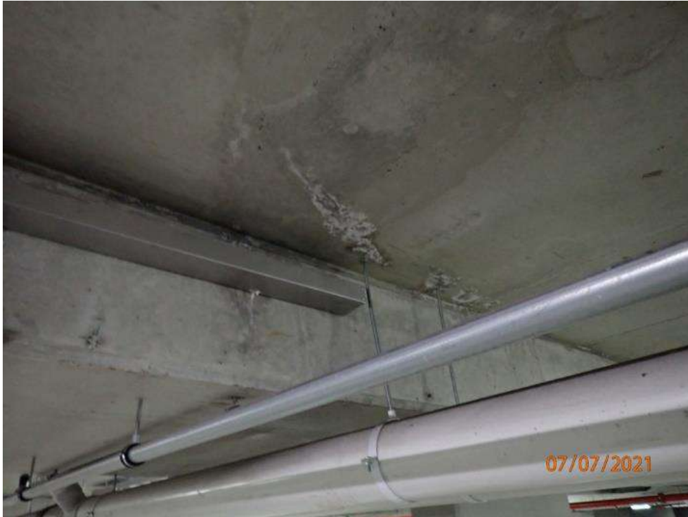
Photograph 31 - Efflorescence, calcification and cracks forming in the concrete ceiling
