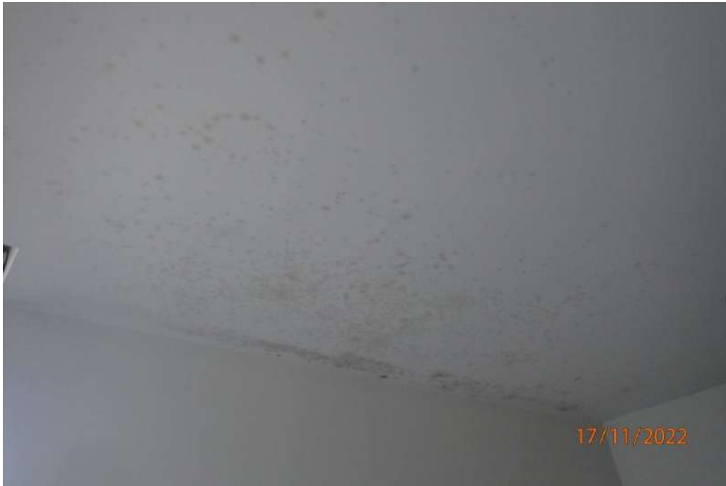
Photograph 135 - Apartment 510A, bedroom ceiling, mould growth in view
