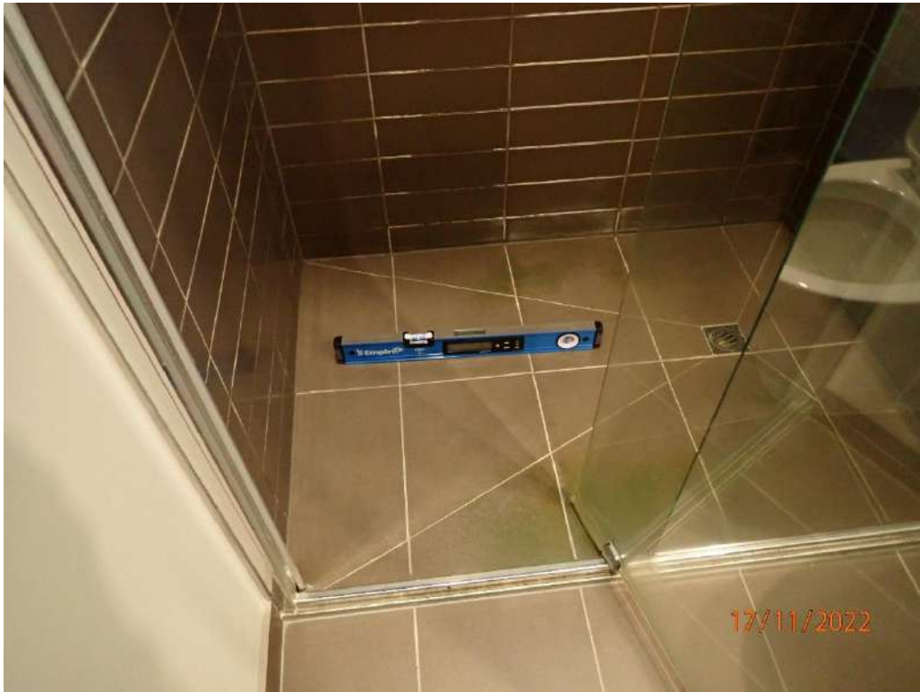
Photograph 27 - Apartment 526B bathroom shower fall
