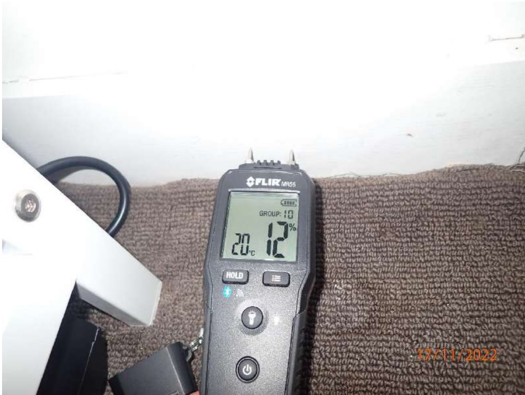
Photograph 63 - Apartment 417B, northwest corner of the living area, low to moderate moisture readings in skirting trim
