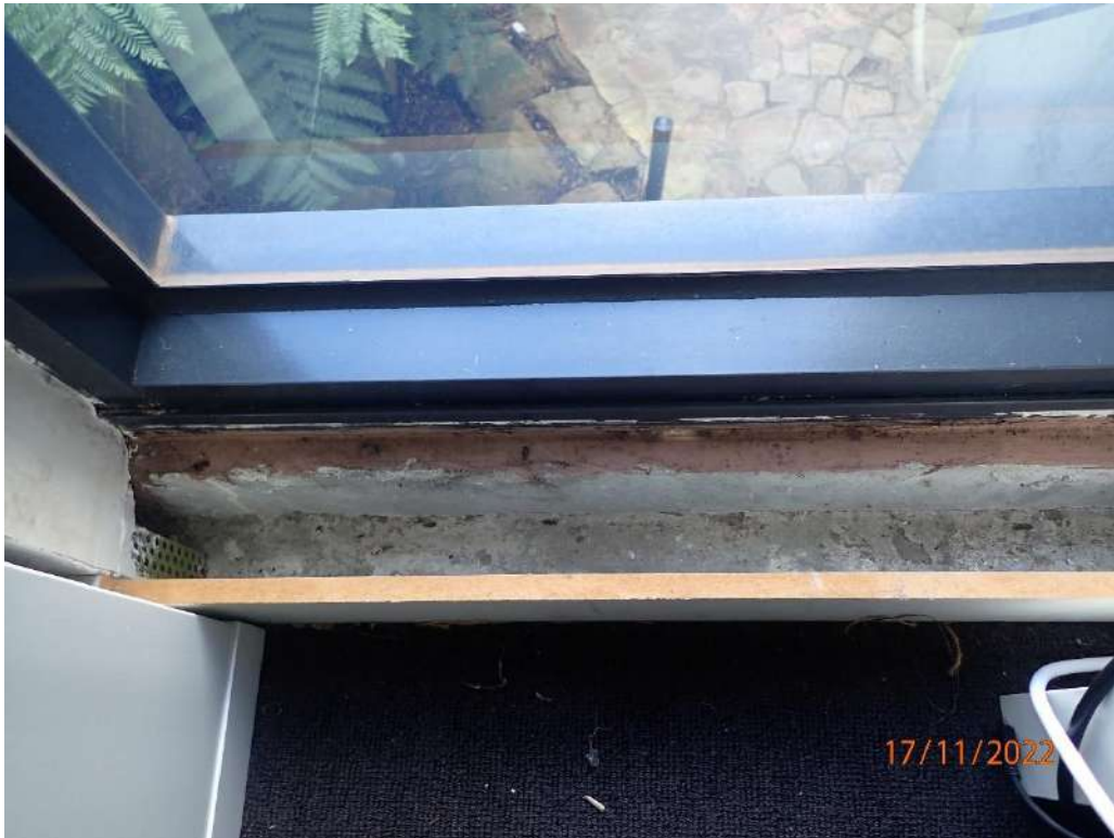
Photograph 47 - Apartment 337B, bedroom 2 window, incomplete repairs to window sill reveal and adjacent wall plaster
