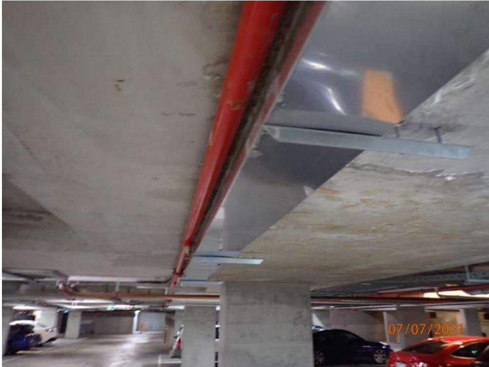
Photograph 49 – Metal tray installed throughout centre of basement carpark
