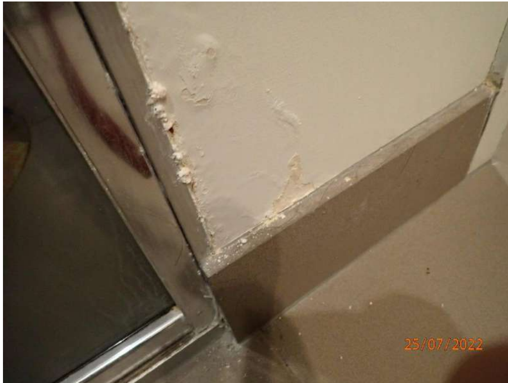
Photograph 165 - Lot 306A/Apartment 306A, moisture damaged wall right of the shower
