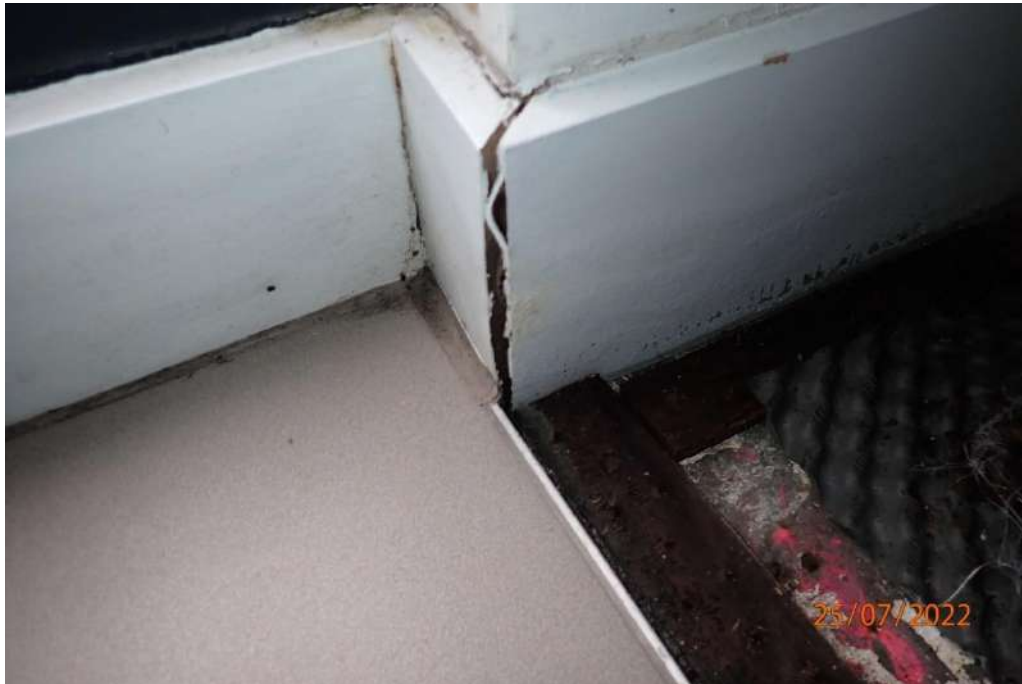
Photograph 195 - Lot 607B/Apartment 605B, west wall opening to the balcony, skirting trim
