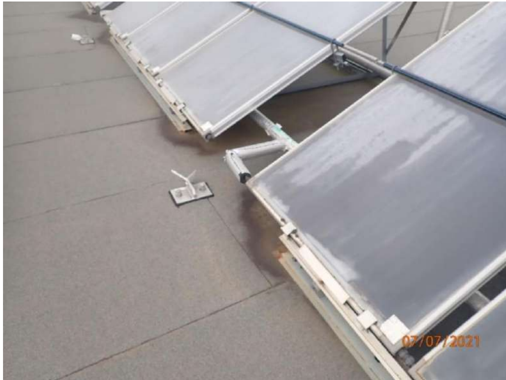
Photograph 129 – Water staining to external edges and around solar panels to building A
