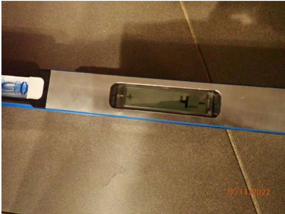
Photograph 3 - Apartment 309A bathroom shower fall 1 in 250
