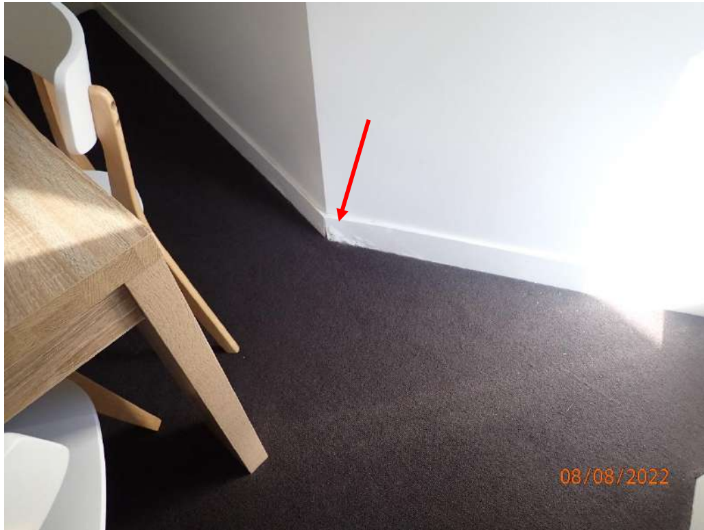
Photograph 185 - Lot 402A/Apartment 402A living area west wall skirting trim
