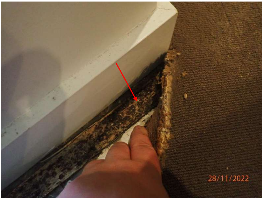
Photograph 74 – Apartment 109A, water ingress to bedroom 2 west window
