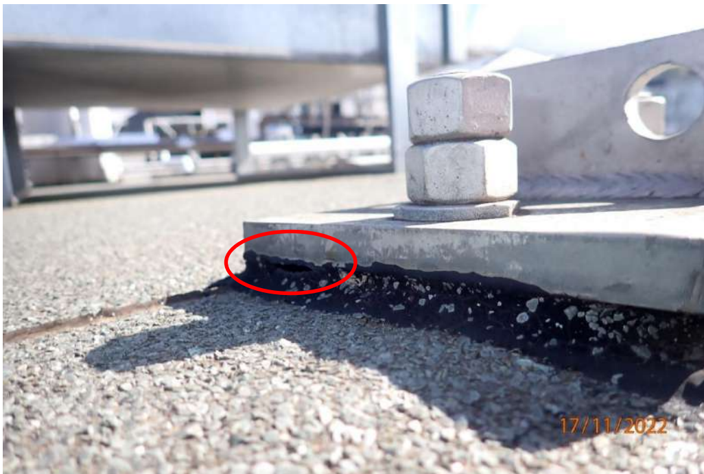
Photograph 138 - Rooftop above Apartment 510A bedroom, gaps in anchor point sealant
