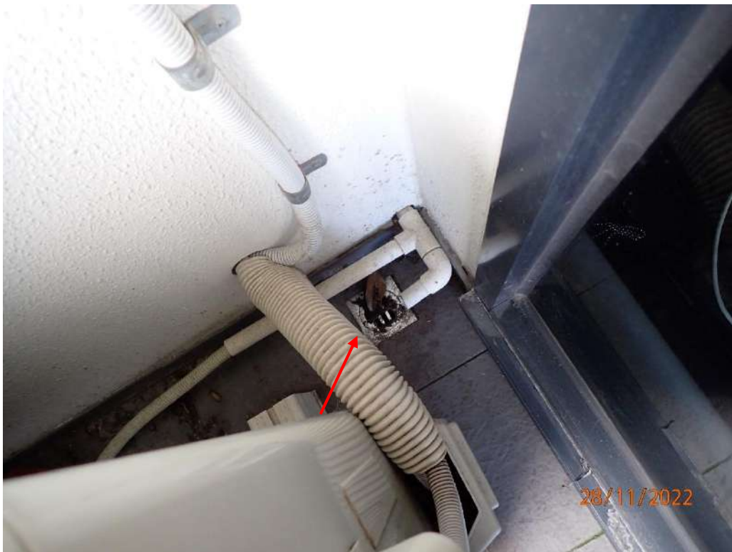
Photograph 88 - Apartment 431B balcony, drainage outlet
