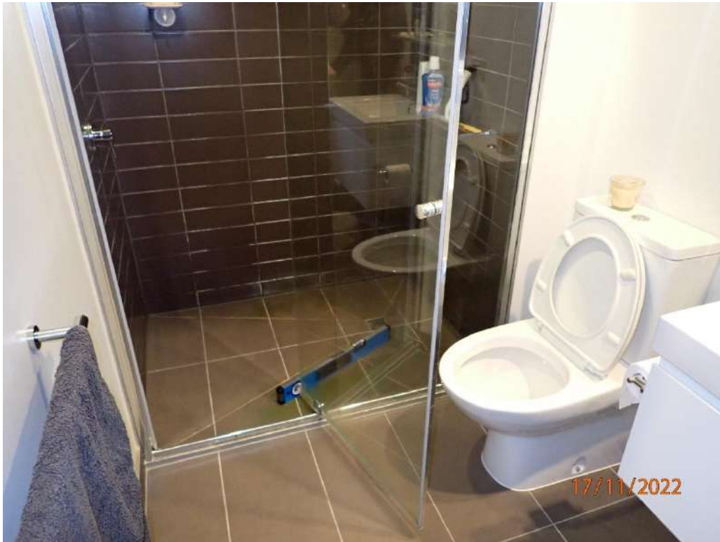
Photograph 29 - Apartment 526B bathroom shower fall
