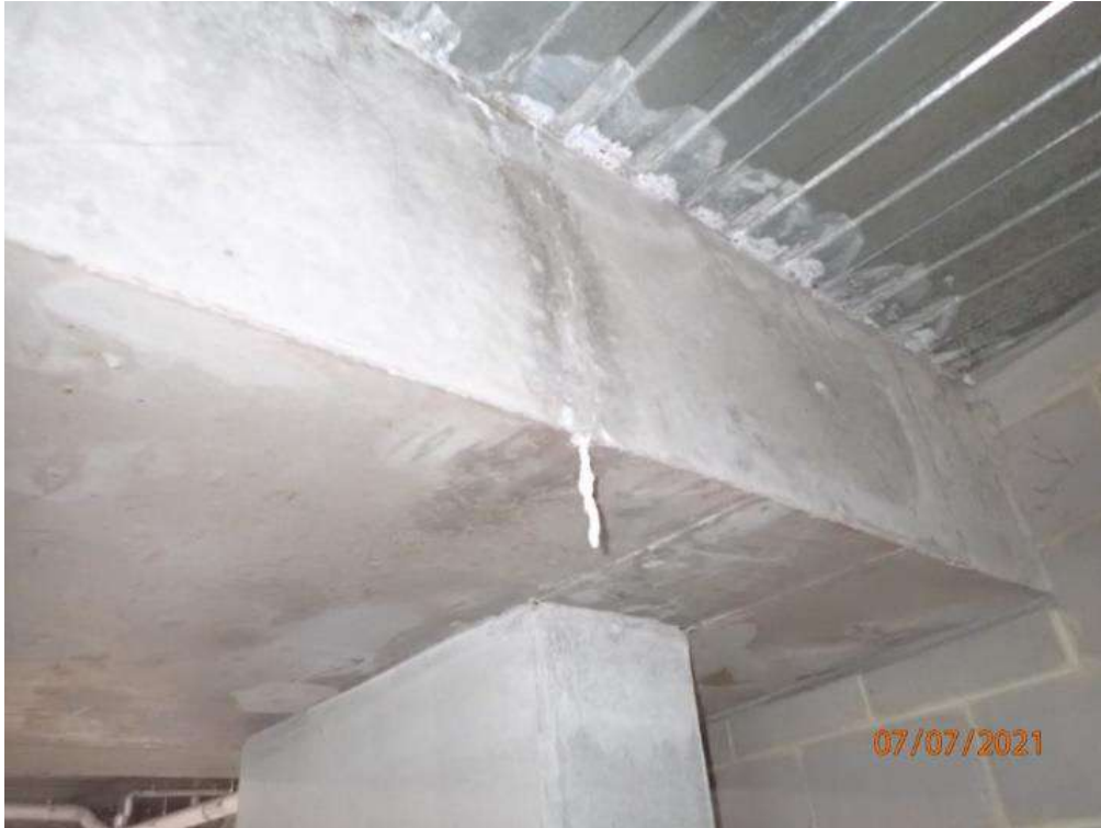
Photograph 63 – Efflorescence and calcium build up to the east end of basement carpark
