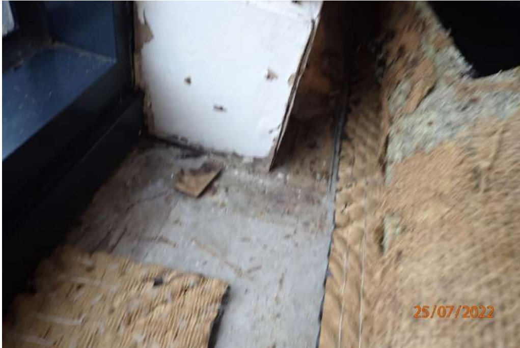
Photograph 177 - Lot 321B/Apartment 333B, damaged carpet adjacent to the window on the south wall of the living area
