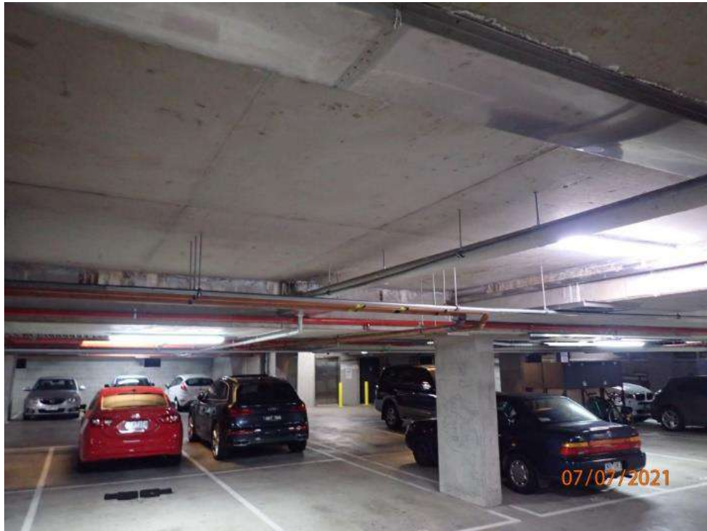
Photograph 37 - Metal tray extends through centre of basement carpark
