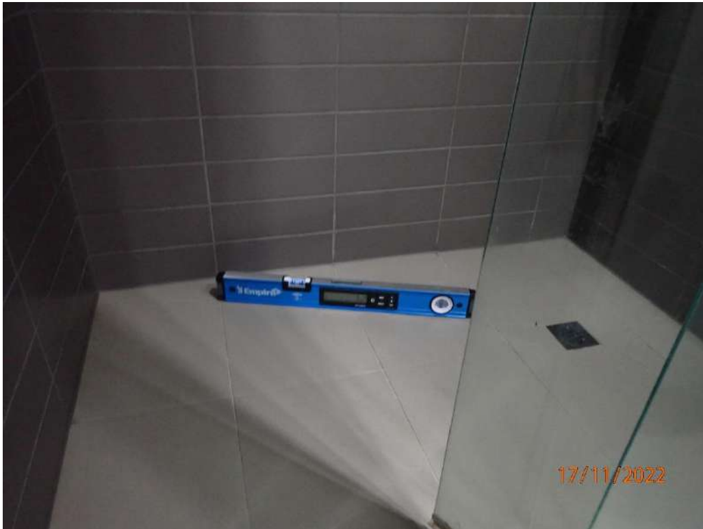
Photograph 35 - Apartment 328B bathroom shower fall
