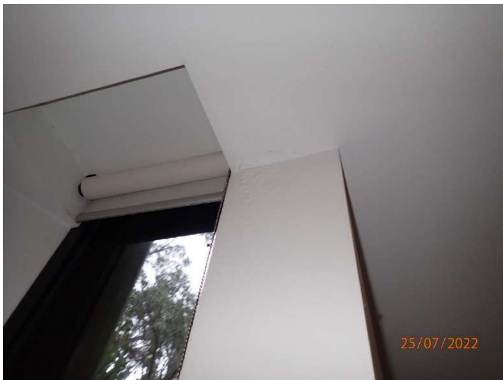
Photograph 156 – Lot 208A/Apartment 208A, bedroom window, moisture damage to wall and ceiling
