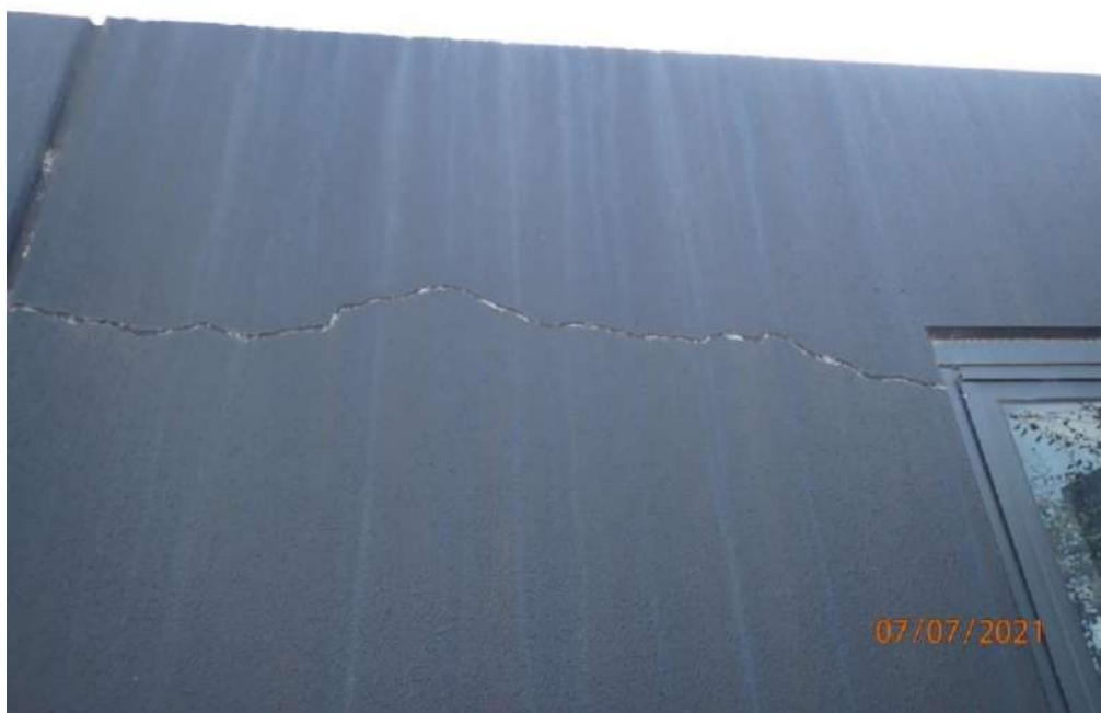
Photograph 96 – Cracking to west elevation of building B
