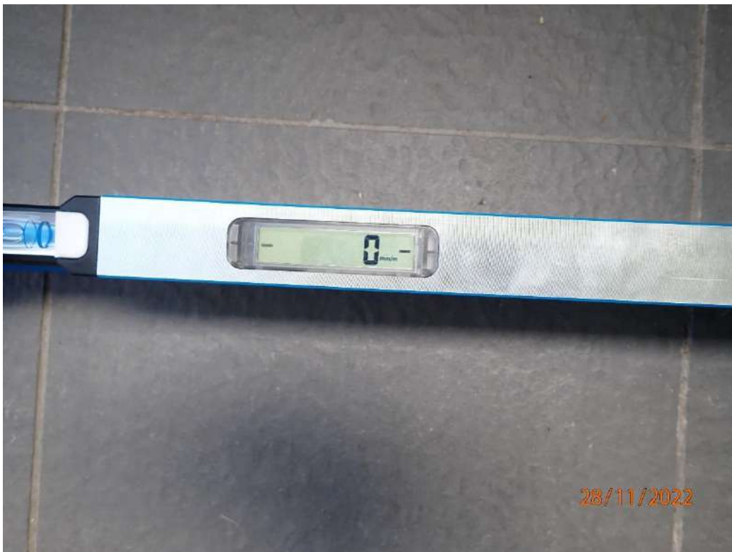
Photograph 90 - Apartment 431B balcony, no fall
