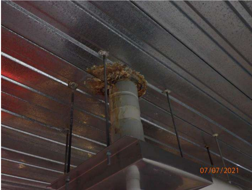
Photograph 35 – Efflorescence and calcification build-up at pipe penetrations
