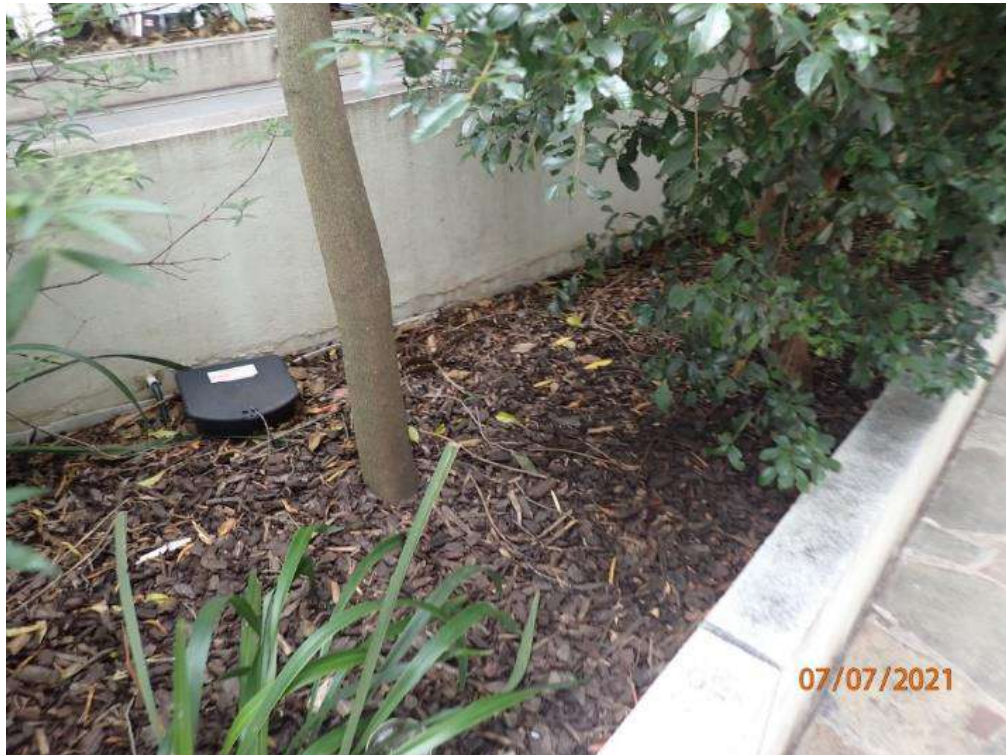
Photograph 71 - Waterproof membrane does not extend above the soil level
