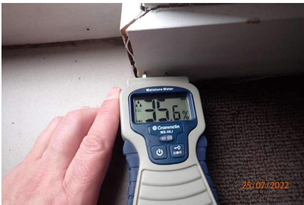
Photograph 196 - Lot 607B/Apartment 605B, north end of west wall opening to the balcony, elevated moisture reading 35.6%
