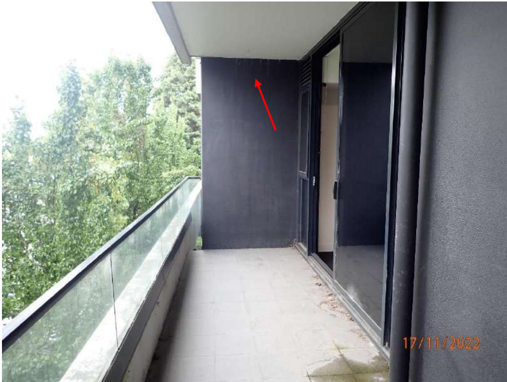
Photograph 21 - Apartment 308A balcony west wall
