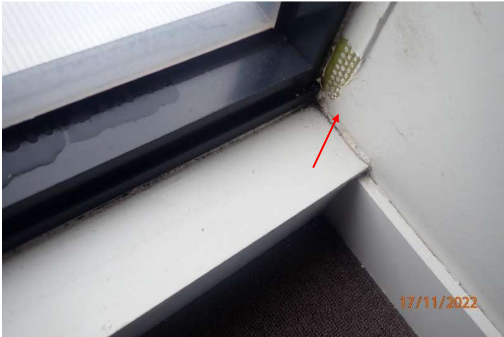
Photograph 125 - Apartment 607B, bedroom window, plaster damage
