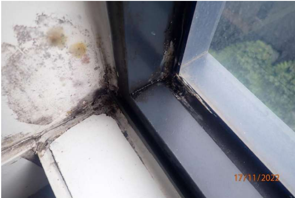
Photograph 129 - Apartment 602B, bedroom window, water damage to adjacent wall plaster
