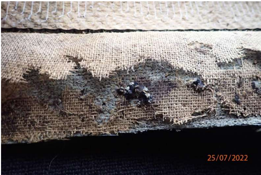
Photograph 176 - Lot 321B/Apartment 333B, damaged carpet adjacent to the window on the south wall of the living area
