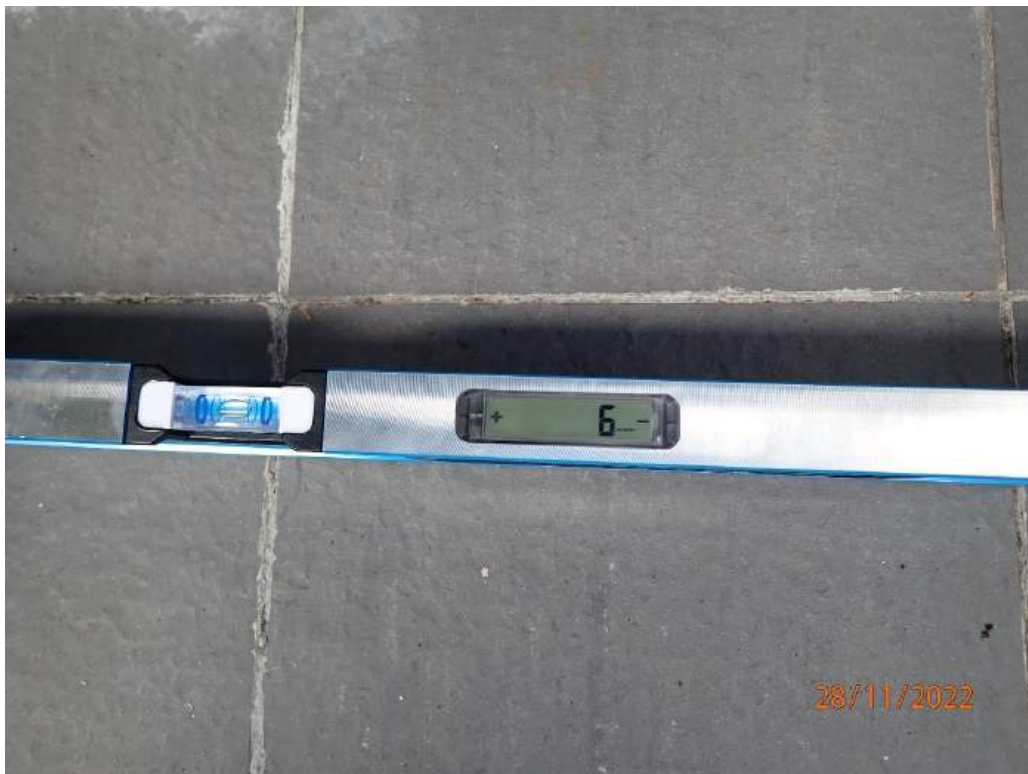
Photograph 94 - Apartment 431B balcony fall 1 in 167
