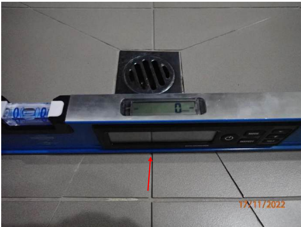
Photograph 38 - Apartment 328B bathroom shower fall within the distance of the level
