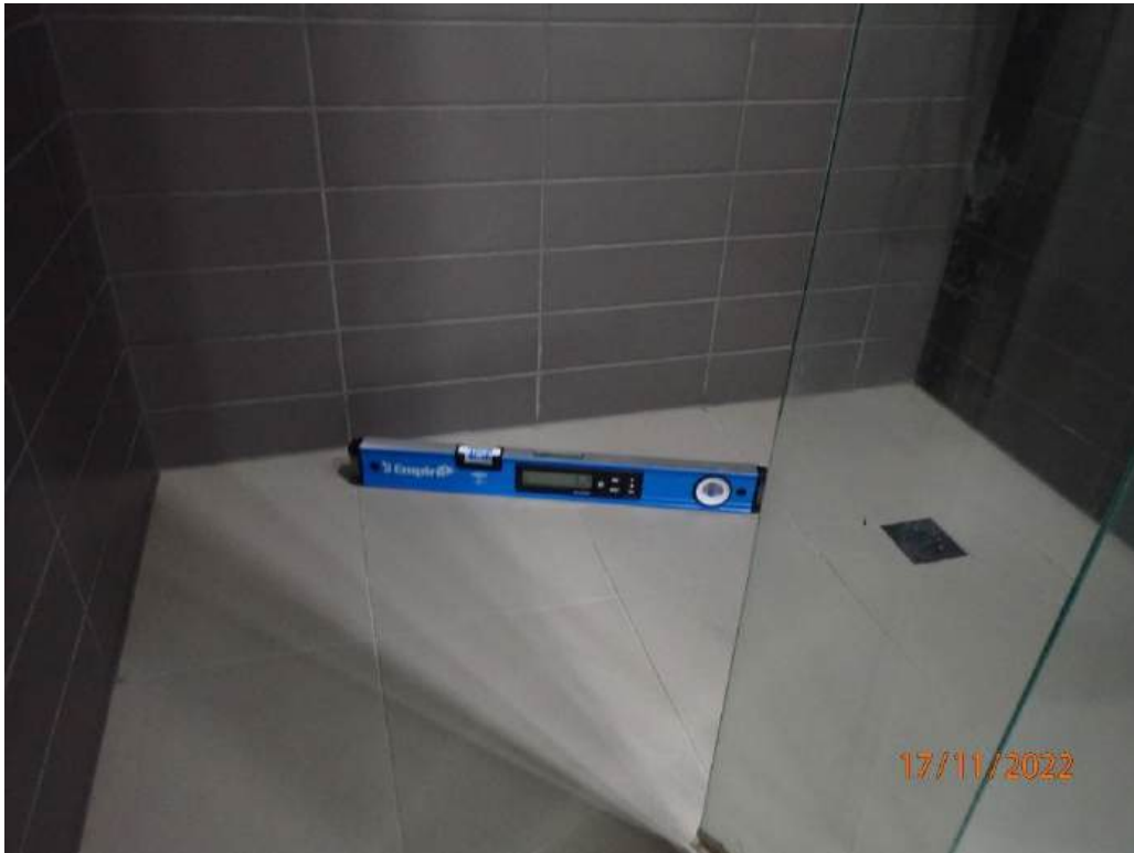
Photograph 35 - Apartment 328B bathroom shower fall
