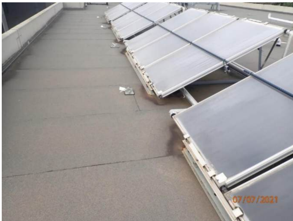
Photograph 128 – Water staining to external edges and around solar panels to building A
