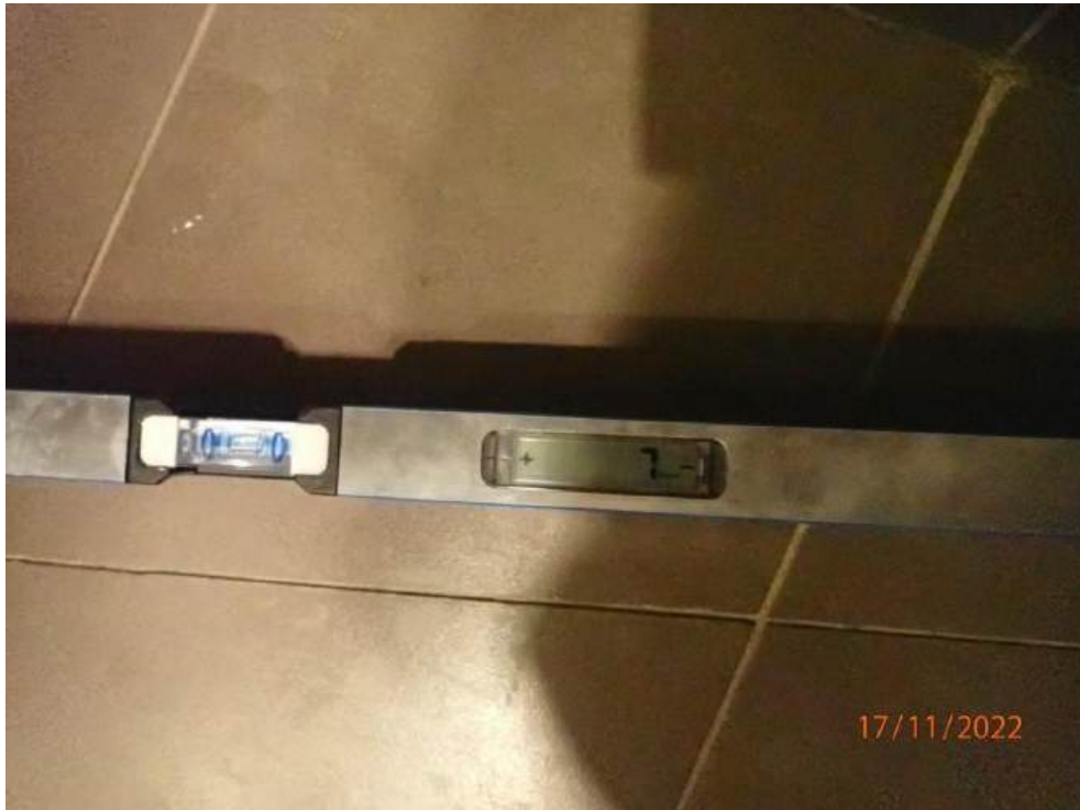
Photograph 7 - Apartment 309A bathroom shower fall 1 in 143
