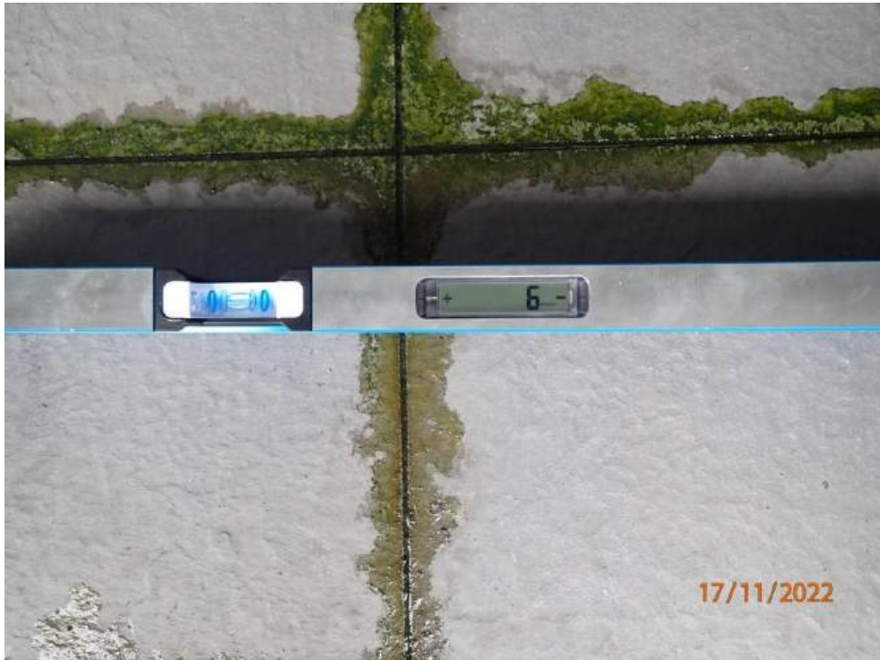
Photograph 17 - Apartment 308A balcony fall 1 in 167
