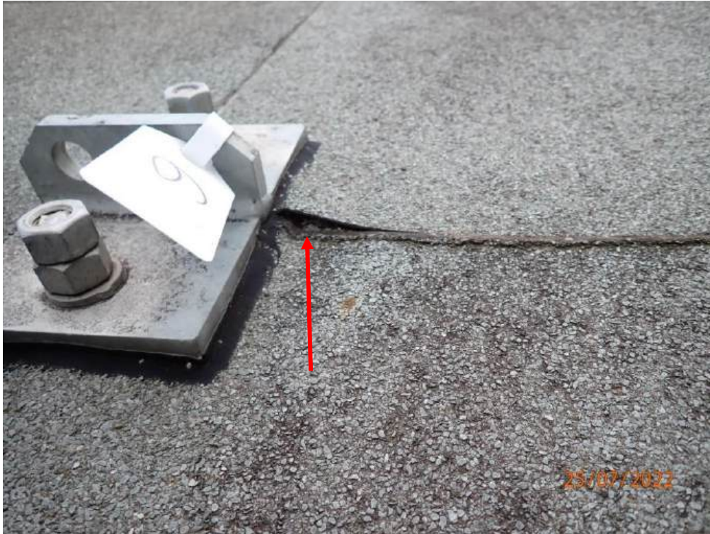
Photograph 171 – Lot 312A/Apartment 312A, rooftop above ceiling hatch, potential area of water ingress
