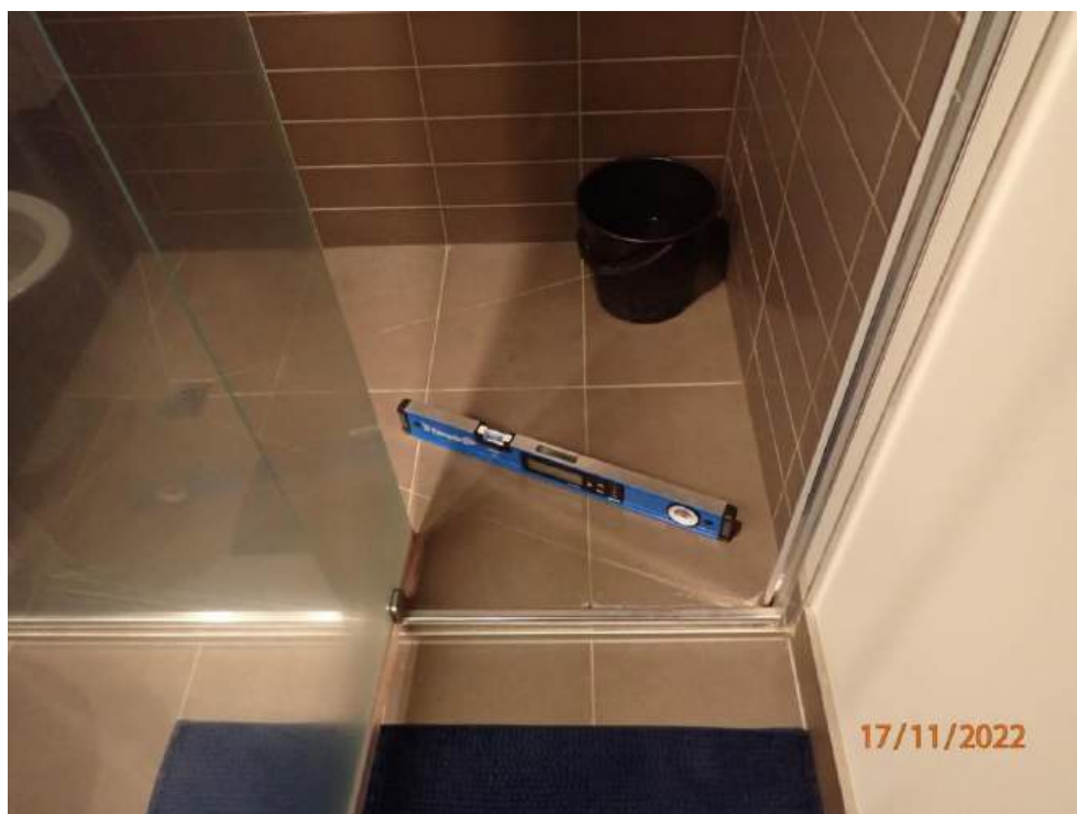
Photograph 2 - Apartment 309A bathroom shower
