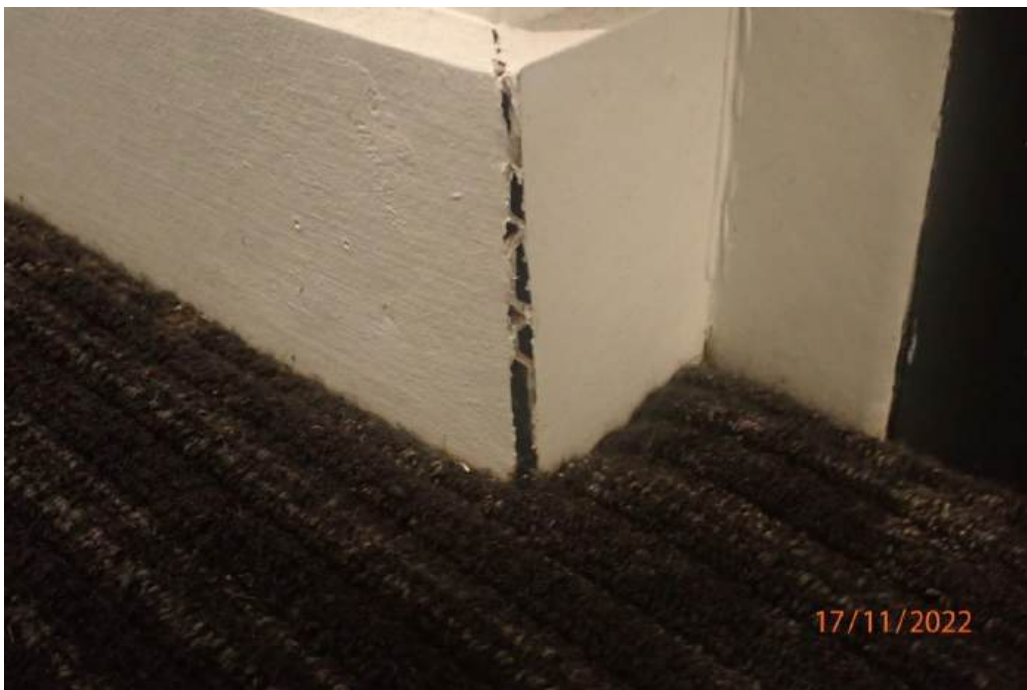
Photograph 120 - Apartment 521B external passageway, skirting trim separation
