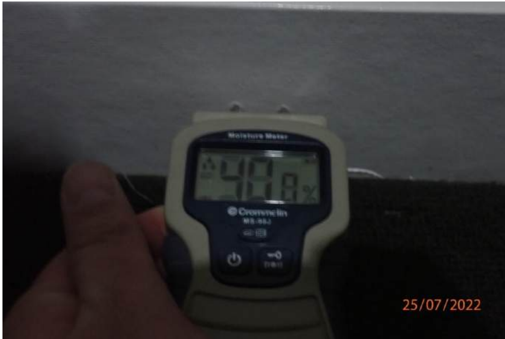
Photograph 145 - Lot 106B/Apartment 116B, west bedroom wall moisture reading
