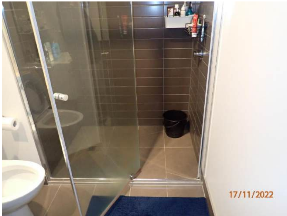
Photograph 1 – Apartment 309A bathroom shower
