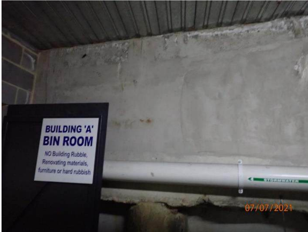
Photograph 1 - Efflorescence and Bondek rusted to southwest corner of bin room
