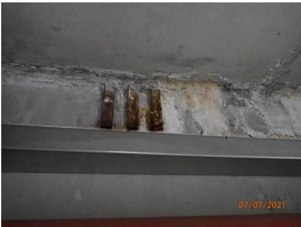
Photograph 24 - Efflorescence, severe calcification build-up and rusty steel components to concrete beams and pipe penetrations near carpark 48 including surrounding carparks
