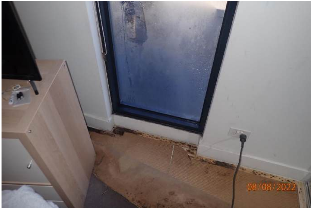
Photograph 203 - 704B/Apartment 703B, west window of the south bedroom, damage to skirting trim
