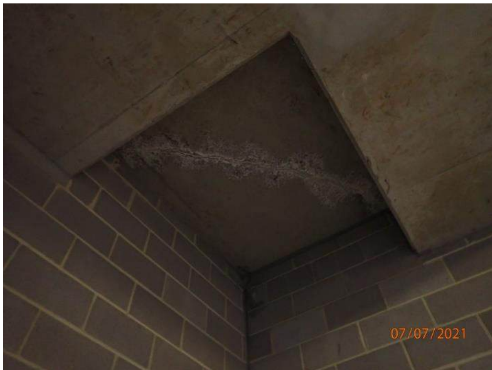
Photograph 10 - Efflorescence and concrete cracked to south elevation above visitor carpark 6
