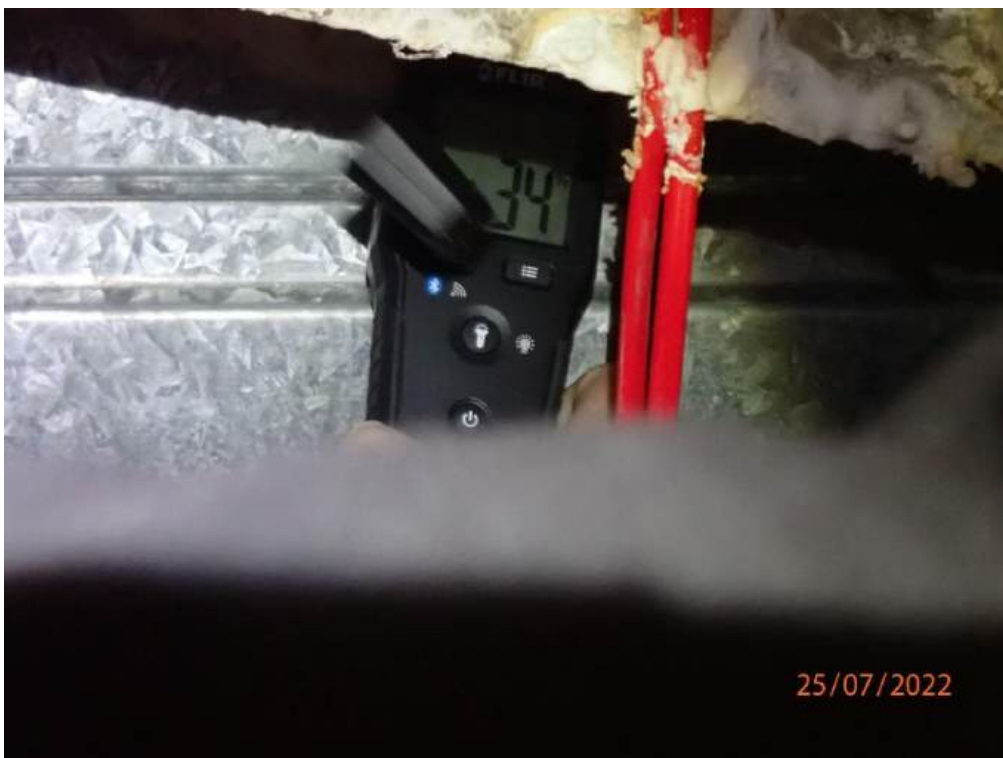
Photograph 170 – Lot 312A/Apartment 312A, concrete roof soffit above ceiling hatch, elevated moisture reading of 34%
