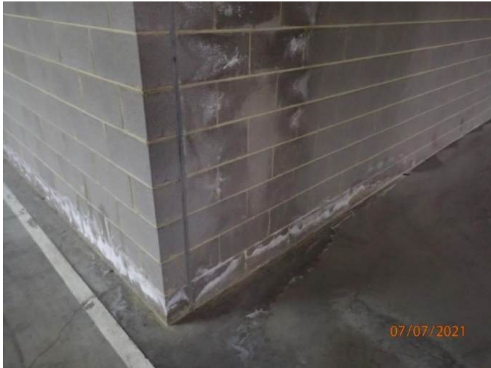
Photograph 87 – Efflorescence to the block walls adjacent the water tanks
