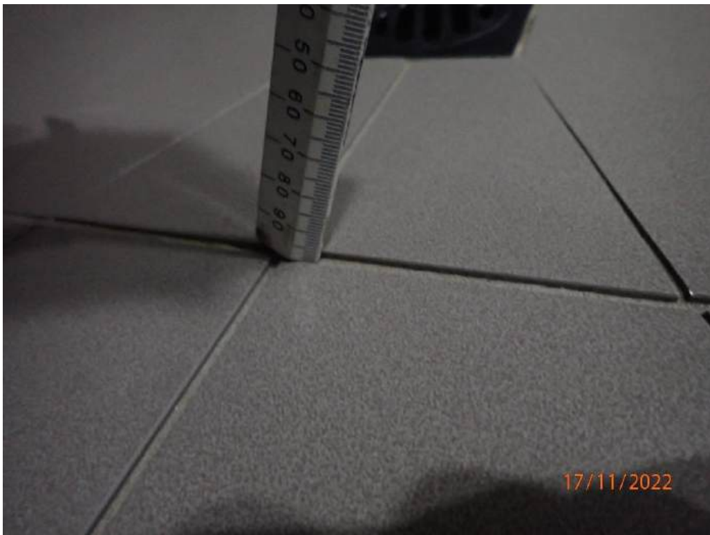
Photograph 40 - Apartment 328B bathroom shower recessed grout lines
