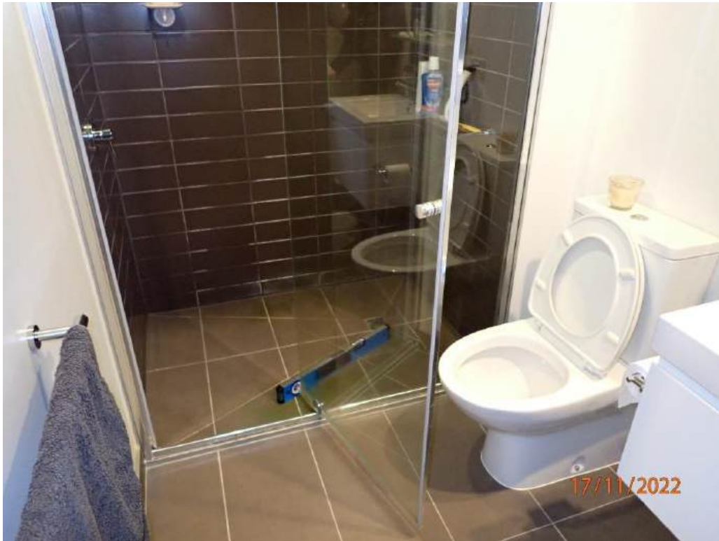
Photograph 29 - Apartment 526B bathroom shower fall
