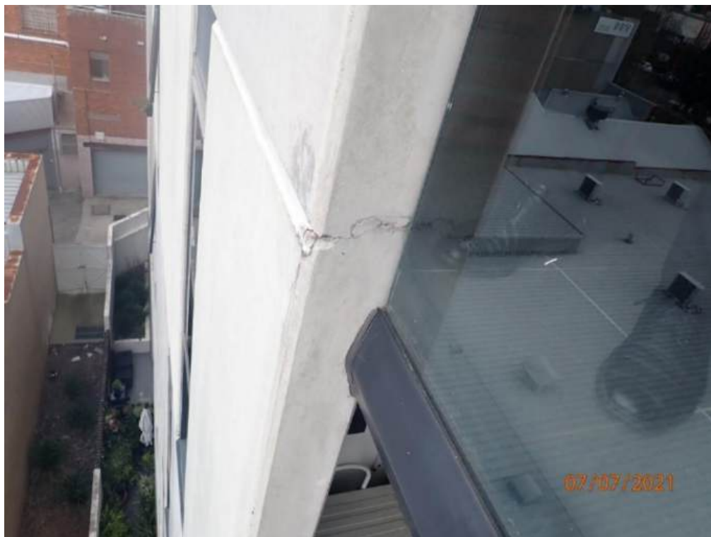
Photograph 98 – Cracking at expansion joints do not extend through the full width of the concrete wall panels to south elevation of building B
