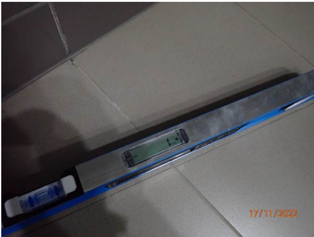
Photograph 36 - Apartment 328B bathroom shower fall 1 in 1,000
