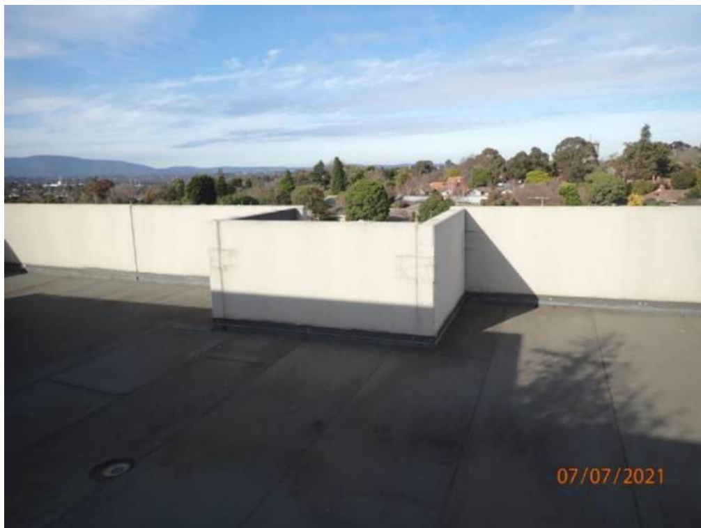
Photograph 112 – Fill is cracking away at tension plates
