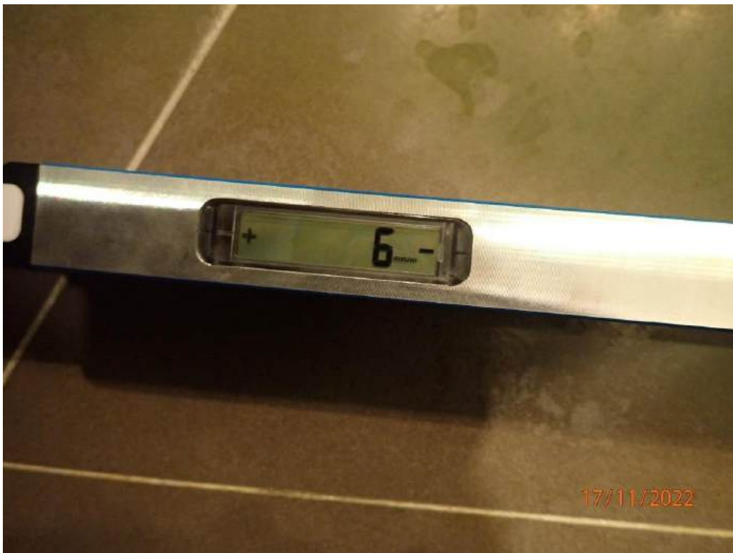
Photograph 30 - Apartment 526B bathroom shower fall 1 in 167
