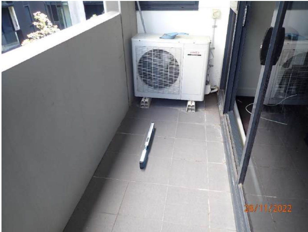
Photograph 89 - Apartment 431B balcony fall
