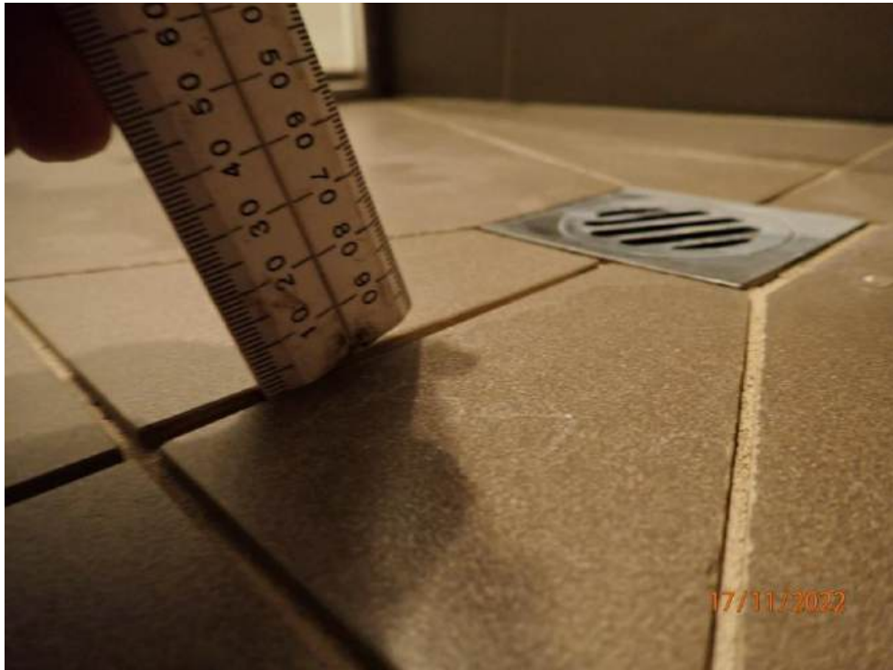
Photograph 9 - Apartment 309A bathroom shower recessed grout lines
