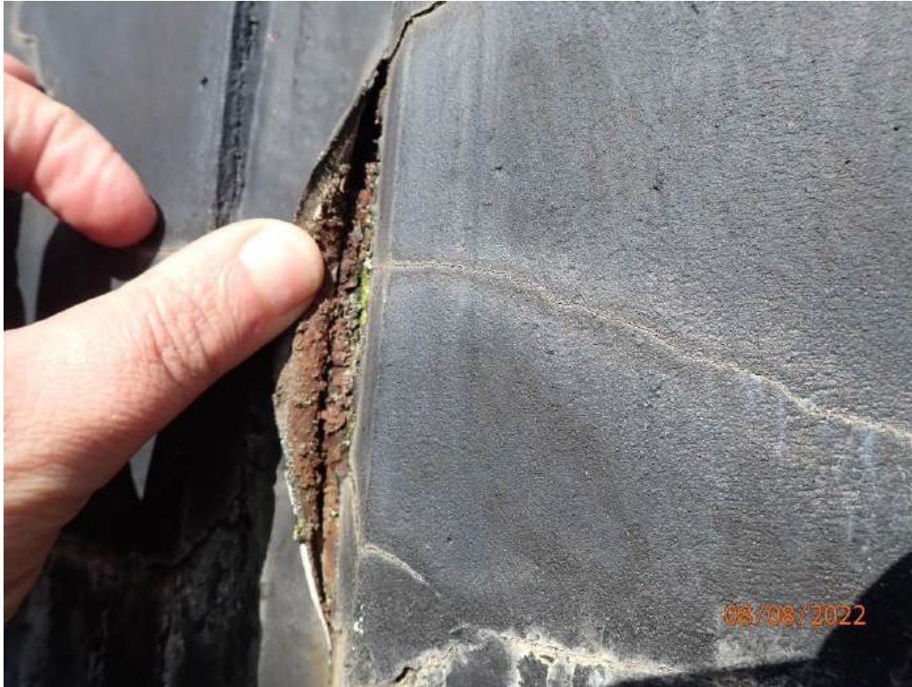
Photograph 141 - Building B facing north west corner of the north stairwell wall at rooftop level, deteriorating patching
