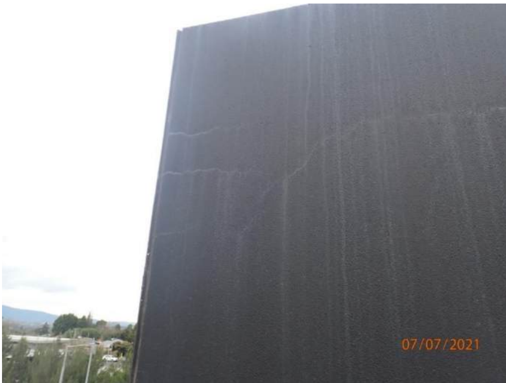
Photograph 104 – Cracking to concrete wall panels to north elevation of building A
