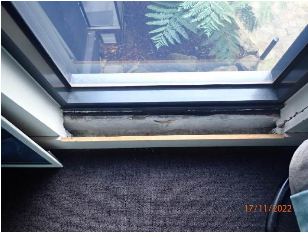
Photograph 49 - Apartment 337B, bedroom 1 window, incomplete repairs to the windowsill reveal and adjacent wall plaster
