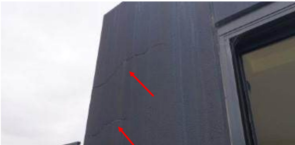
Photograph 220 - Lot 713B/Apartment 712B south wall cracking visible from main balcony. (photo taken on Samsung mobile phone on 25 July 2022 by Peter Kyriakou)
