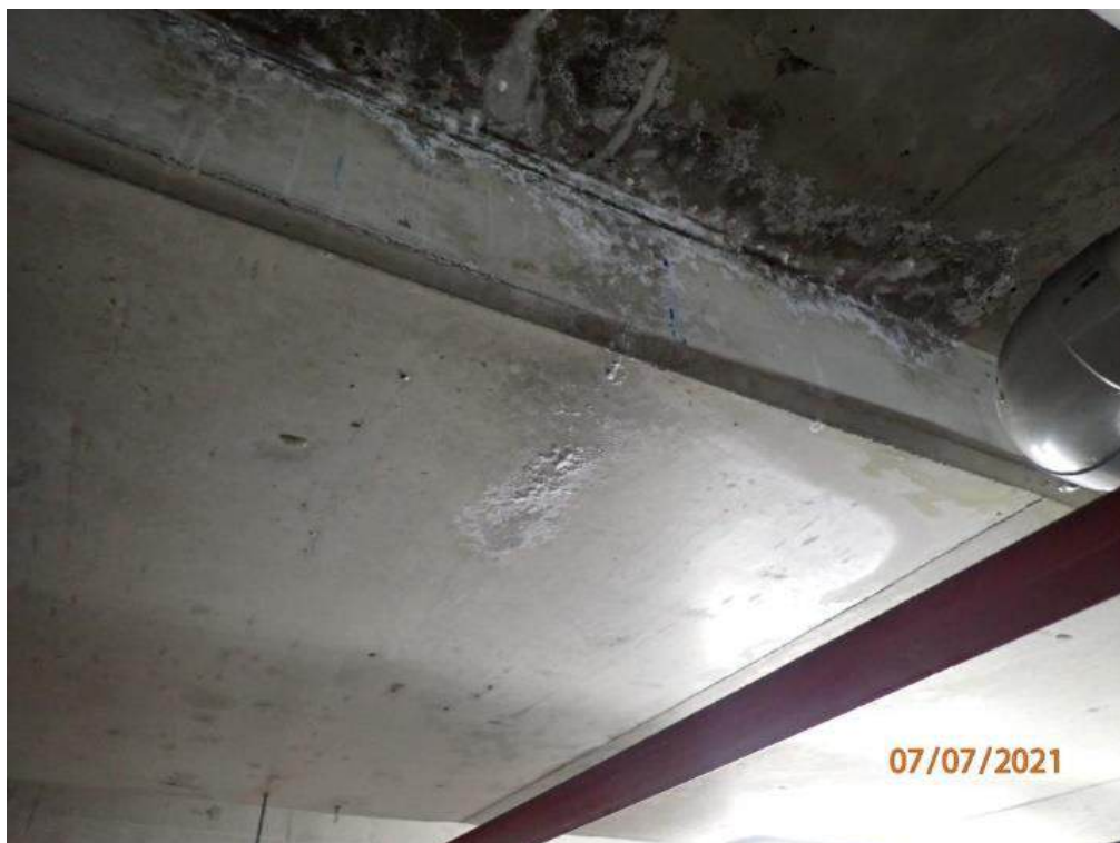
Photograph 42 – Efflorescence and calcium build up
