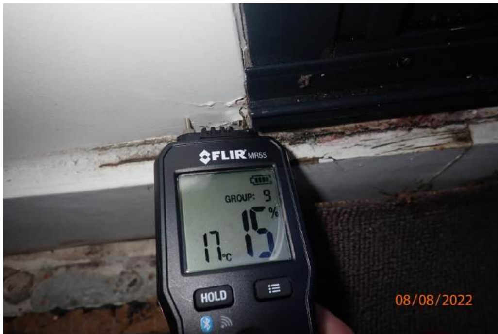
Photograph 212 - 704B/Apartment 703B, living sliding door opening to balcony elevated moisture level of 15% to adjacent plasterboard wall
