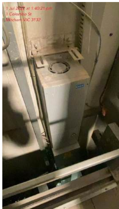
Internal lift shaft, slurry to lift drive
