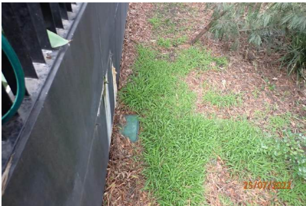
Photograph 148 - Lot 109A/Apartment 109A, planter box overflow outlet
