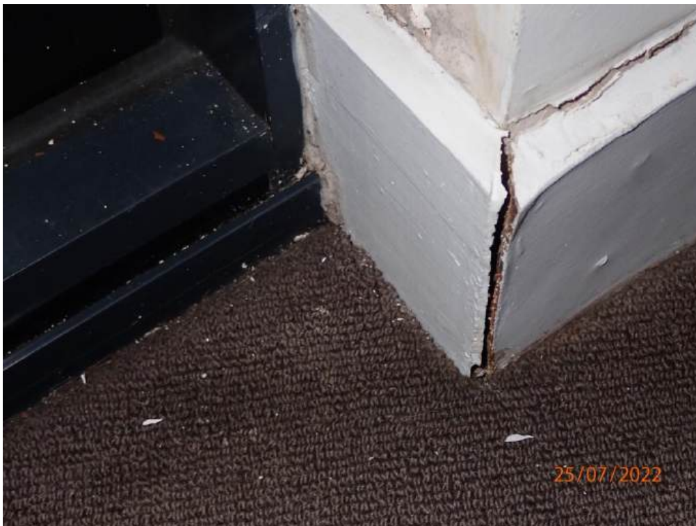
Photograph 158 - Lot 208A/Apartment 208A, bedroom window, moisture damage to skirting trim
