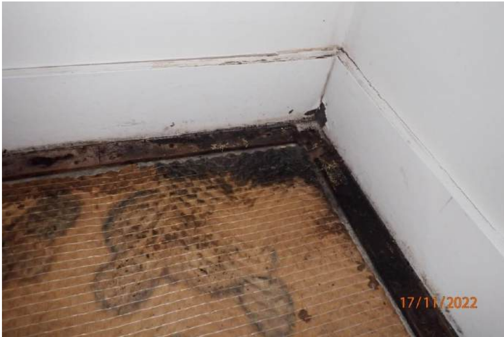
Photograph 115 - Apartment 126B, southeast corner of bedroom 2, water damage and mould growth to carpet and underlay
