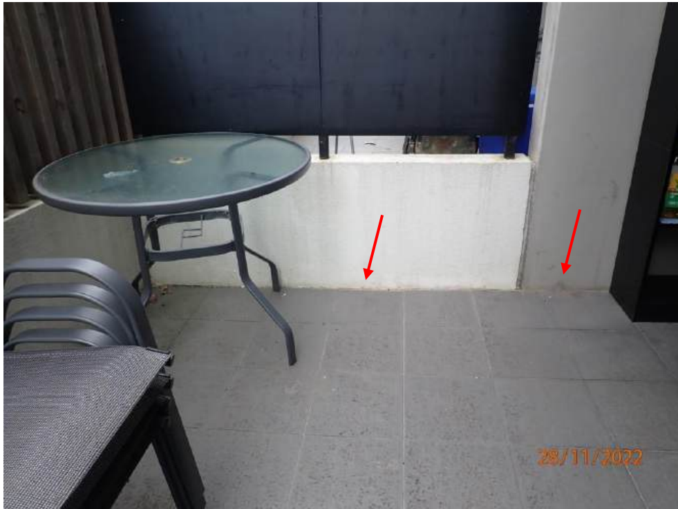
Photograph 103 - Apartment 123B balcony, omission of waterproofing upturns
