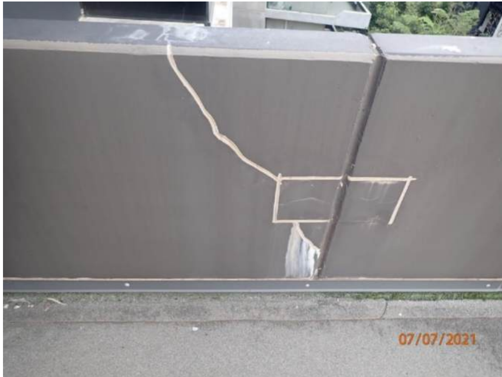
Photograph 109 – Cracking to the concrete wall panels to the north elevation of building A
