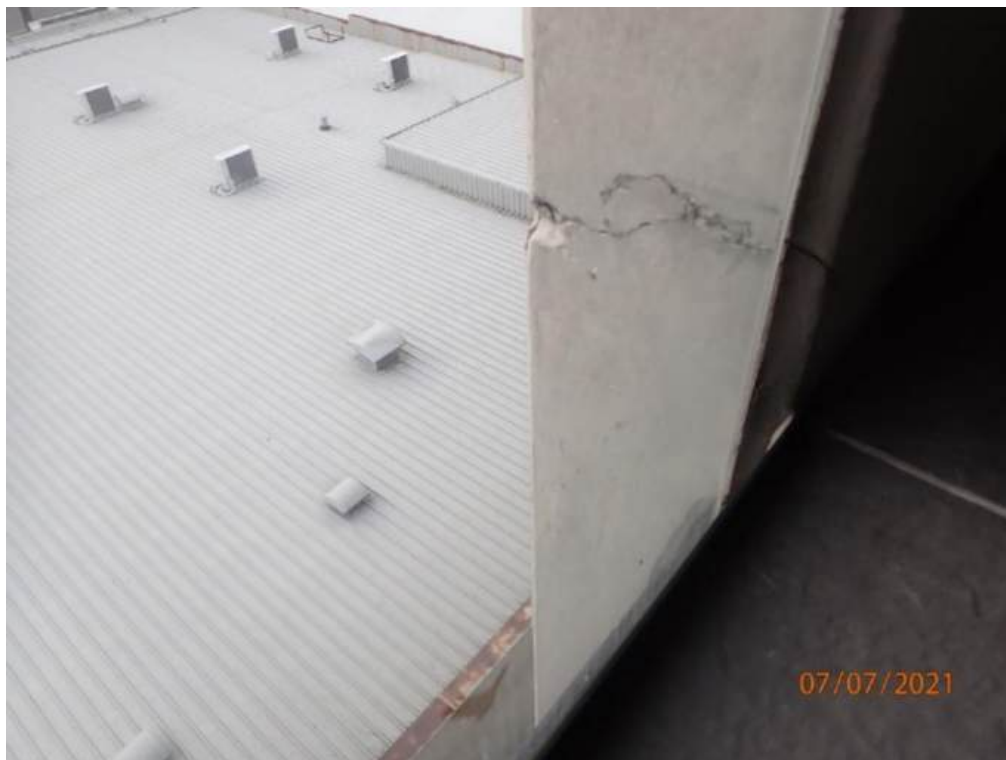
Photograph 100 – Cracking to south elevation of building B
