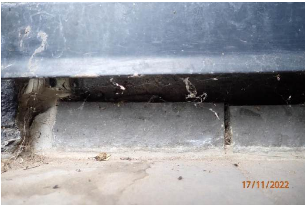
Photograph 108 - Apartment 205A balcony upturn beneath aluminium sliding door and window unit
