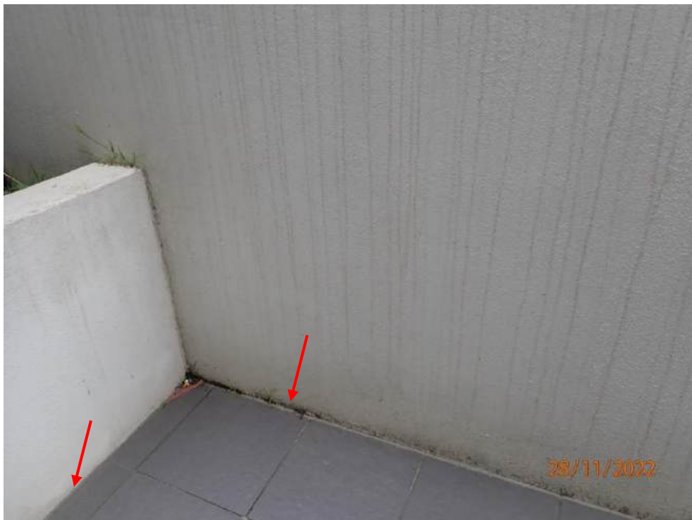
Photograph 102 – Apartment 123B balcony, omission of waterproofing upturns
