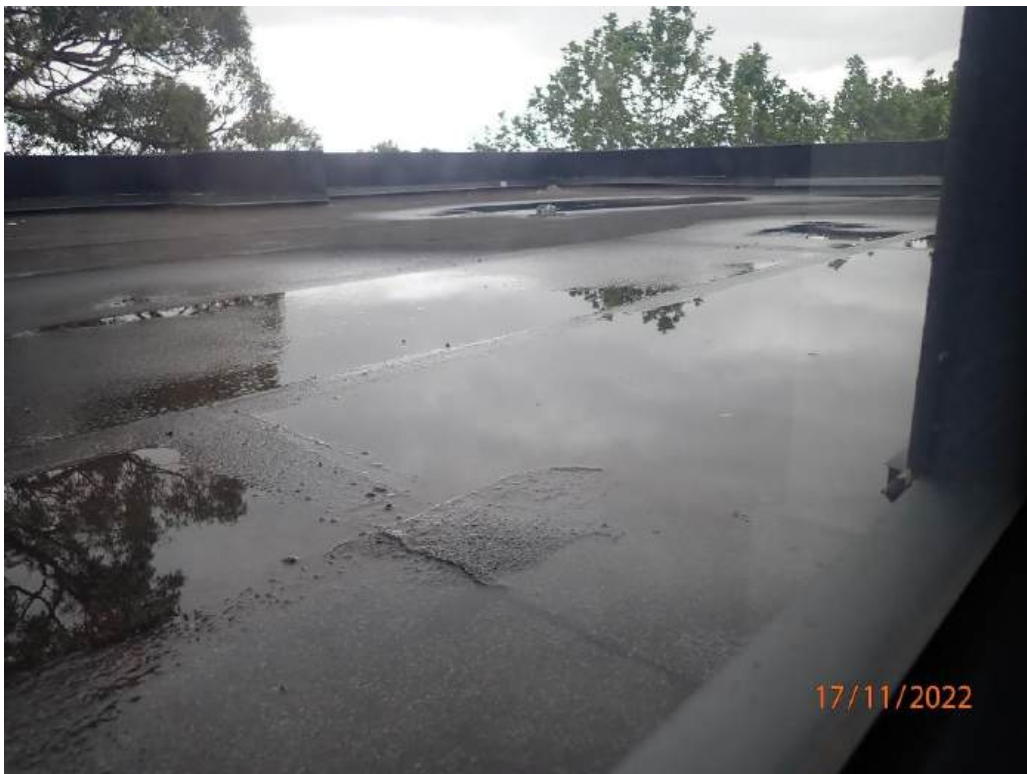
Photograph 52 - Apartment 417B, pooling water on rooftop adjacent to bedroom 2 window
