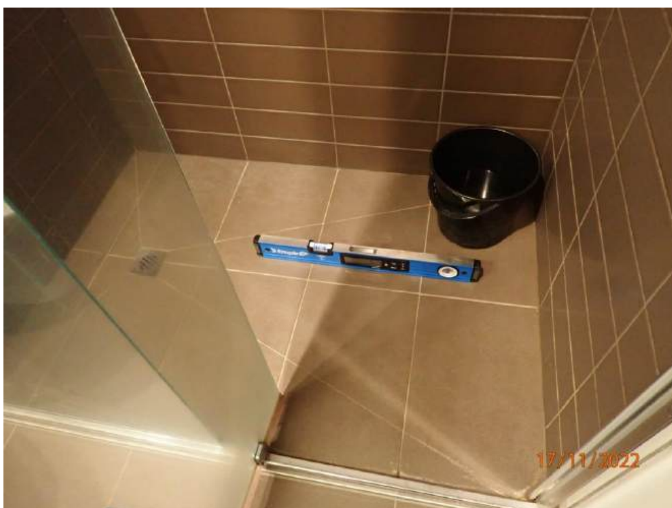
Photograph 4 - Apartment 309A bathroom shower
