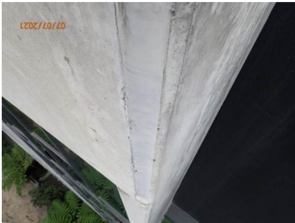
Photograph 118 – Gaps between concrete wall panels exceeding 50 mm to building B
