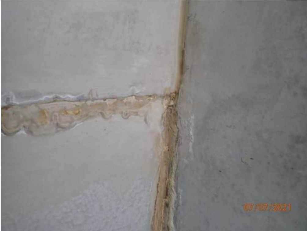
Photograph 79 - Efflorescence, water staining and cracking of concrete to staircase 01 adjacent planter box
