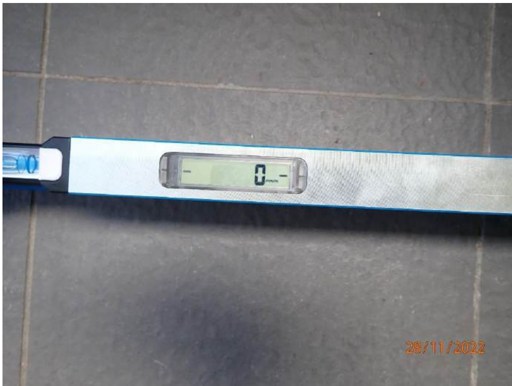
Photograph 90 - Apartment 431B balcony, no fall
