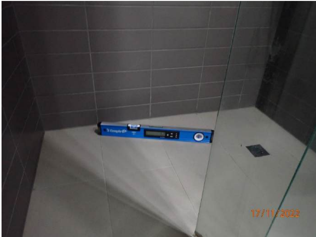
Photograph 35 - Apartment 328B bathroom shower fall
