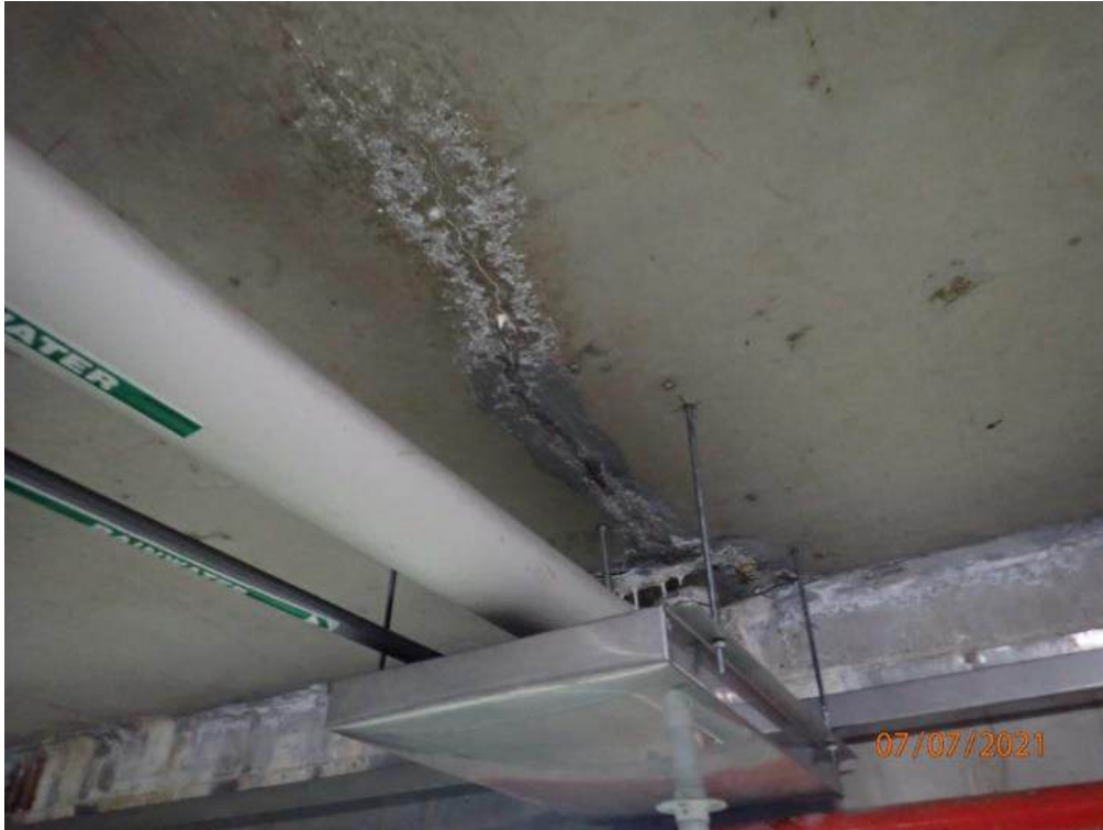
Photograph 27 - Cracks forming in the concrete ceiling near carpark 48 including surrounding carparks
