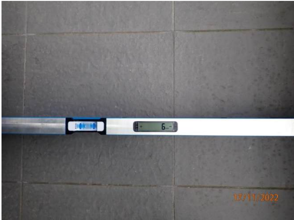
Photograph 15 - Apartment 308A balcony fall 1 in 167
