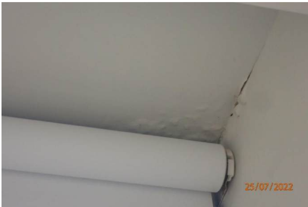
Photograph 162 – Lot 221B/Apartment 231B, northern bedroom, west window reveal paint damage
