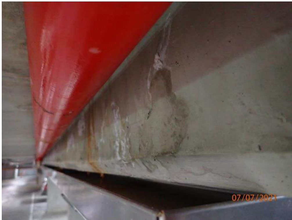
Photograph 48 - Efflorescence and calcium build up
