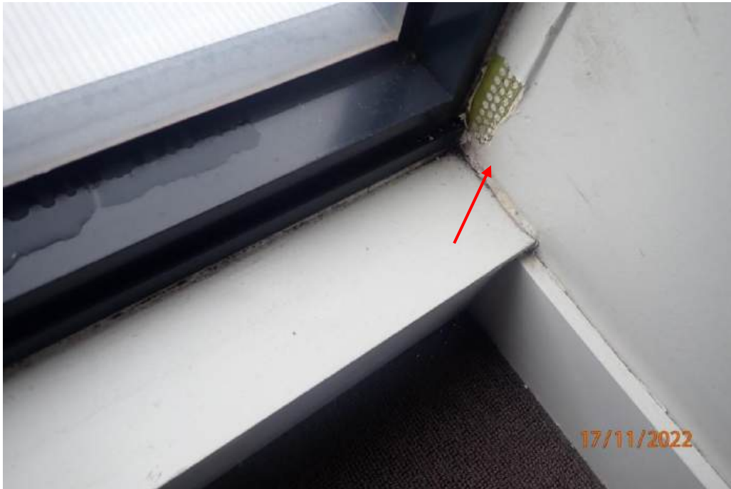
Photograph 125 - Apartment 607B, bedroom window, plaster damage
