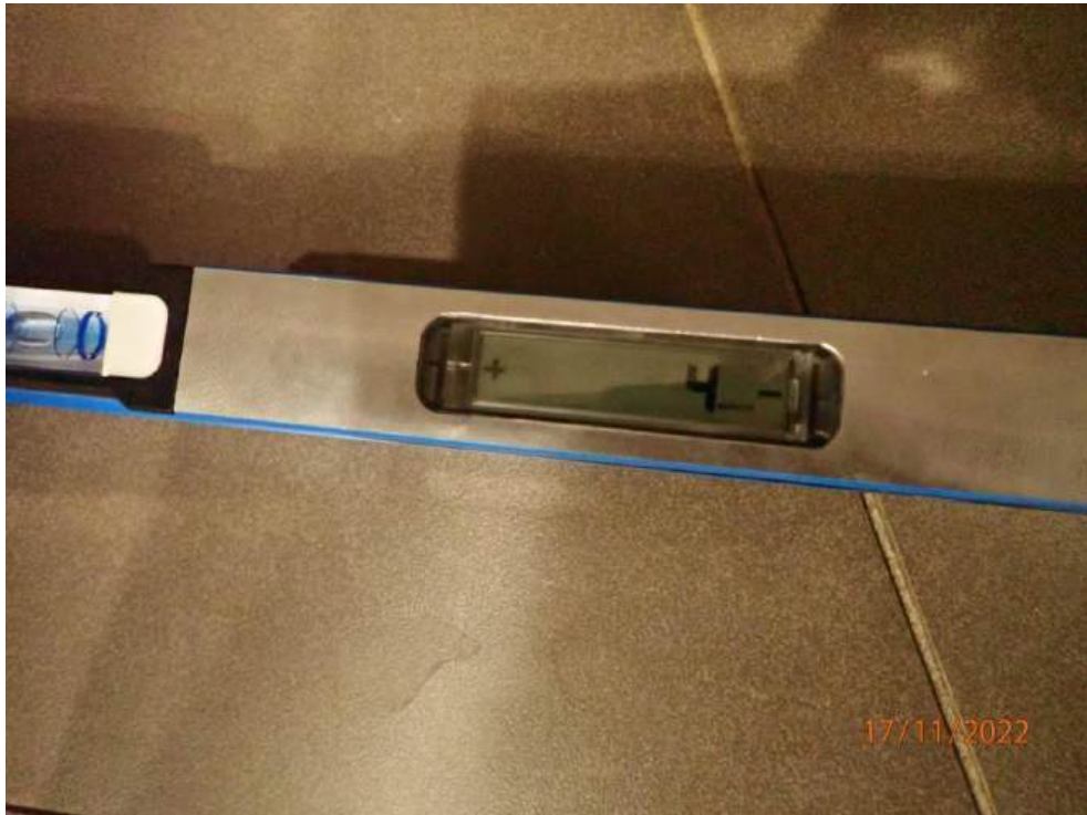
Photograph 3 - Apartment 309A bathroom shower fall 1 in 250
