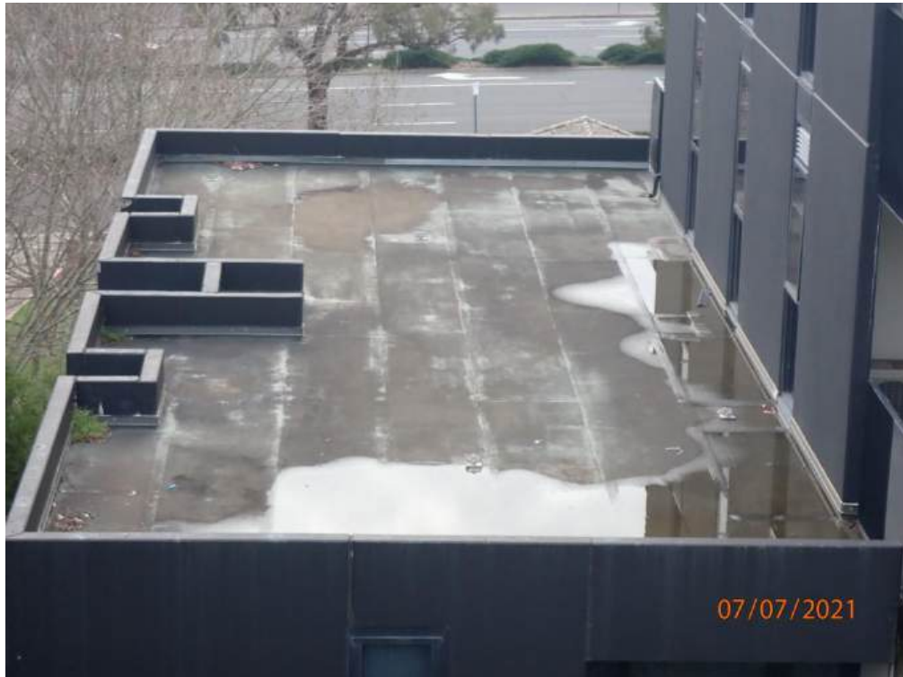
Photograph 125 – Water ponding west elevation of building B
