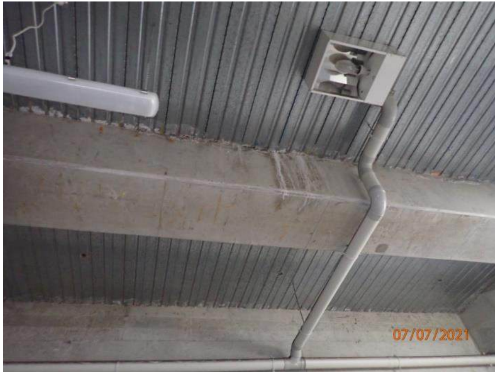
Photograph 65 - Efflorescence and calcium build up to the east end of basement carpark
