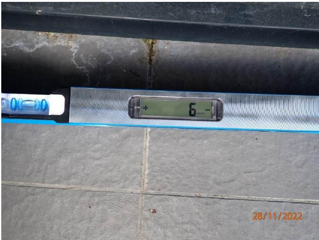
Photograph 92 - Apartment 431B balcony fall 1 in 167
