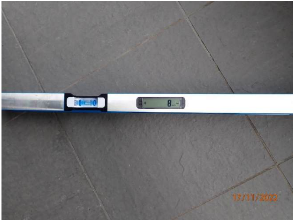
Photograph 13 - Apartment 308A balcony fall 1 in 125
