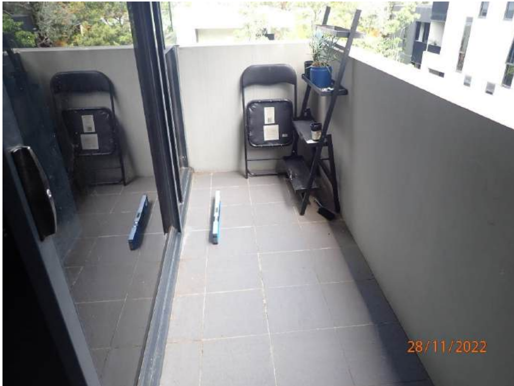
Photograph 93 - Apartment 431B balcony fall
