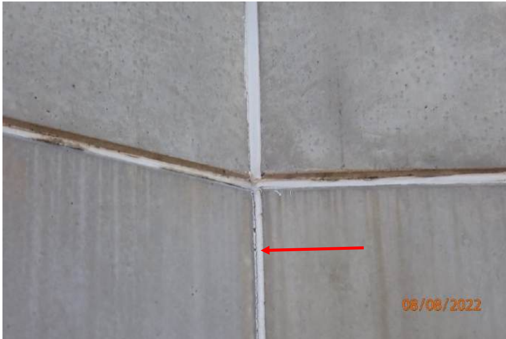
Photograph 189 - Lot 402A/Apartment 402A perished sealant to west elevation wall
