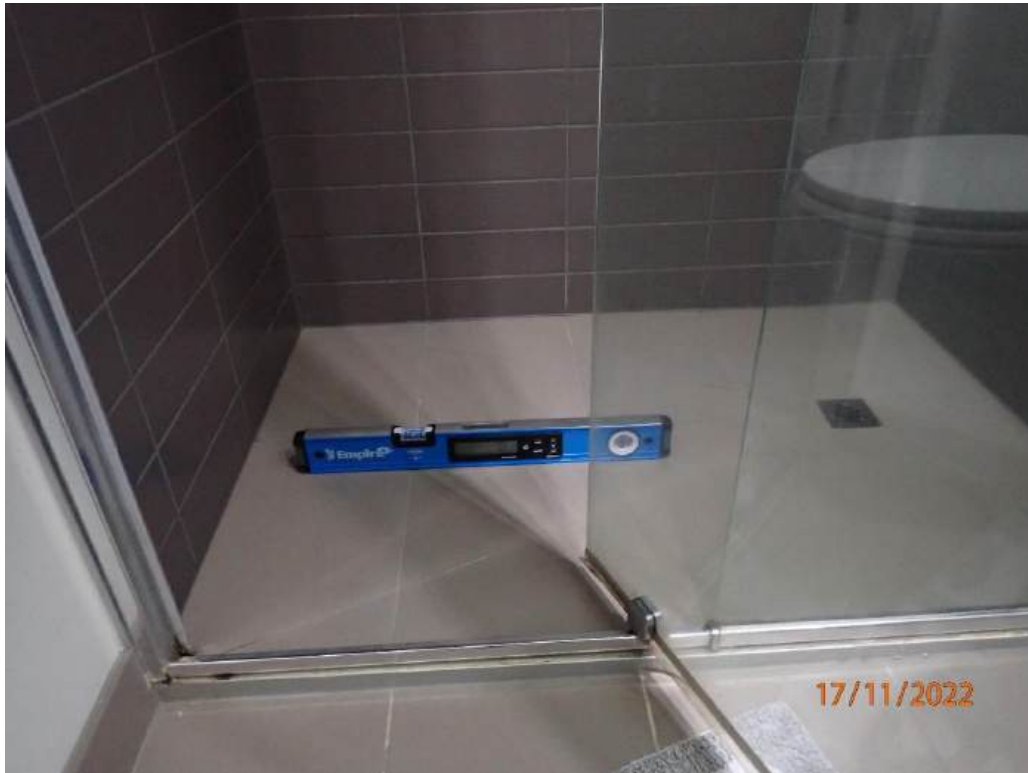
Photograph 33 - Apartment 328B bathroom shower fall
