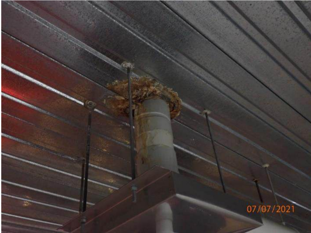
Photograph 35 – Efflorescence and calcification build-up at pipe penetrations
