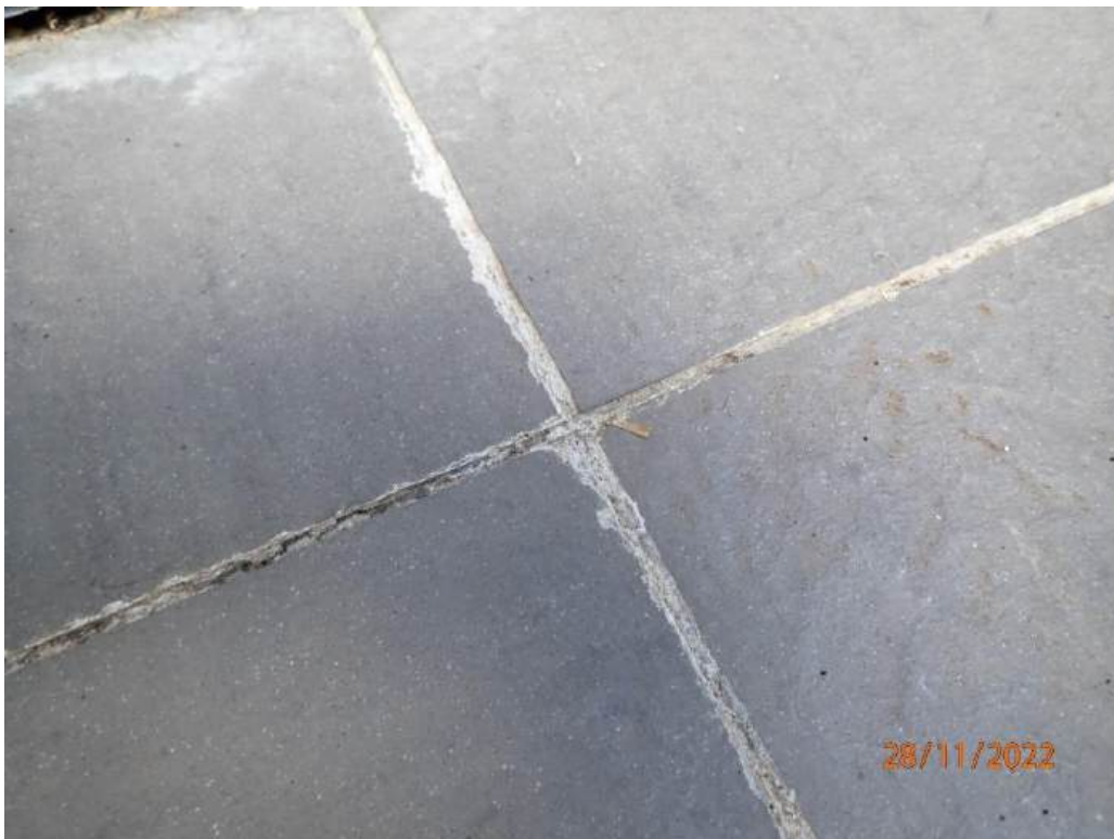
Photograph 98 - Apartment 431B balcony, efflorescence between grout lines
