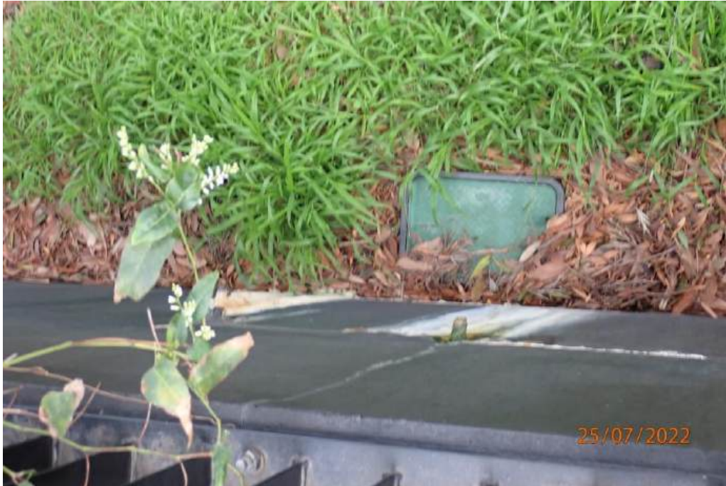
Photograph 149 - Lot 109A/Apartment 109A, planter box overflow outlet
