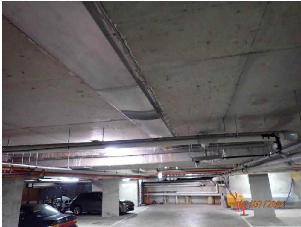
Photograph 38 – Efflorescence visible to either side of metal tray
