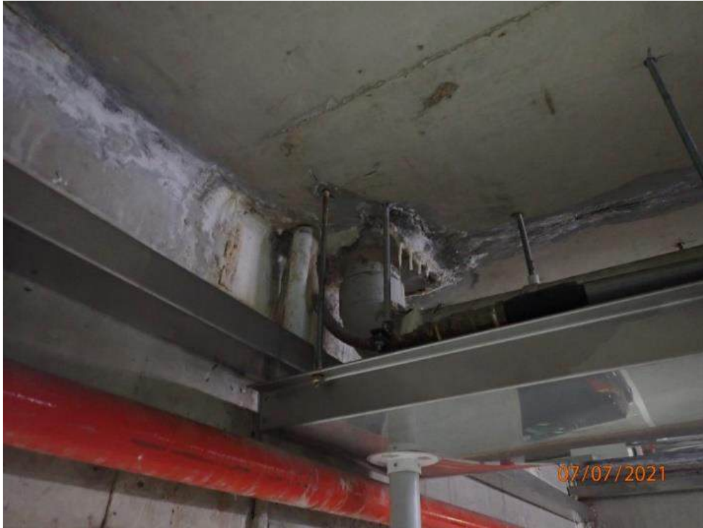
Photograph 25 - Efflorescence, severe calcification build-up and rusty steel components to concrete beams and pipe penetrations near carpark 48 including surrounding carparks
