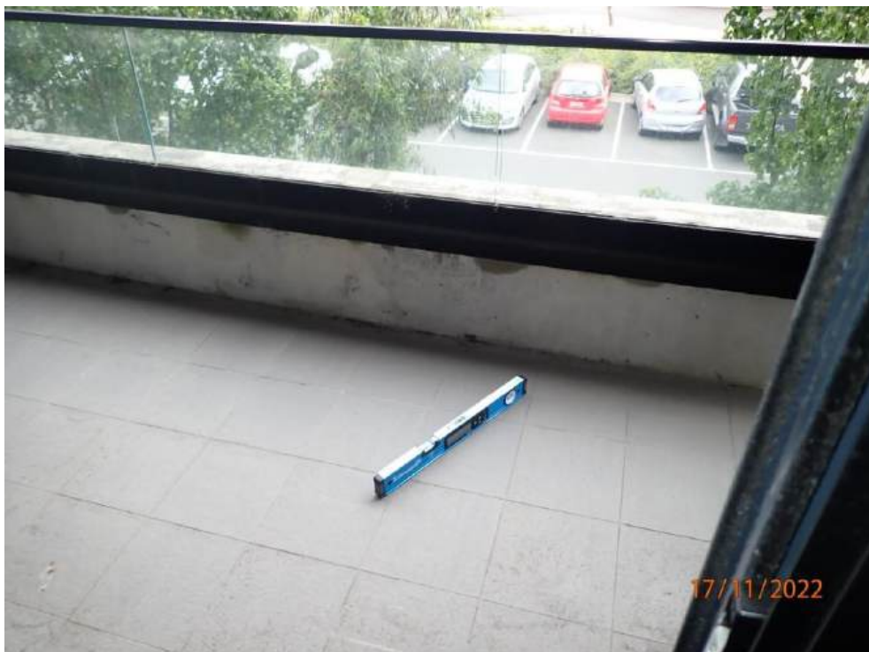
Photograph 12 - Apartment 308A balcony fall
