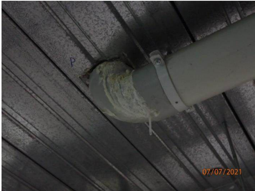
Photograph 15 - Calcification at PVC pipe penetration above carpark 65
