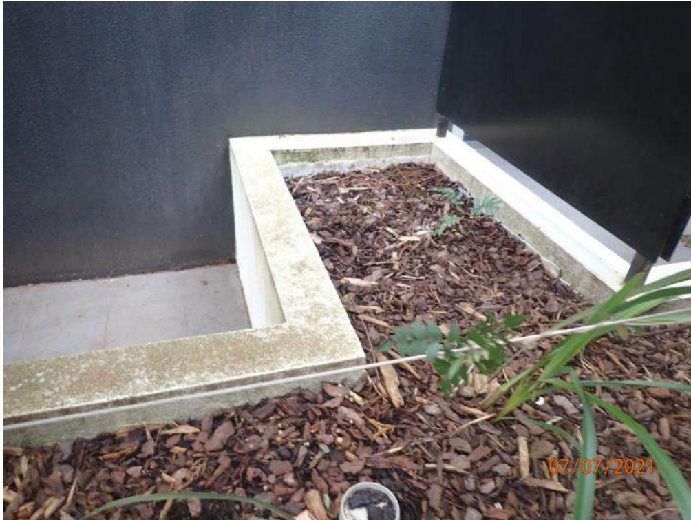
Photograph 75 - Over flashings and capping flashings are not installed to the planter boxes
