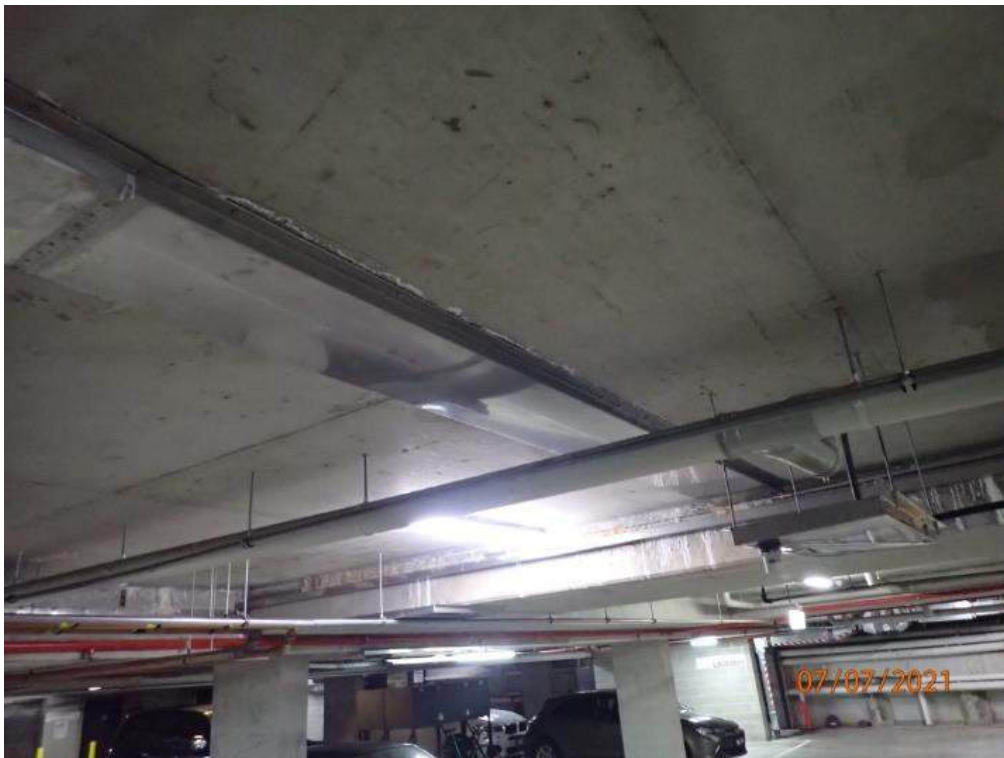
Photograph 36 – Metal tray extends through centre of basement carpark
