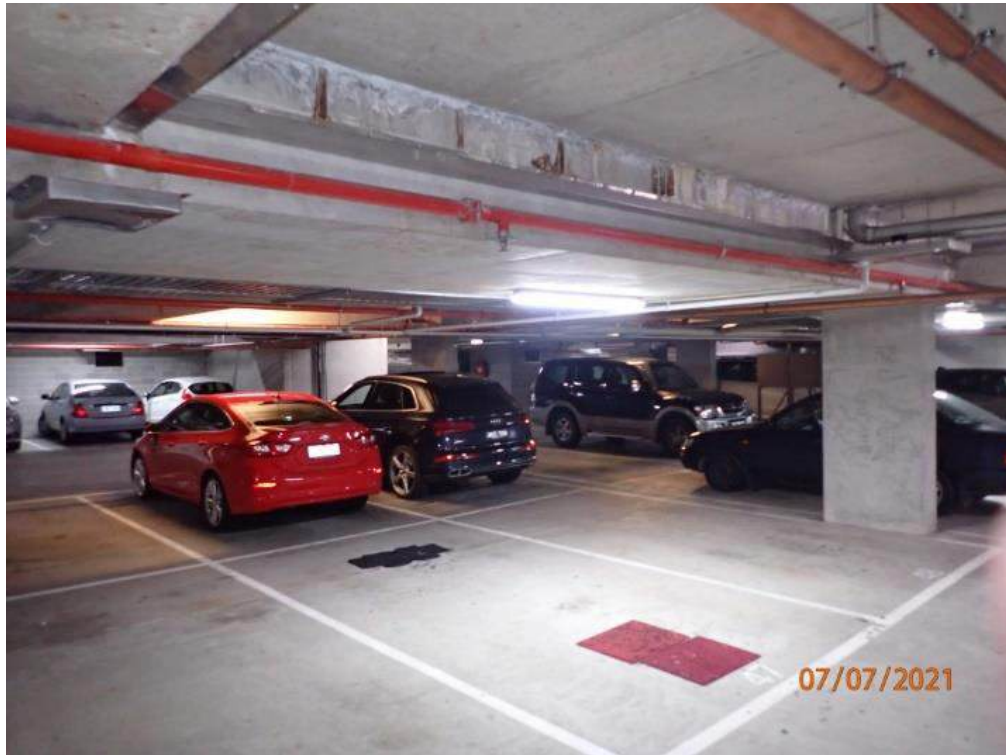
Photograph 21 - Efflorescence, severe calcification build-up and rusty steel components to concrete beams and pipe penetrations near carpark 48 including surrounding carparks
