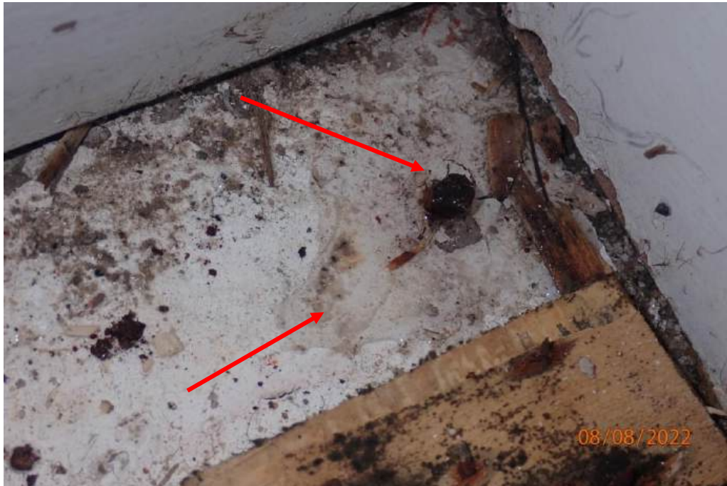
Photograph 209 - 704B/Apartment 703B, west window of the south bedroom, water ingress from water testing
