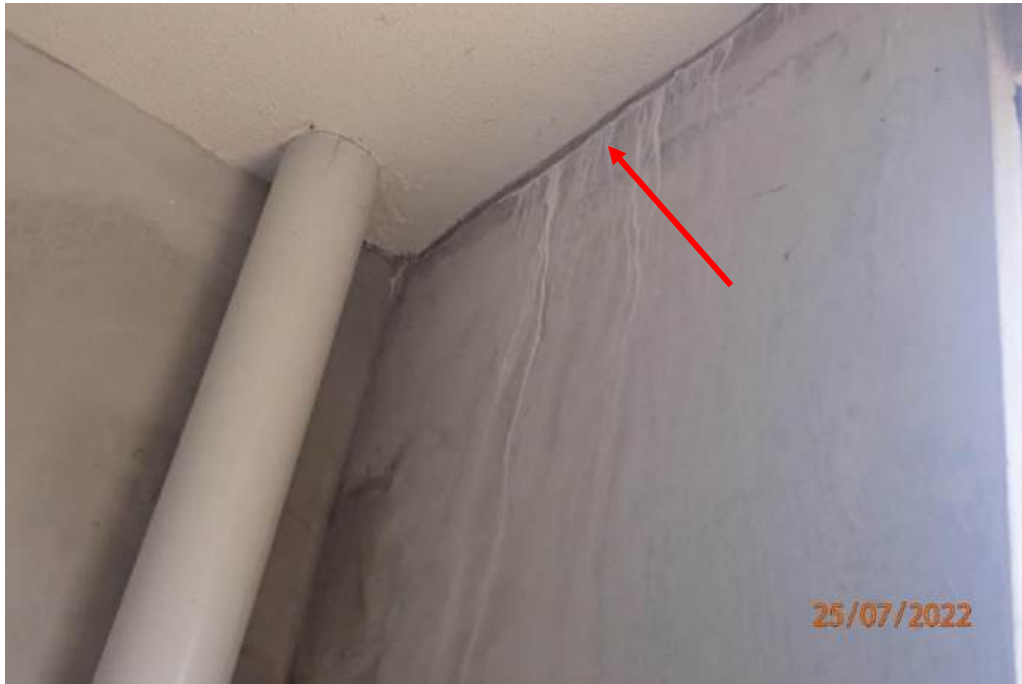
Photograph 191 - Lot 418B/Apartment 428B, north east balcony soffit, efflorescence visible from Lot 321B/Apartment 333B
