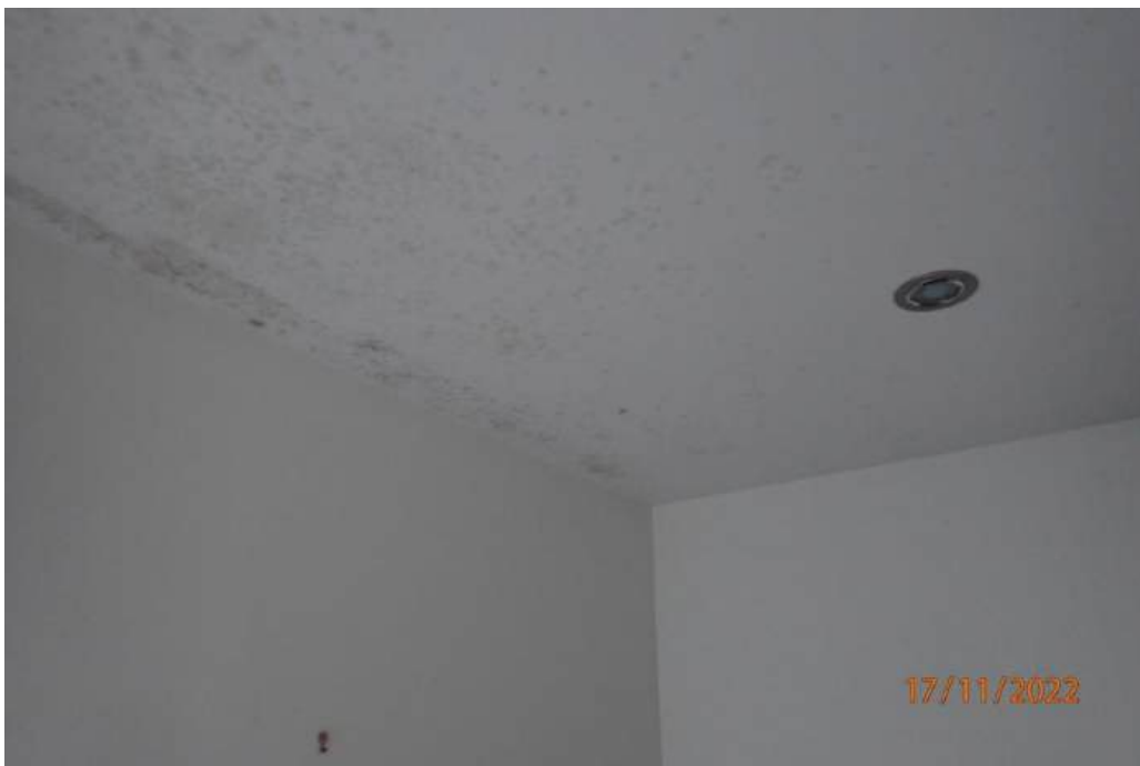
Photograph 134 - Apartment 510A, bedroom ceiling, mould growth in view
