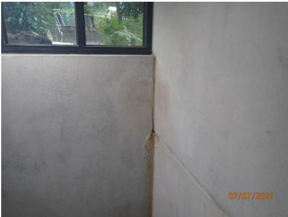
Photograph 80 - Efflorescence, water staining and cracking of concrete to staircase 01 adjacent planter box
