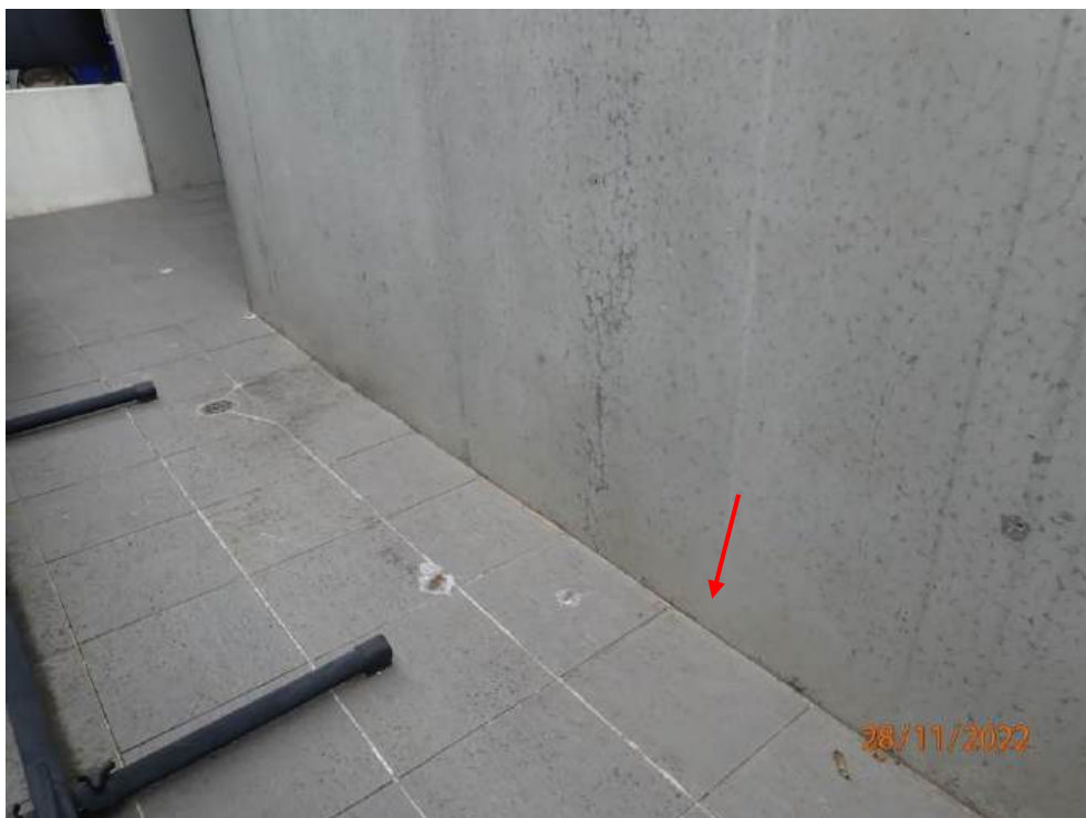
Photograph 104 - Apartment 123B balcony, omission of waterproofing upturns
