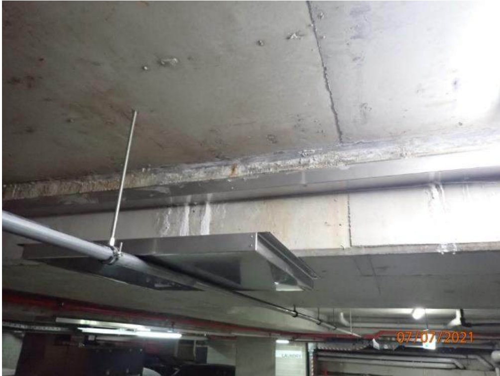
Photograph 29 - Efflorescence, severe calcification build-up and rusty steel components to concrete beams and pipe penetrations near carpark 48 including surrounding carparks
