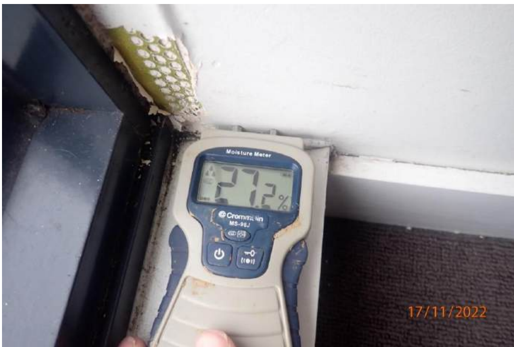
Photograph 126 - Apartment 607B, bedroom window, elevated moisture levels in wall plaster
