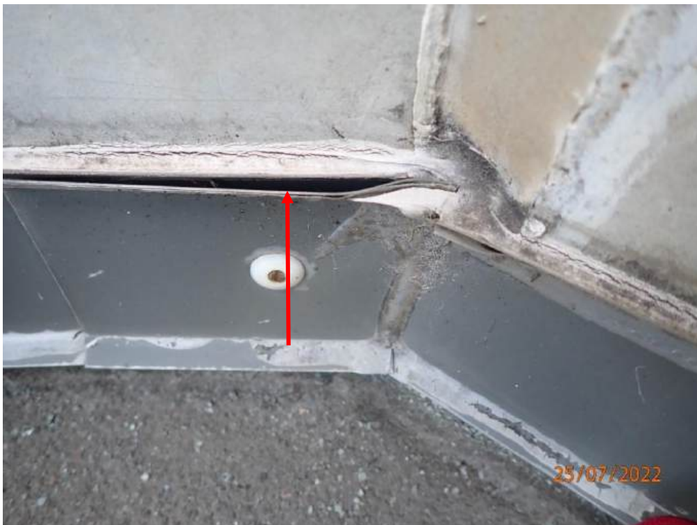
Photograph 172 – Lot 312A/Apartment 312A, rooftop above ceiling hatch, potential area of water ingress
