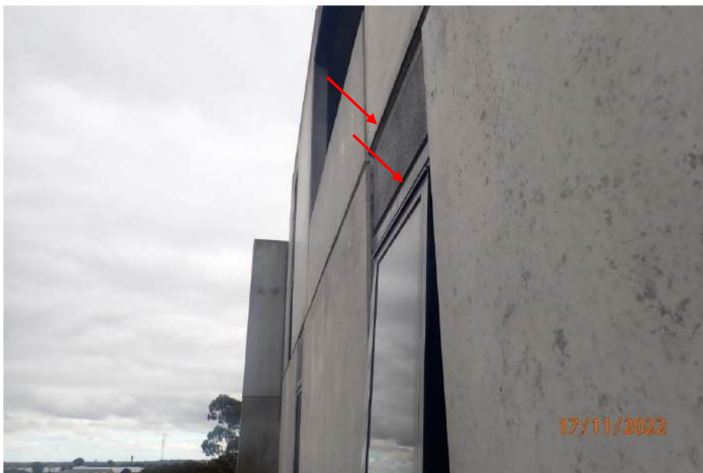
Photograph 132 - Apartment 607B, bedroom window, external view, likely entry points of water ingress
