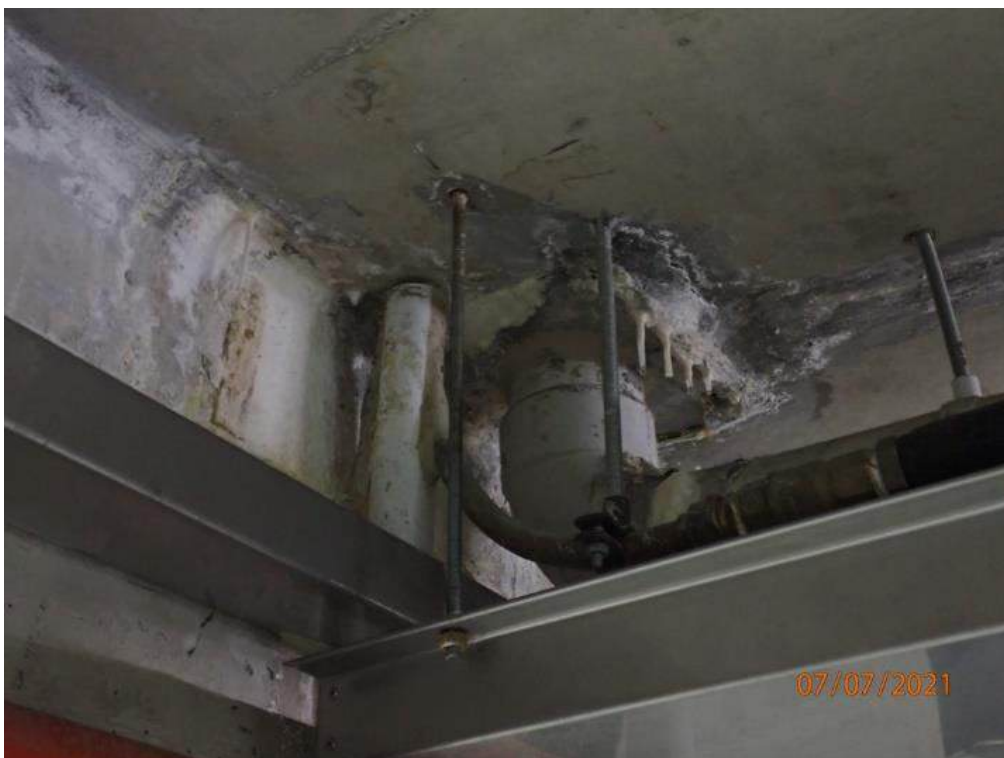
Photograph 26 - Efflorescence, severe calcification build-up and rusty steel components to concrete beams and pipe penetrations near carpark 48 including surrounding carparks
