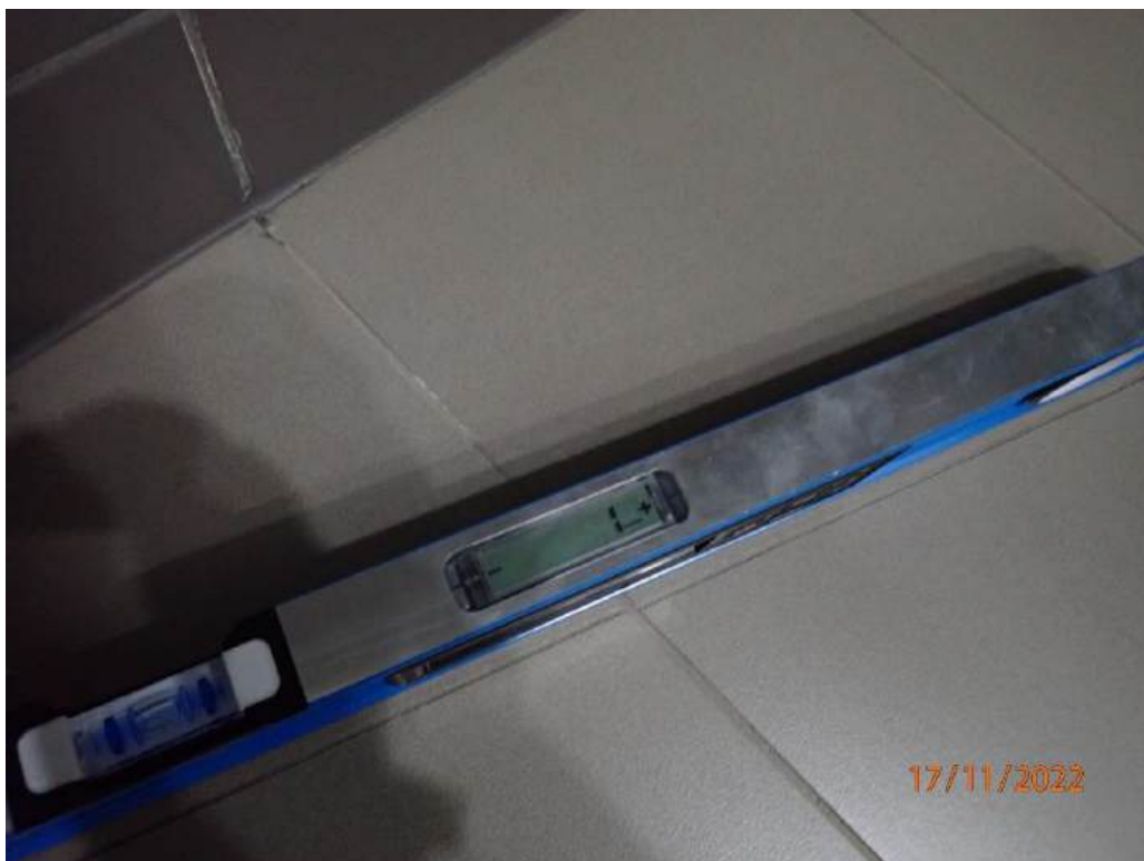
Photograph 36 - Apartment 328B bathroom shower fall 1 in 1,000
