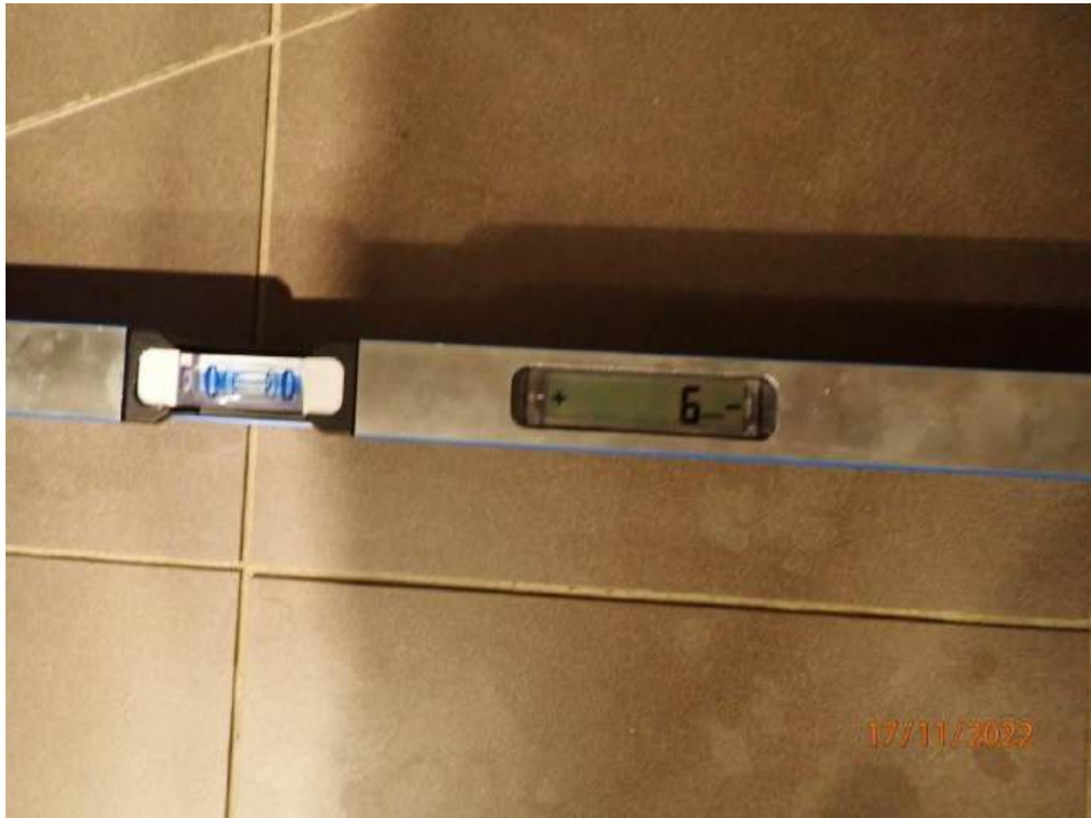
Photograph 5 - Apartment 309A bathroom shower fall 1 in 167
