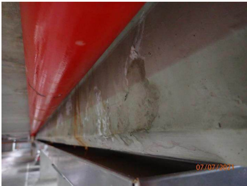
Photograph 48 - Efflorescence and calcium build up
