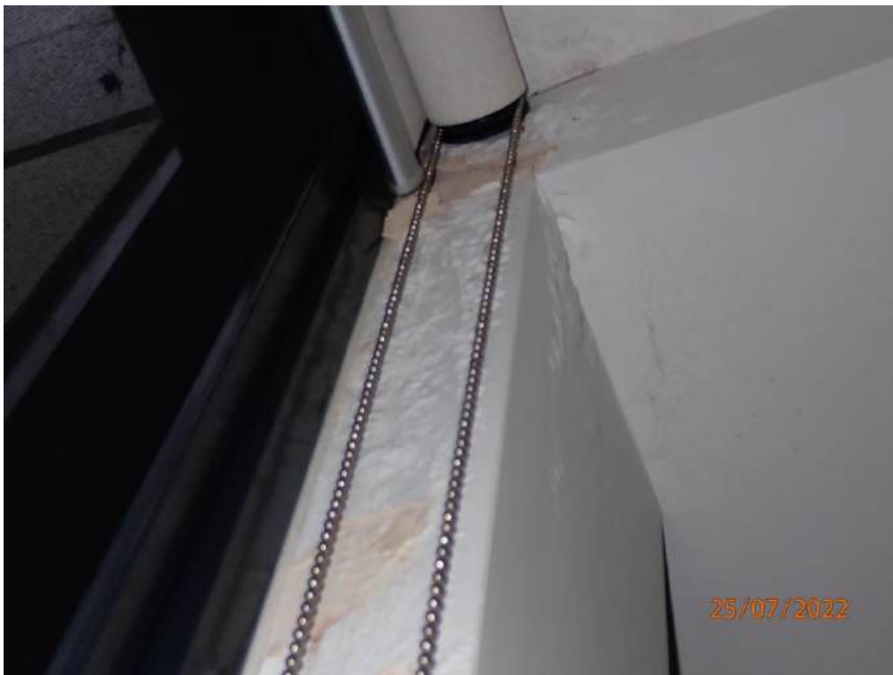
Photograph 160 – Lot 208A/Apartment 208A, bedroom window, moisture damage to window reveal and adjacent wall and ceiling
