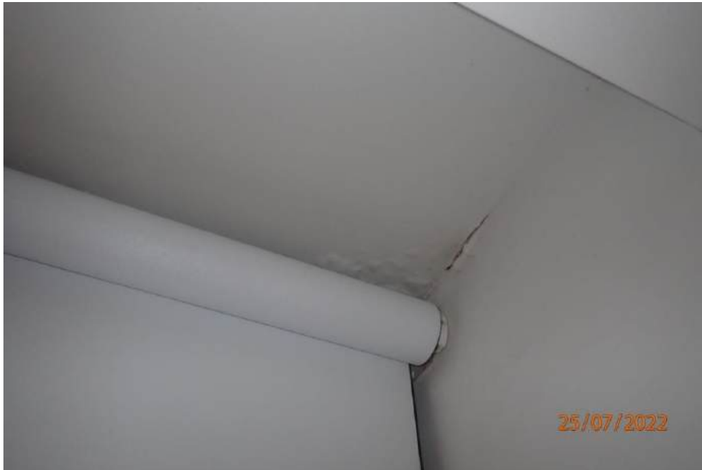
Photograph 161 – Lot 221B/Apartment 231B, northern bedroom, west window reveal paint damage
