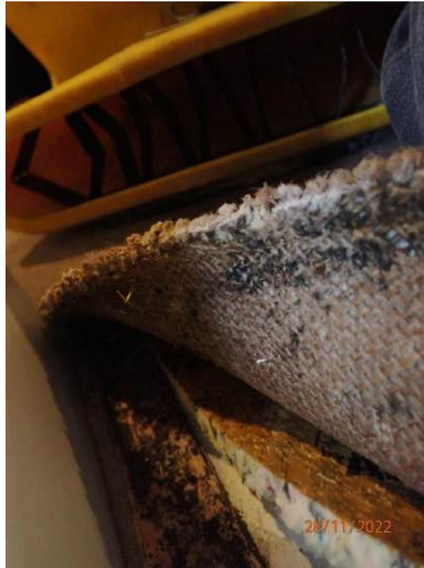
Photograph 69 - Apartment 109A bedroom 2 initial moisture damage to underside of carpet
