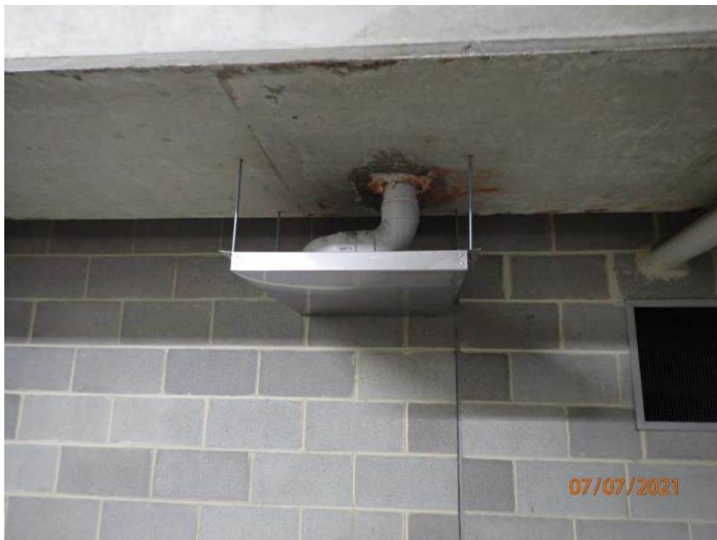
Photograph 8 - Builder installed tray below PVC pipe above carpark 68
