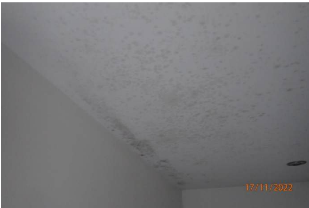
Photograph 136 - Apartment 510A, bedroom ceiling, mould growth in view
