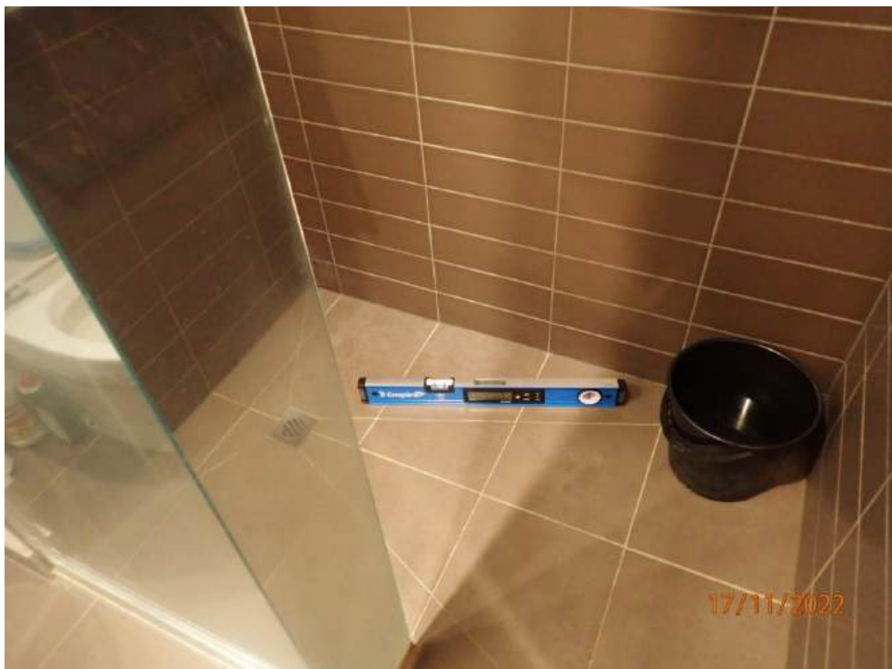
Photograph 6 - Apartment 309A bathroom shower
