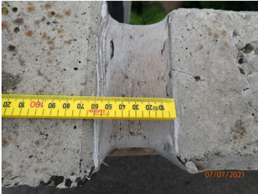
Photograph 117 – Gaps between concrete wall panels exceeding 50 mm to building B
