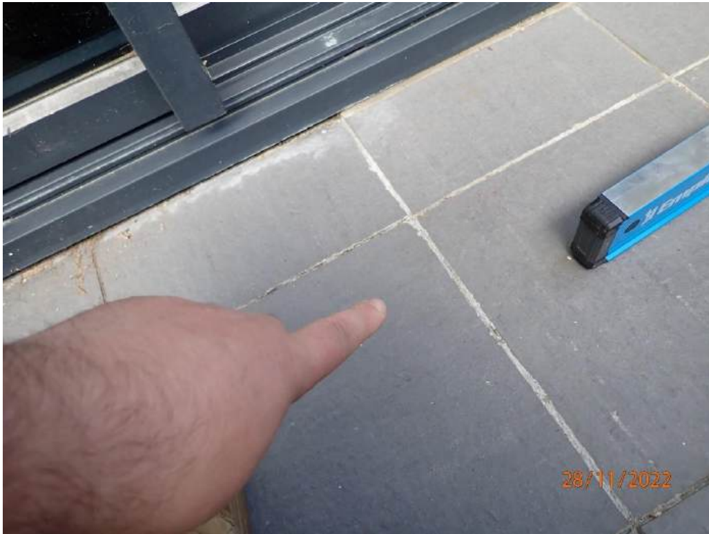
Photograph 97 - Apartment 431B balcony, efflorescence between grout lines
