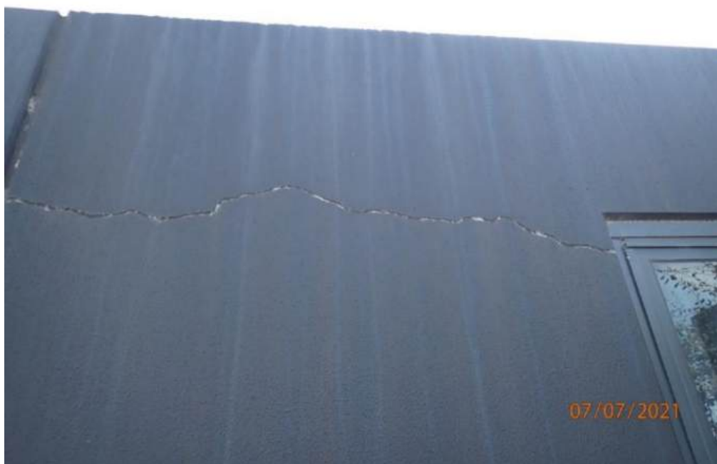
Photograph 96 – Cracking to west elevation of building B
