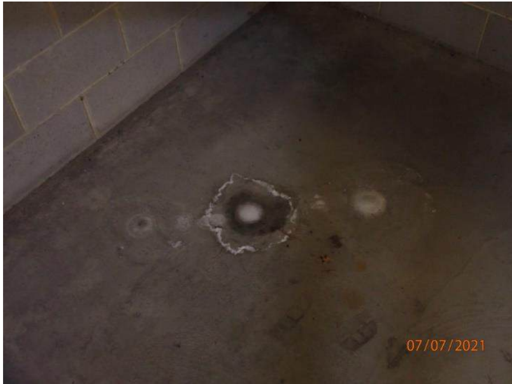
Photograph 13 - Calcium deposits to ground concrete slab of visitor carpark 6
