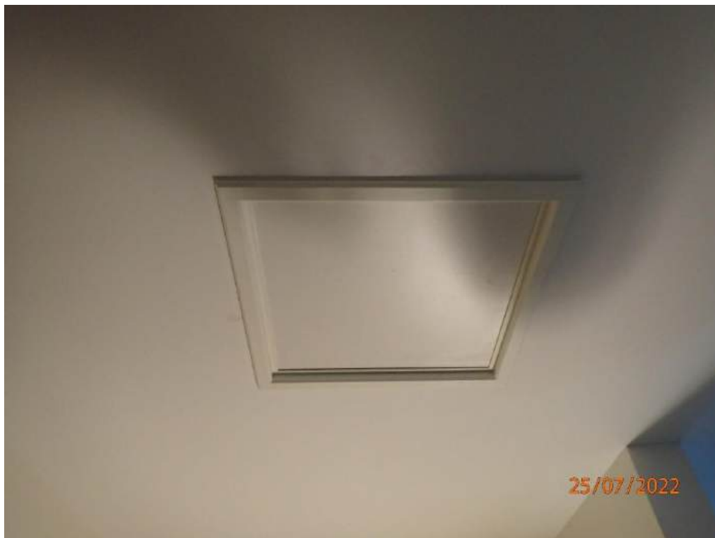
Photograph 168 – Lot 312A/Apartment 312A, entrance hallway ceiling hatch
