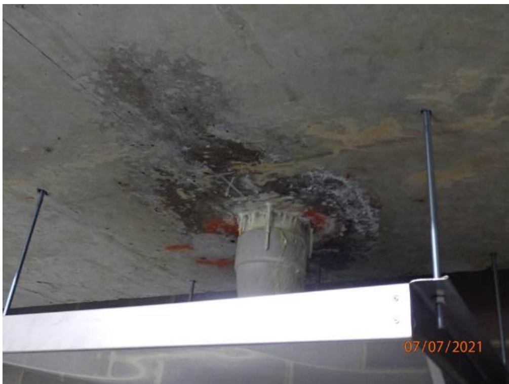
Photograph 6 - efflorescence and calcium deposits at PVC penetration above carpark 70
