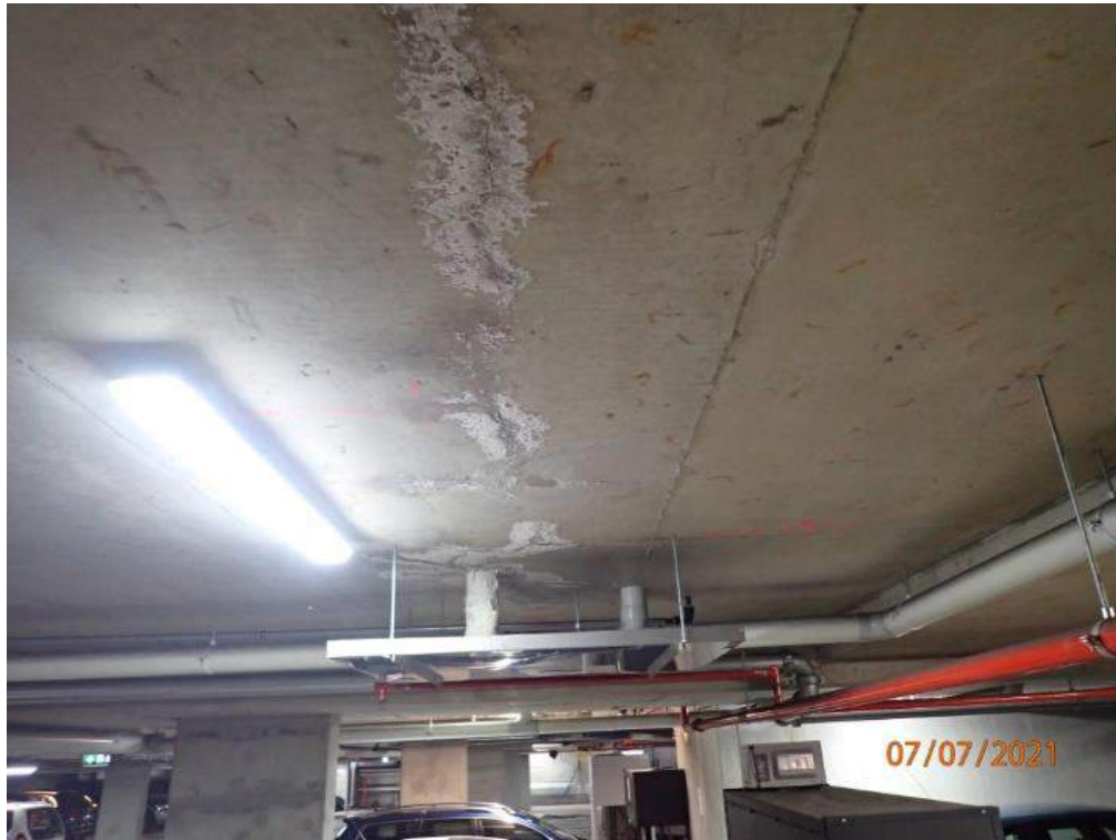
Photograph 61 - Efflorescence, calcium build up and cracking to centre of basement ceiling
