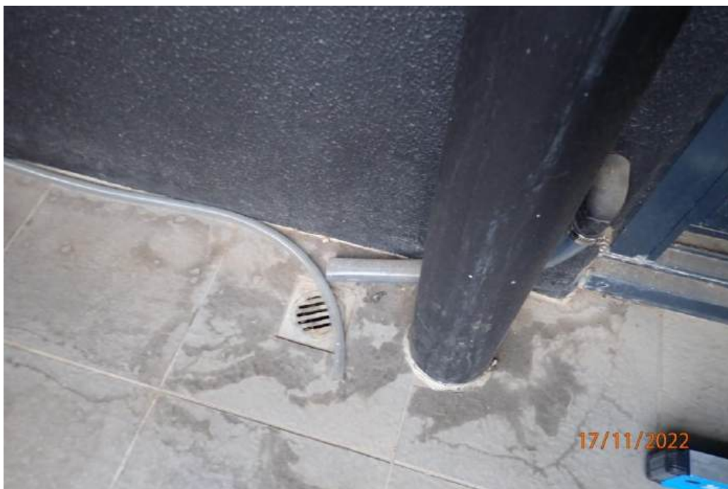
Photograph 106 - Apartment 205A balcony drainage outlet and adjacent drain pipe penetration
