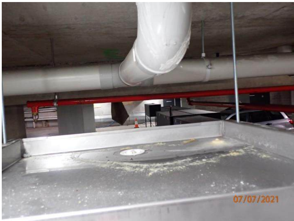
Photograph 40 - Drip tray showing calcification deposits below a pipe penetration
