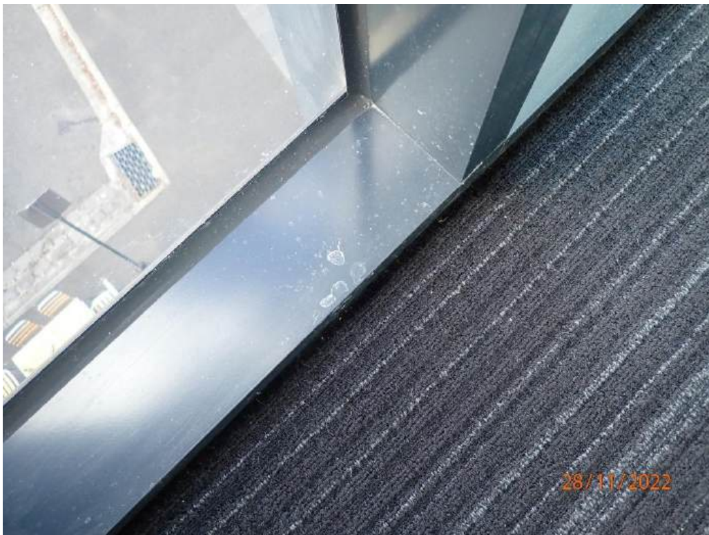
Photograph 84 - Level 4 south passageway aluminium windows, water stains
