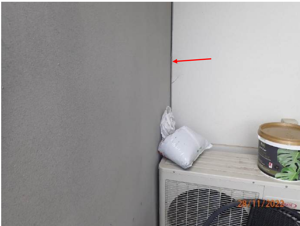
Photograph 78 - Apartment 517B gap between east and north balcony walls
