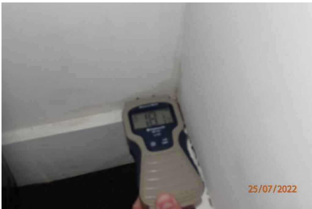
Photograph 144 - Lot 106B/Apartment 116B, southwest bedroom corner moisture reading
