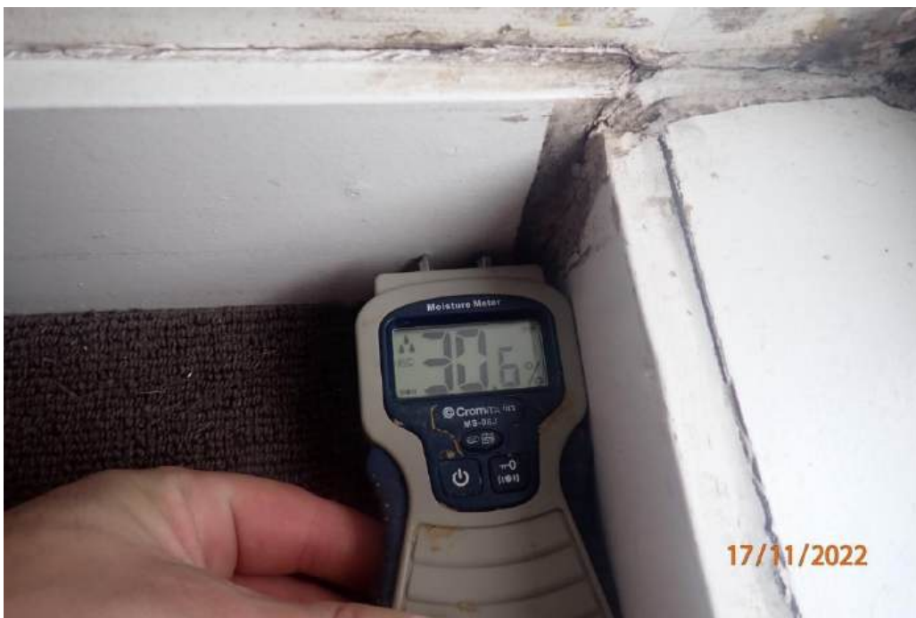
Photograph 130 - Apartment 602B, bedroom window, elevated moisture levels to skirting trim
