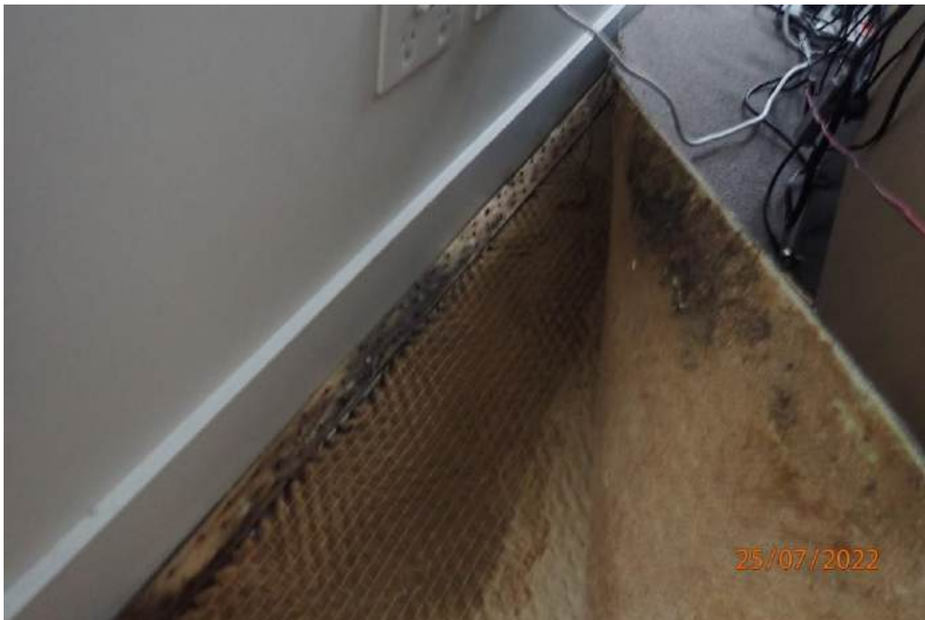
Photograph 200 - Lot 607B/Apartment 605B, north end of west wall opening to the balcony, damage to carpet
