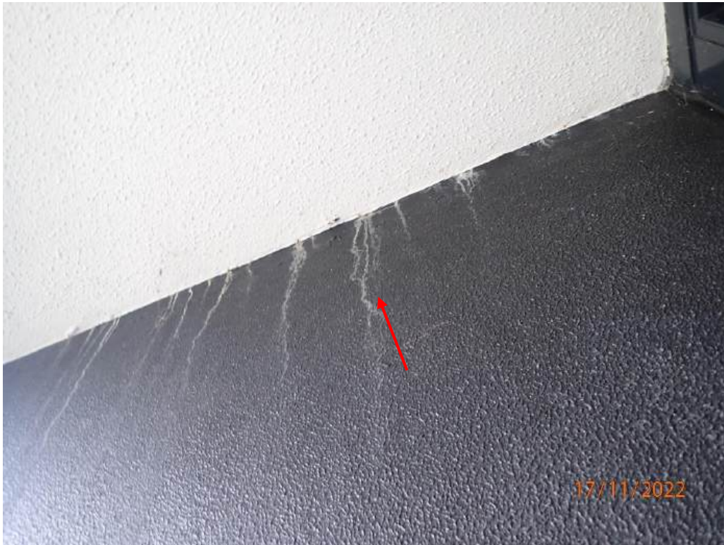
Photograph 23 - Apartment 308A balcony west wall efflorescence discharging from soffit junction
