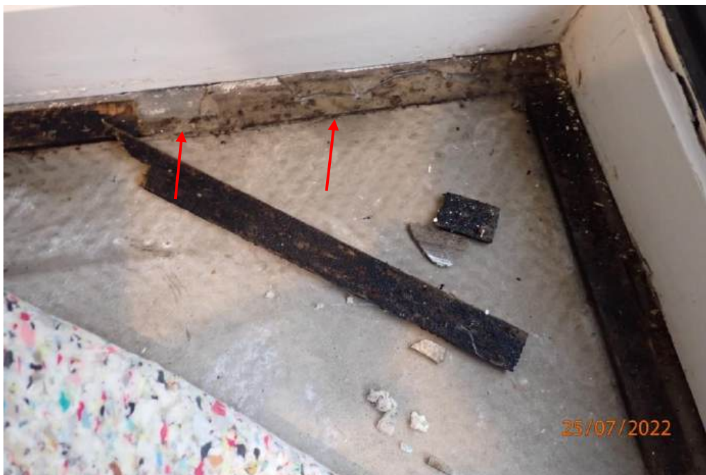
Photograph 184 - Lot 324B/Apartment 336B, north west corner of living area, water ingress from water testing
