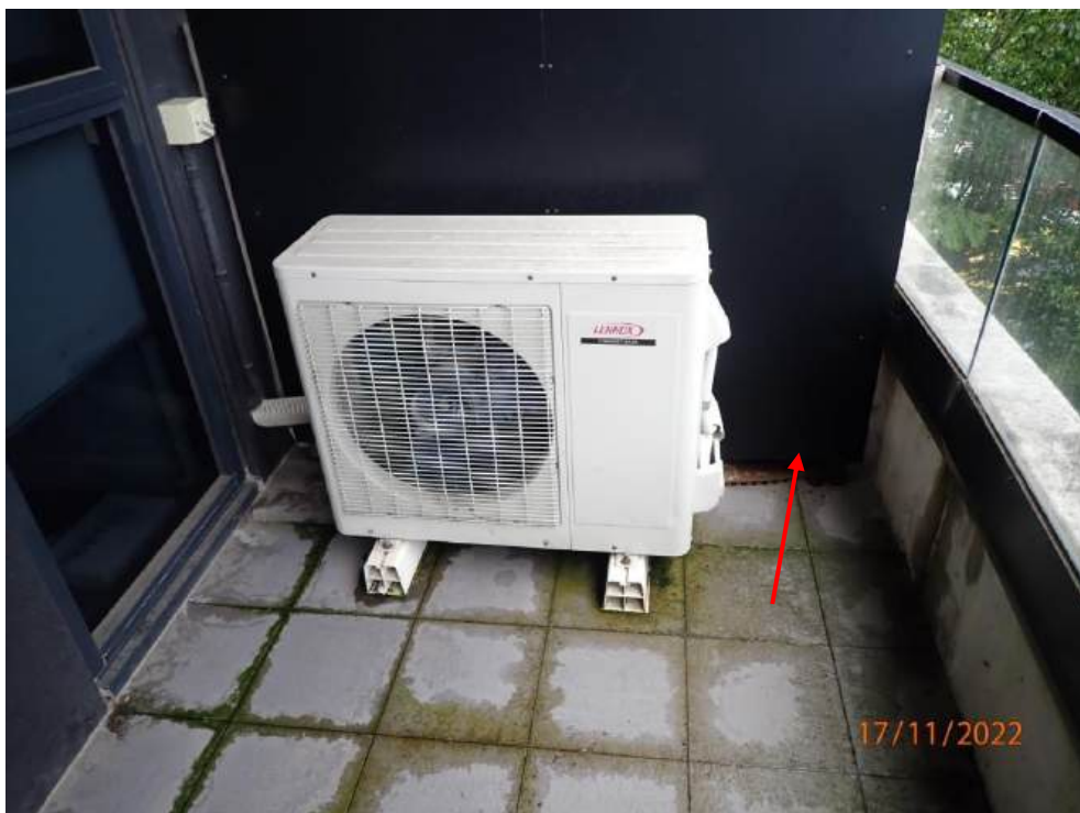
Photograph 20 - Apartment 308A balcony, water discharging beneath east wall
