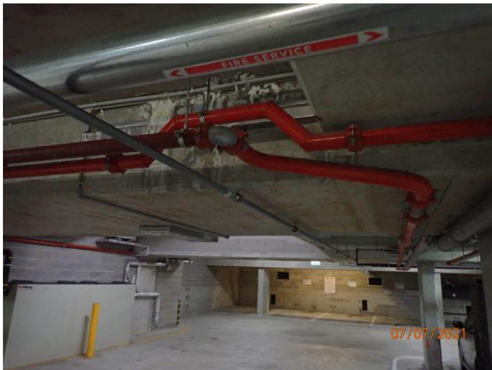
Photograph 18 – Efflorescence and severe calcification build-up to the concrete beam above carpark 43
