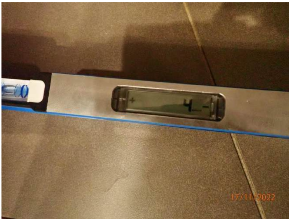
Photograph 3 - Apartment 309A bathroom shower fall 1 in 250
