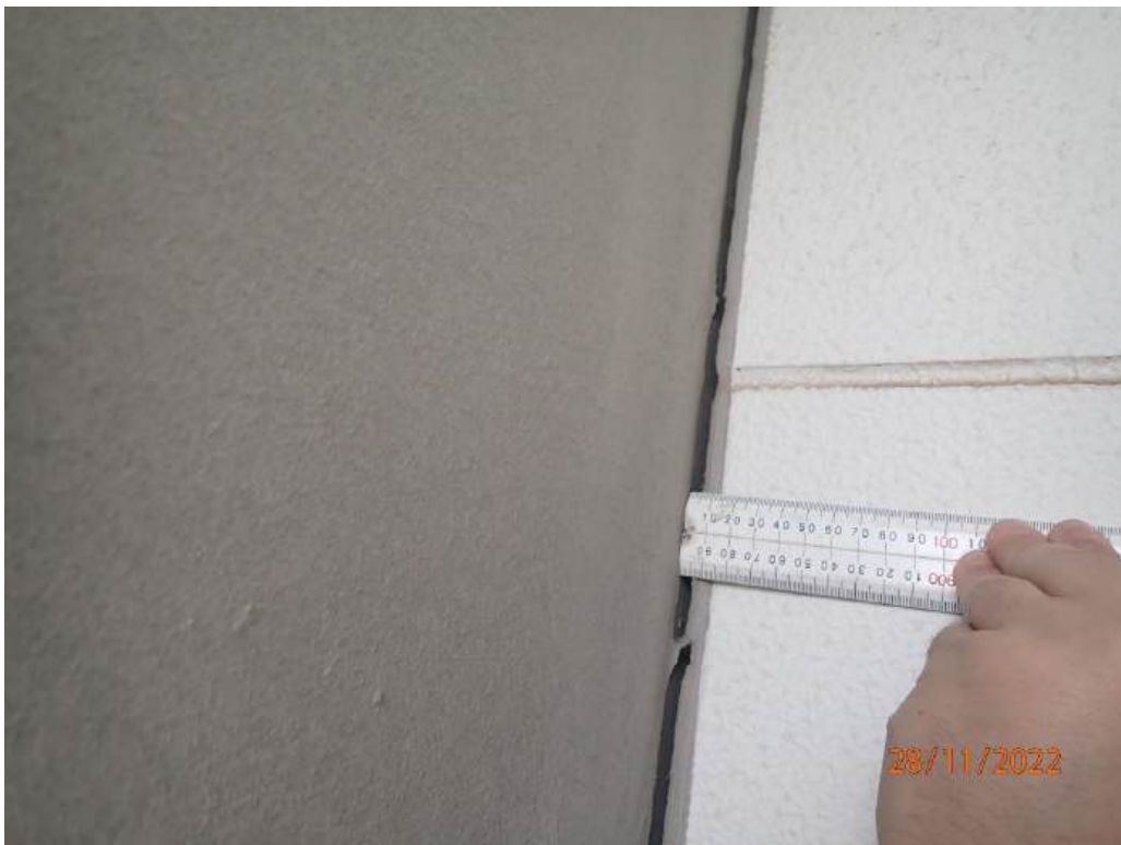
Photograph 80 - Apartment 517B gap between east and north balcony walls
