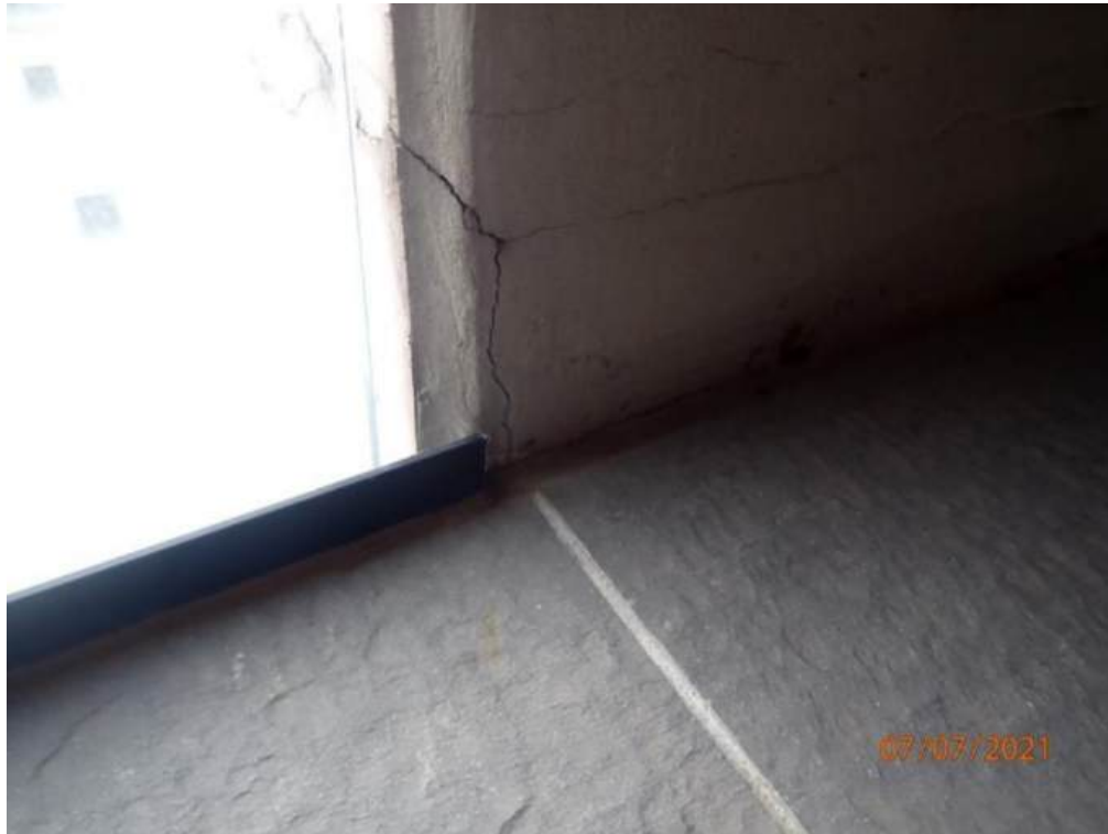
Photograph 99 – Cracking to south elevation of building B
