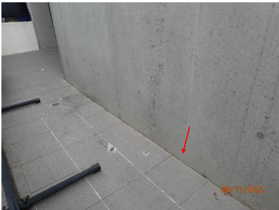
Photograph 104 - Apartment 123B balcony, omission of waterproofing upturns
