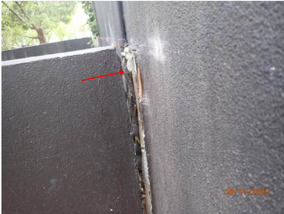
Photograph 141 - Ground level common property to west elevation of north building, gap in block wall in view
