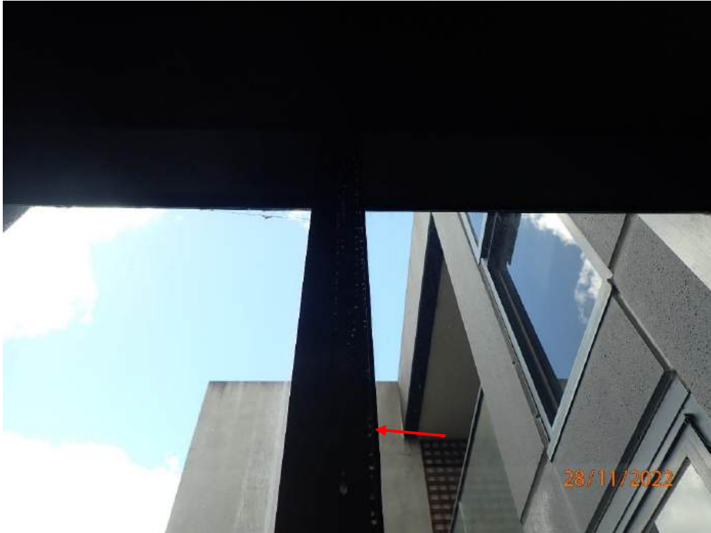
Photograph 85 - Level 4 south passageway aluminium windows, water stains
