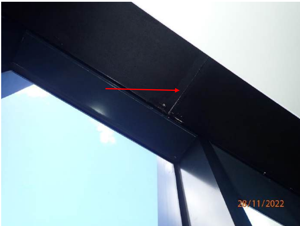
Photograph 86 - Level 4 south passageway aluminium windows, swelling and separation at join of reveal
