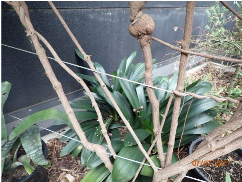
Photograph 73 - Over flashings and capping flashings are not installed to the planter boxes
