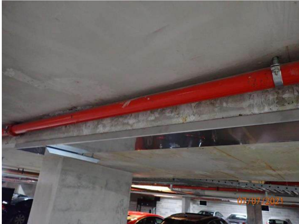
Photograph 47 - Efflorescence and calcium build up
