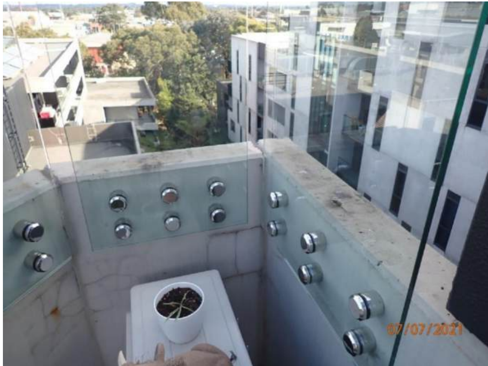
Photograph 113 – Fill is cracking away at tension plates
