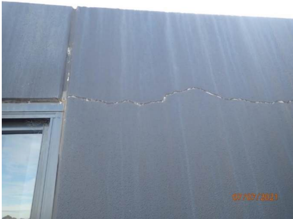
Photograph 95 – Cracking up to 10 mm wide to west elevation of building B
