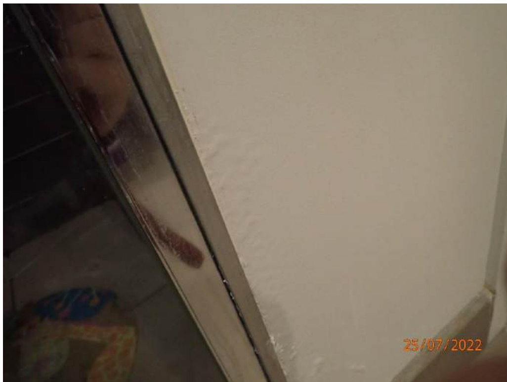
Photograph 166 – Lot 306A/Apartment 306A, moisture damage to lower wall right of the shower
