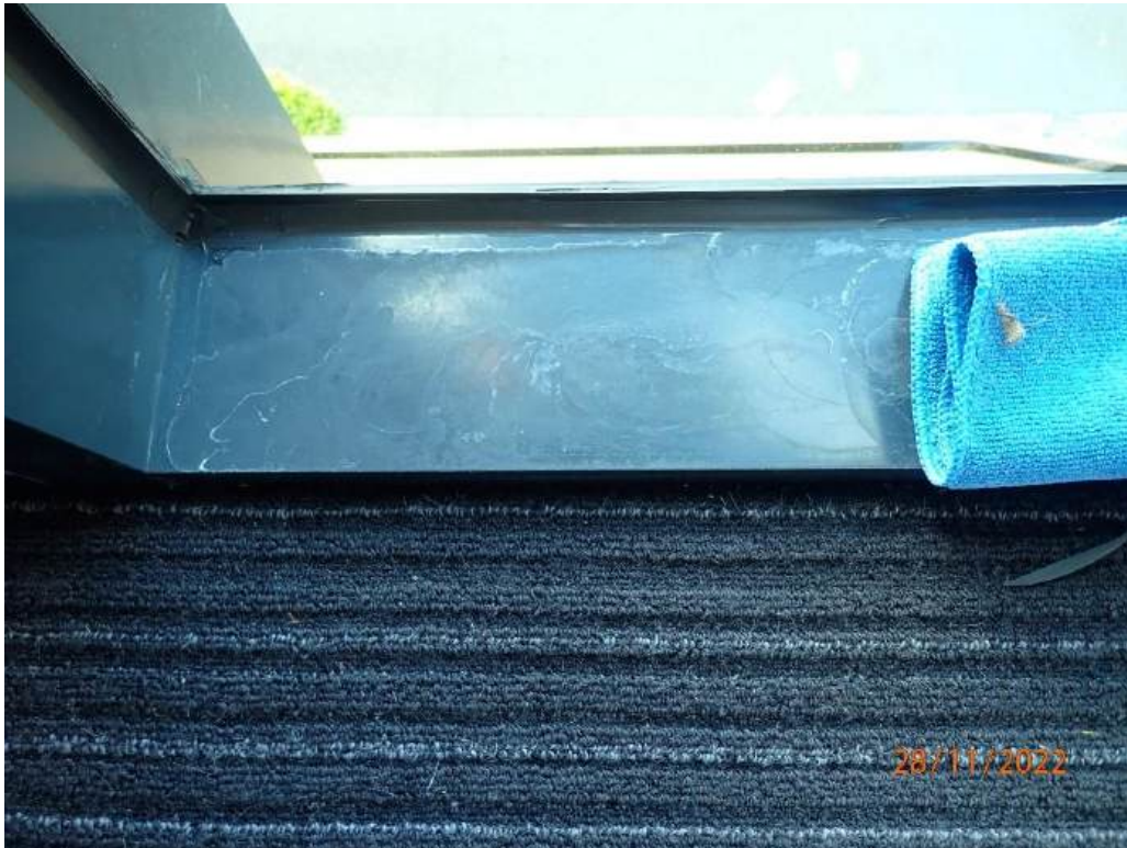
Photograph 83 - Level 4 south passageway aluminium windows, water stains
