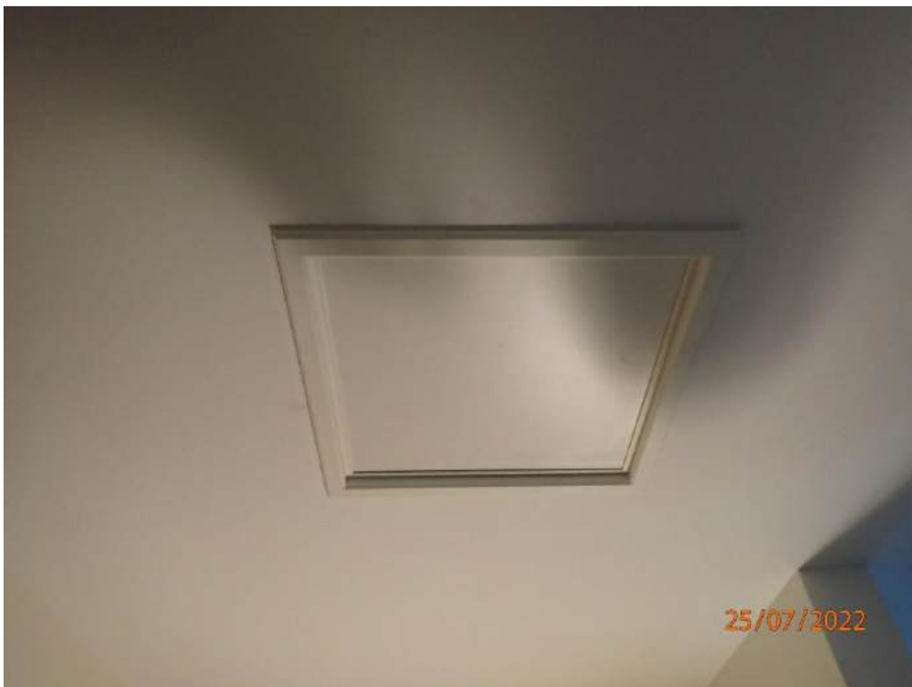
Photograph 168 – Lot 312A/Apartment 312A, entrance hallway ceiling hatch
