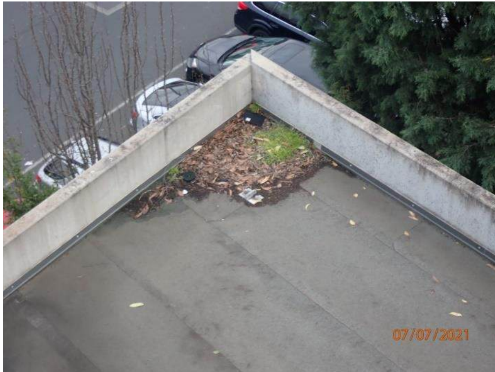
Photograph 127 – Water staining and leaves gathering at external edges of roof to west elevation of building A
