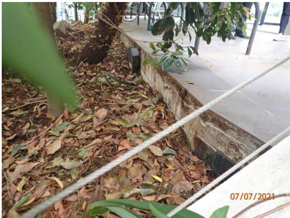
Photograph 70 - Waterproof membrane does not extend above the soil level
