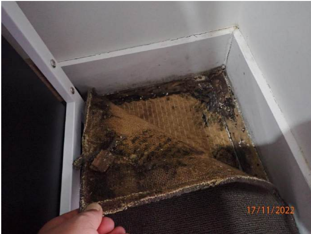
Photograph 61 - Apartment 417B, northwest corner of the living area, water damage to carpet and skirting trim
