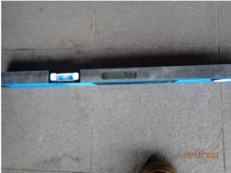
Photograph 11 - Apartment 308A balcony fall 1 in 143
