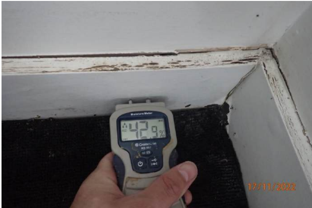
Photograph 113 - Apartment 126B, southeast corner of bedroom 2, high moisture elevation to skirting trim
