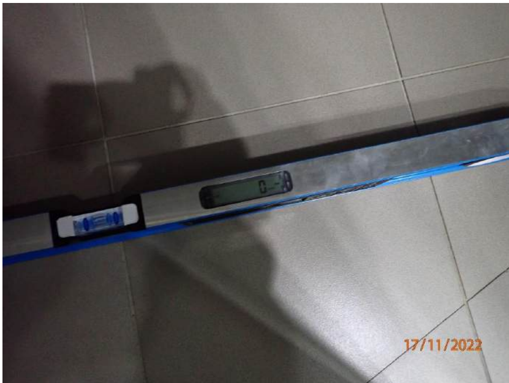
Photograph 34 - Apartment 328B bathroom shower, no fall
