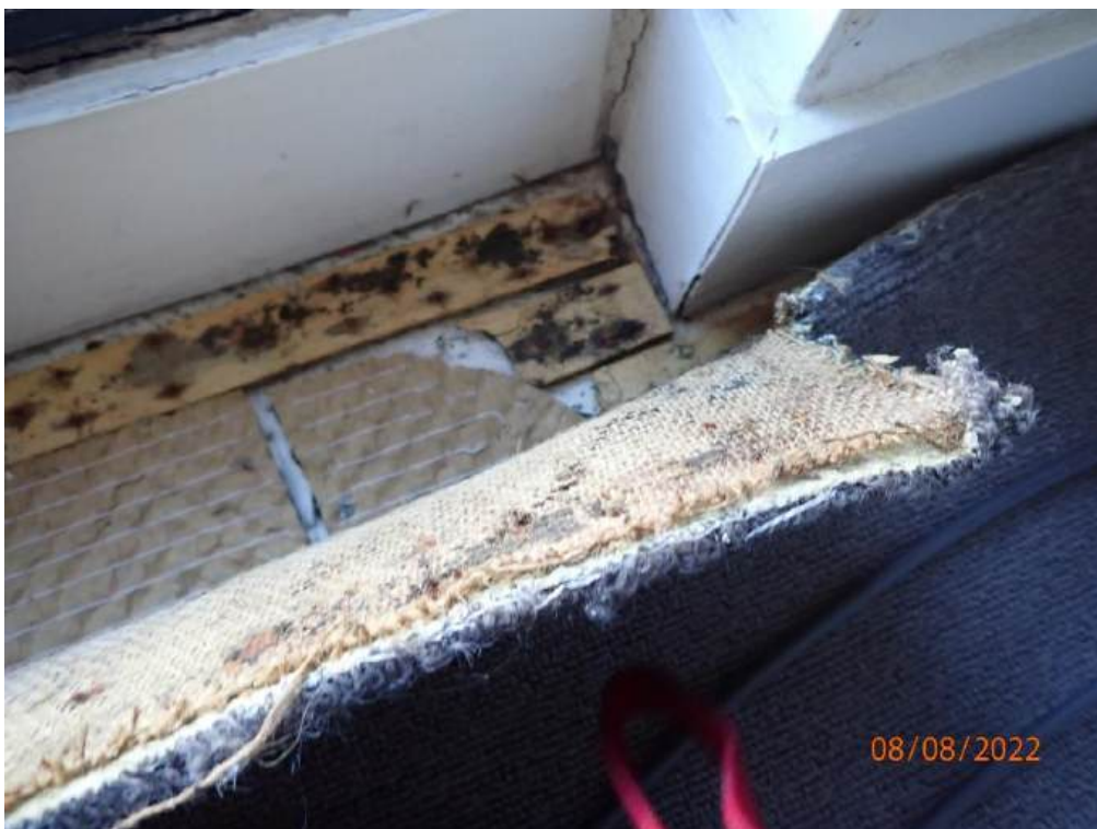
Photograph 206 - 704B/Apartment 703B, west window of the south bedroom, damage to carpet and smooth edge
