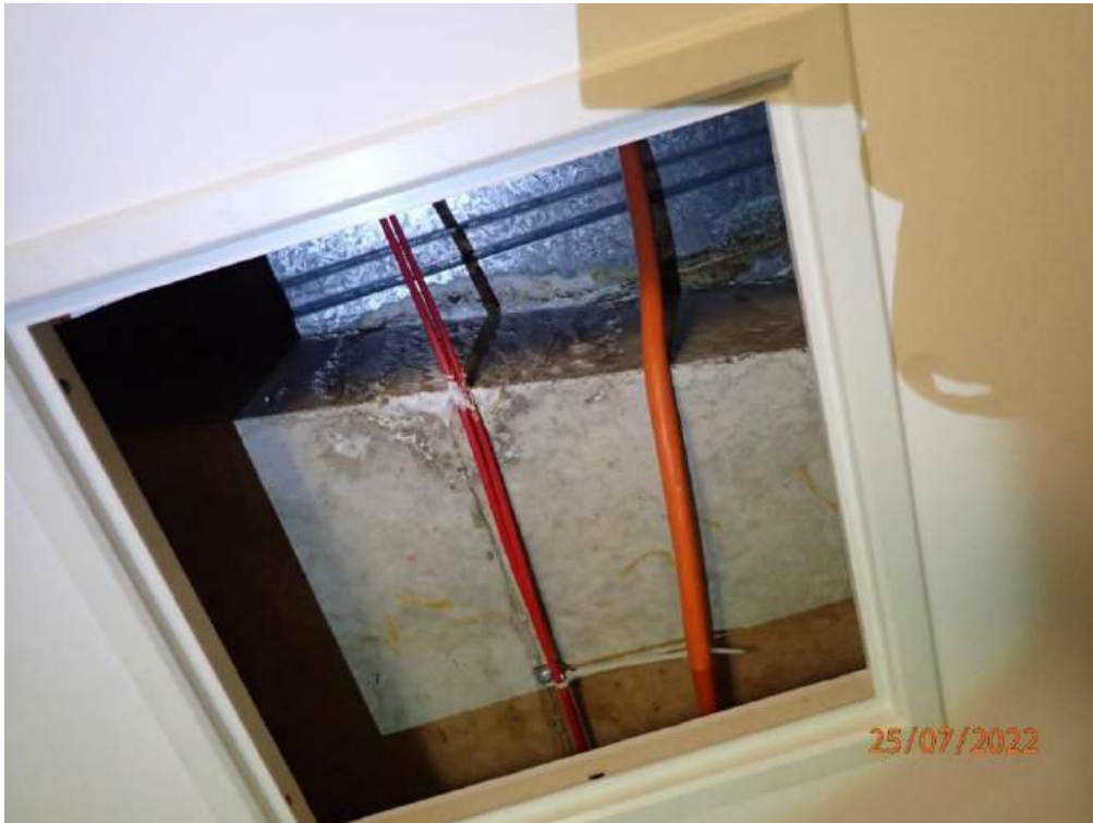
Photograph 169 – Lot 312A/Apartment 312A, concrete roof soffit above ceiling hatch, efflorescence and calcium deposits
