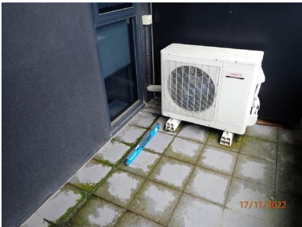
Photograph 16 - Apartment 308A balcony fall
