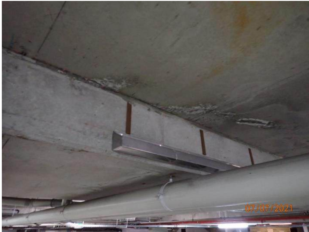
Photograph 33 – Efflorescence, calcification and cracks forming in the concrete ceiling
