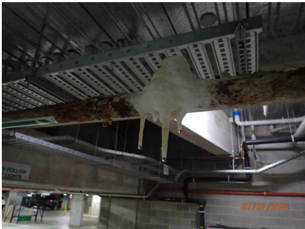
Photograph 16 - Metal water pipe rusted with calcification forming above carpark 65
