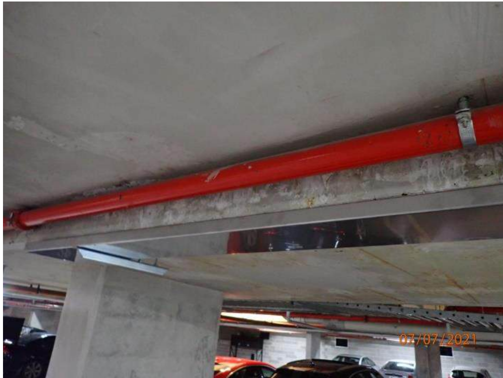
Photograph 47 - Efflorescence and calcium build up
