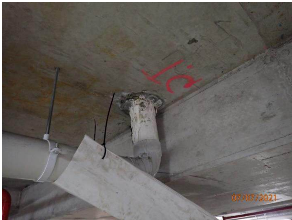
Photograph 34 – Efflorescence and calcification build-up at pipe penetrations
