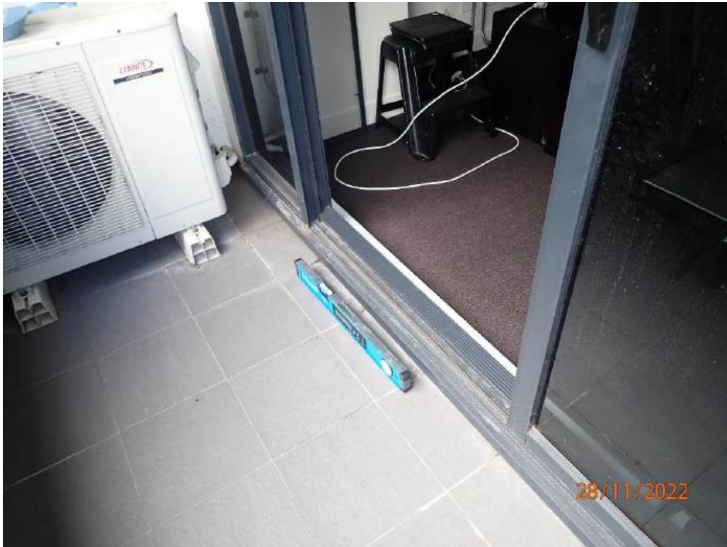
Photograph 91 - Apartment 431B balcony fall
