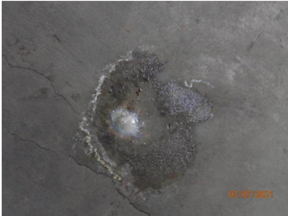
Photograph 17 - Calcium deposits to concrete slab of carpark 65
