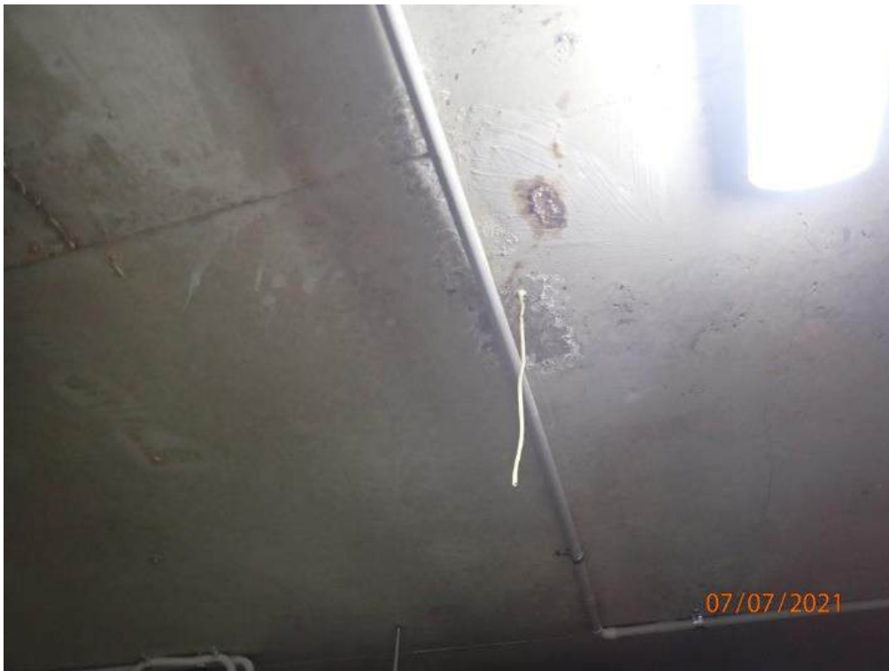
Photograph 50 - Efflorescence, severe calcium build up
