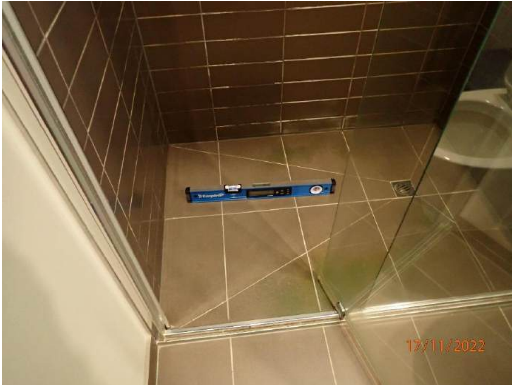
Photograph 27 - Apartment 526B bathroom shower fall
