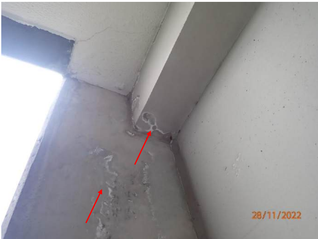
Photograph 76 - Apartment 518B, northeast balcony wall, efflorescence in view
