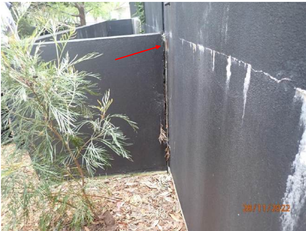
Photograph 140 – Ground level common property to west elevation of north building, gap in block wall
