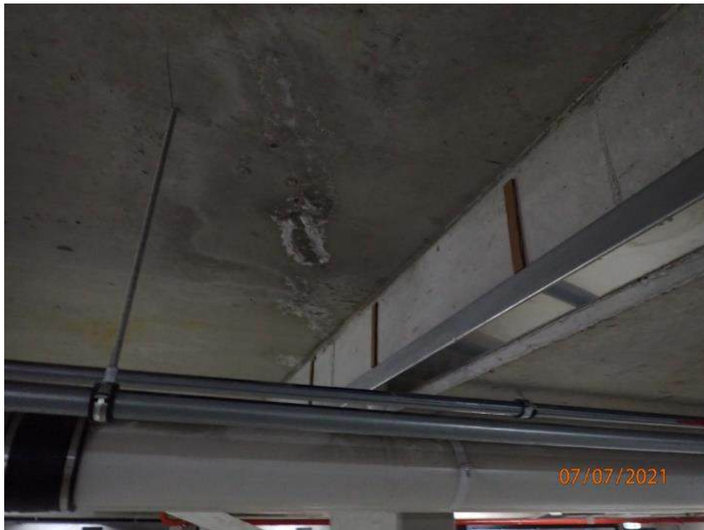
Photograph 32 - Efflorescence, calcification and cracks forming in the concrete ceiling
