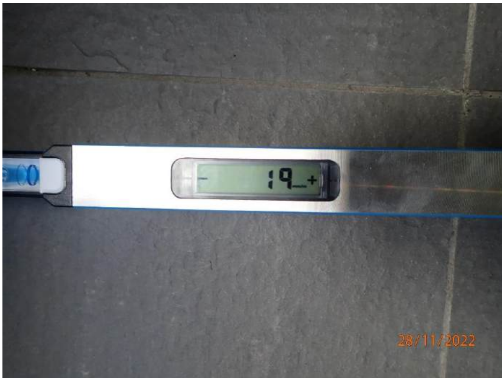
Photograph 96 - Apartment 431B balcony cross fall 1 in 50
