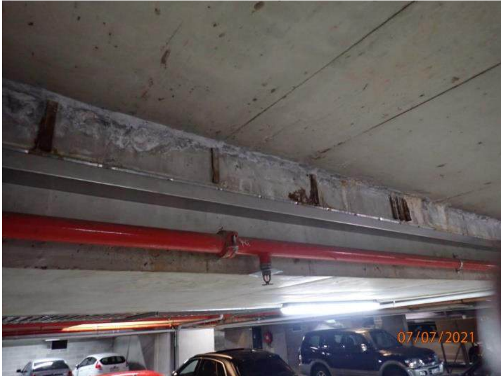
Photograph 23 - Efflorescence, severe calcification build-up and rusty steel components to concrete beams and pipe penetrations near carpark 48 including surrounding carparks
