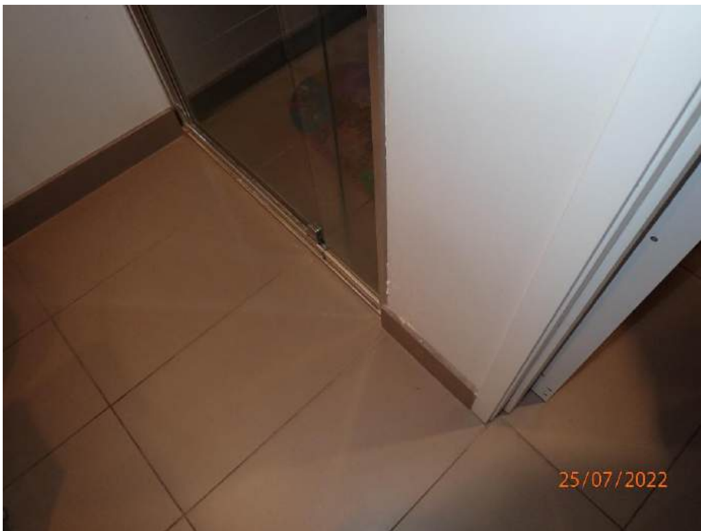
Photograph 164 – Lot 306A/Apartment 306A, affected wall right of the shower
