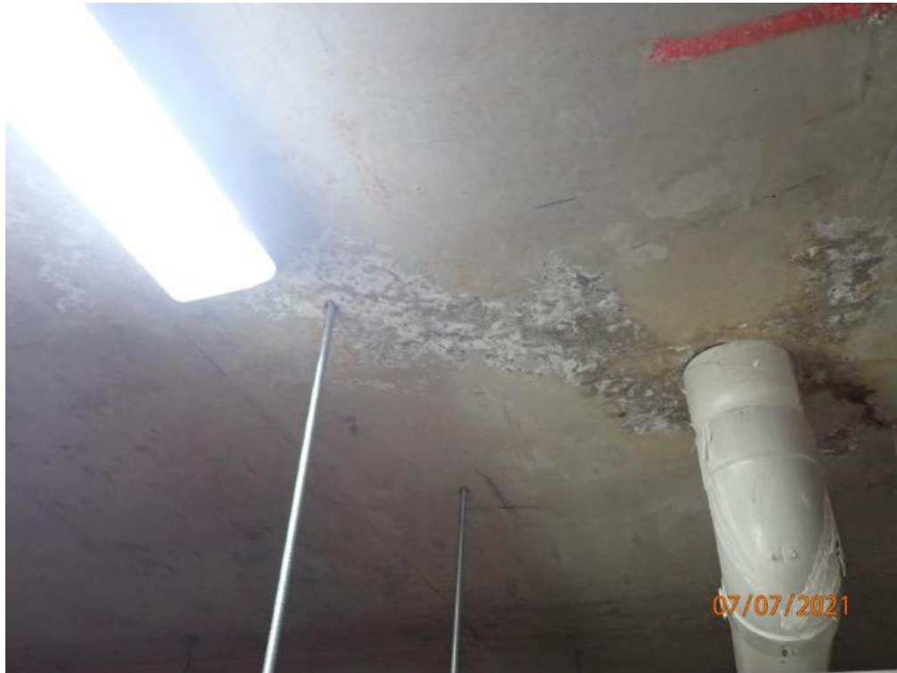
Photograph 41 - Efflorescence, calcium build up and concrete cracking to the ceiling and around pipe penetrations
