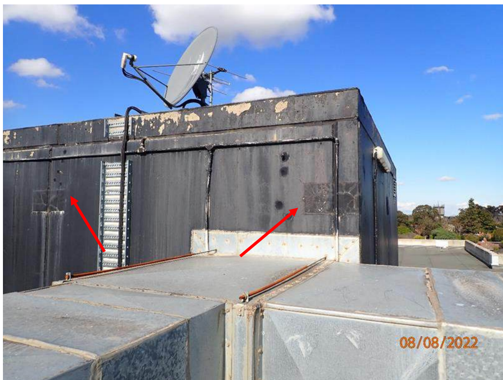
Photograph 140 - Building B facing north west corner of the north stairwell wall at rooftop level, deteriorating patching
