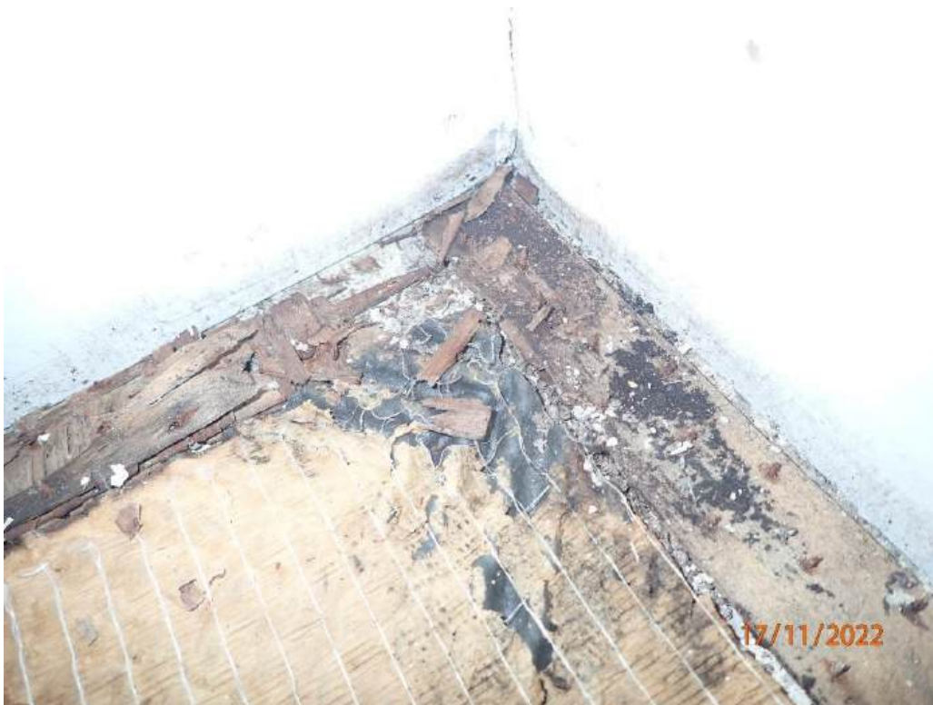
Photograph 62 - Apartment 417B, northwest corner of the living area, water damage to carpet, underlay, smooth edge and skirting trim
