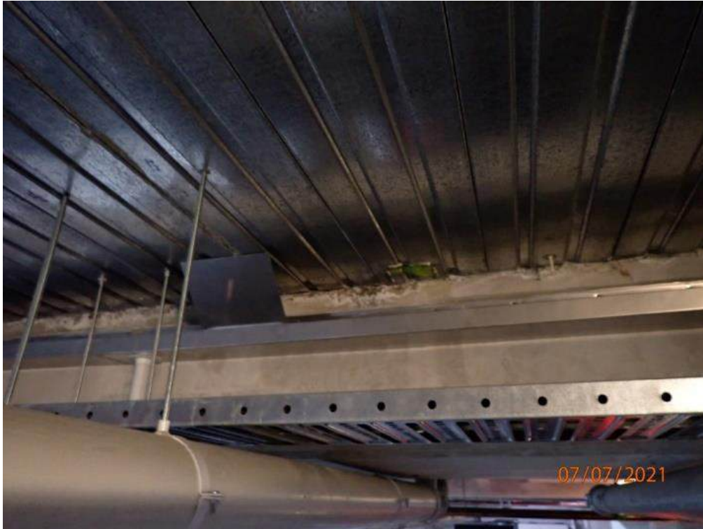
Photograph 45 – Efflorescence and calcium build up
