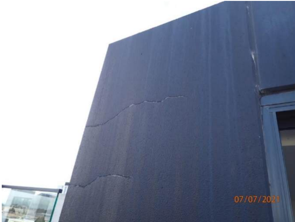
Photograph 93 – Cracking to west elevation of building B
