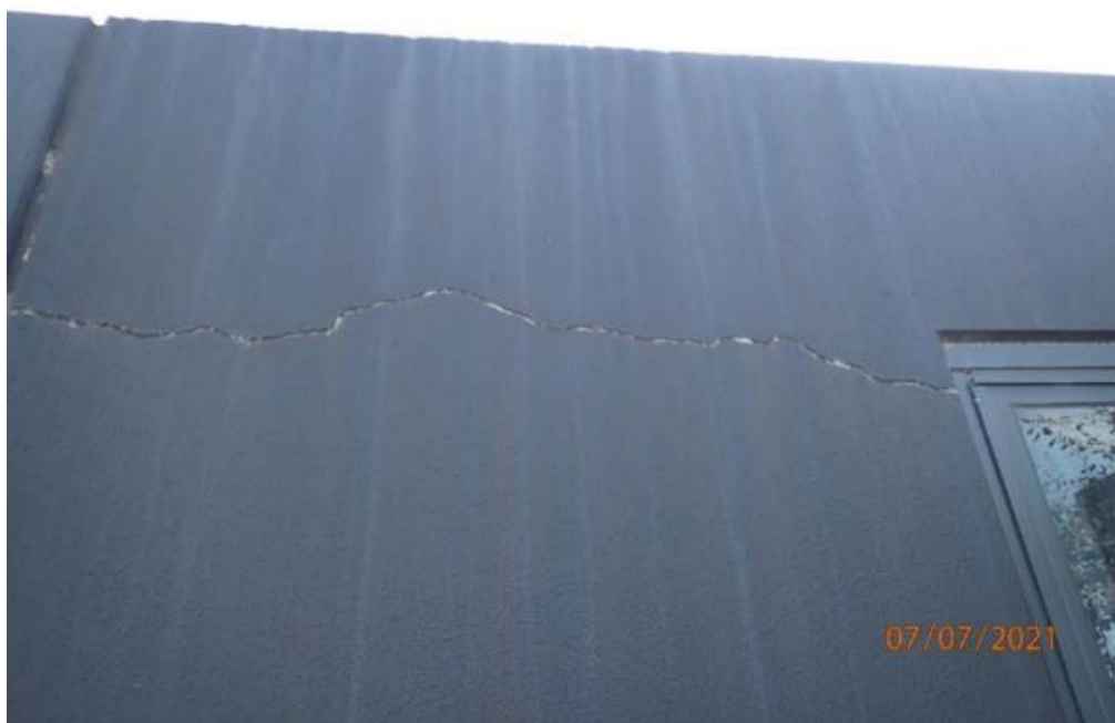
Photograph 96 – Cracking to west elevation of building B
