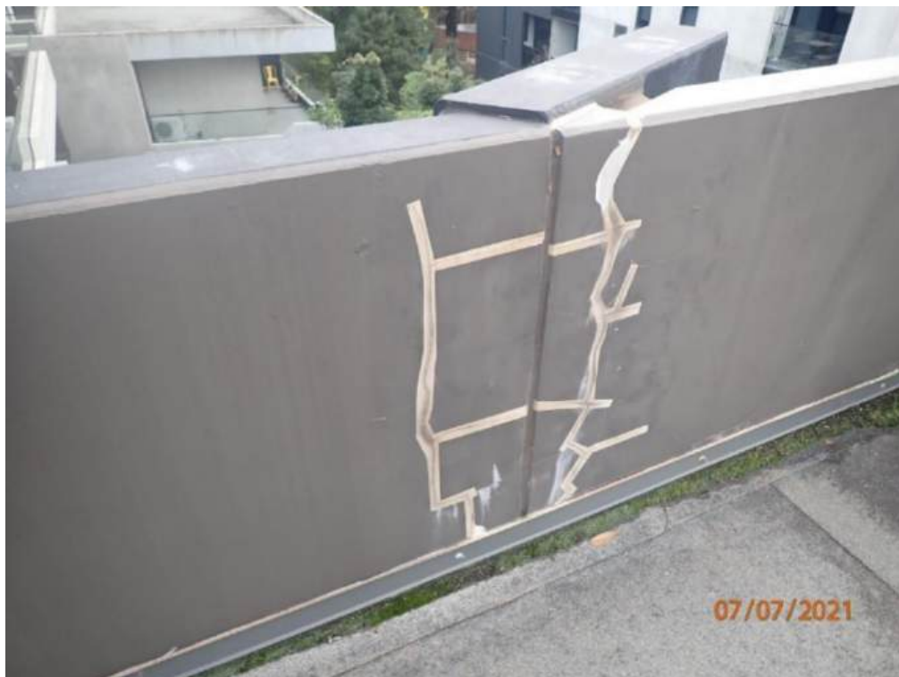
Photograph 108 – Cracking to the concrete wall panels to the north elevation of building A
