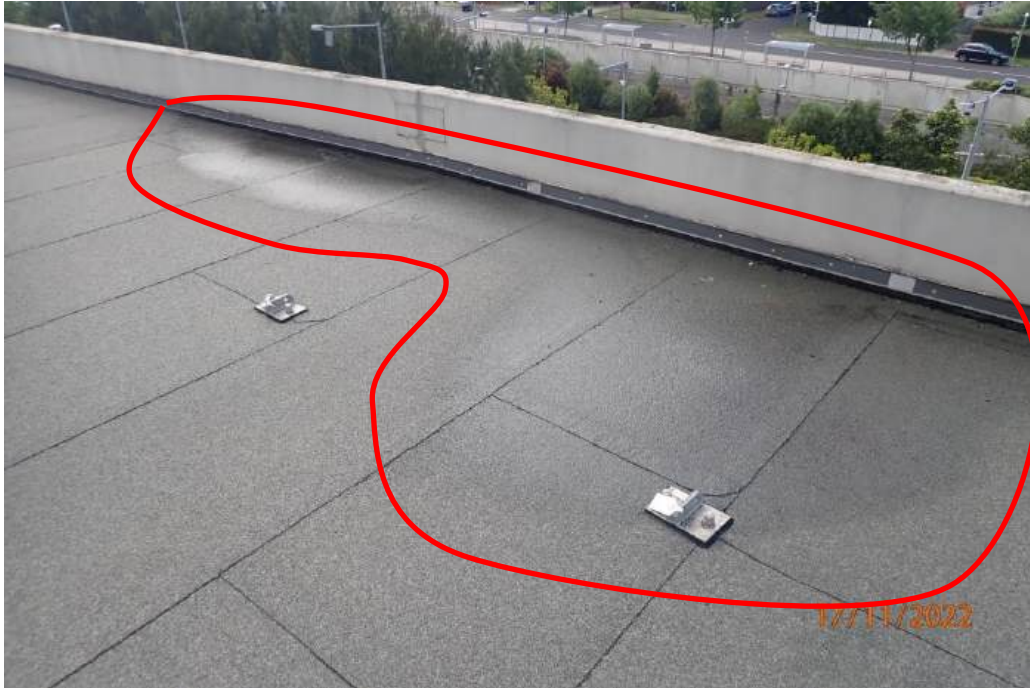
Photograph 137 – Rooftop above Apartment 510A bedroom, area of water pooling
