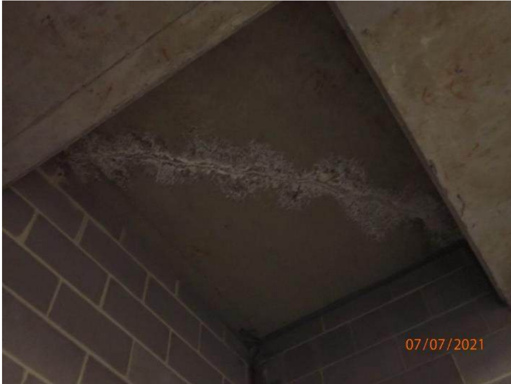
Photograph 11 - Efflorescence and concrete cracked to south elevation above visitor carpark 6
