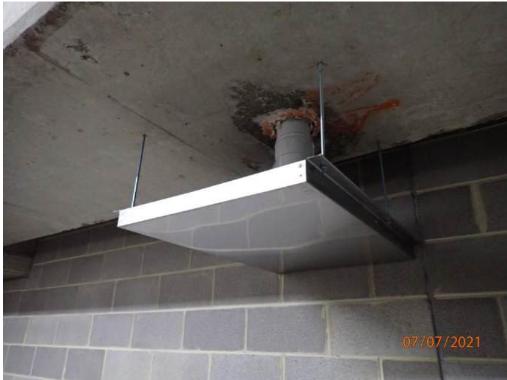
Photograph 9 - Efflorescence and calcium deposits at PVC penetration above carpark 68
