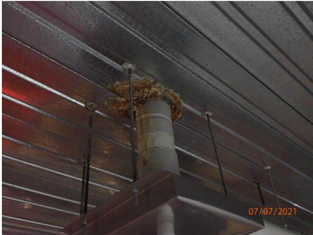
Photograph 35 – Efflorescence and calcification build-up at pipe penetrations
