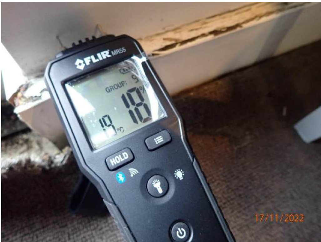
Photograph 56 - Apartment 417B bedroom 2, elevated moisture levels in wall plaster
