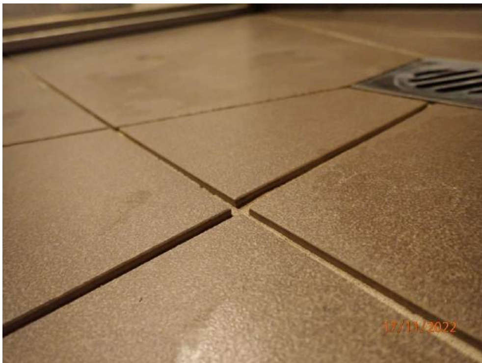
Photograph 8 - Apartment 309A bathroom shower recessed grout lines
