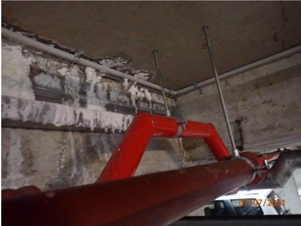
Photograph 19 - Efflorescence and severe calcification build-up to the concrete beam above carpark 43
