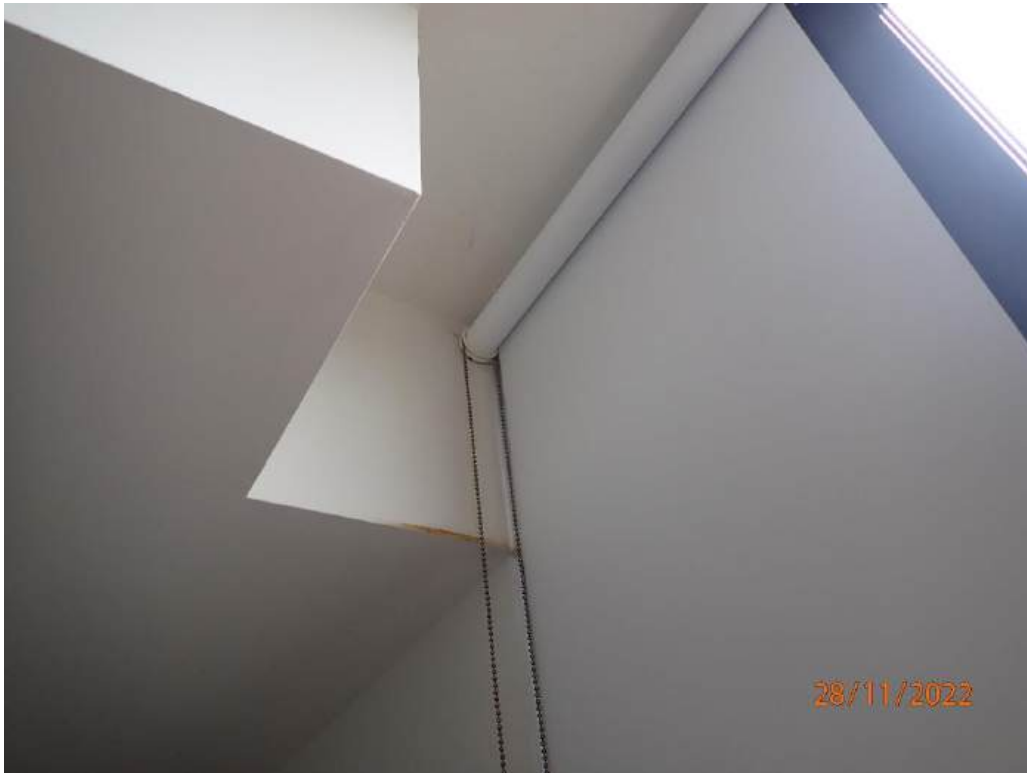
Photograph 99 – Apartment 604B, living area opening pelmet
