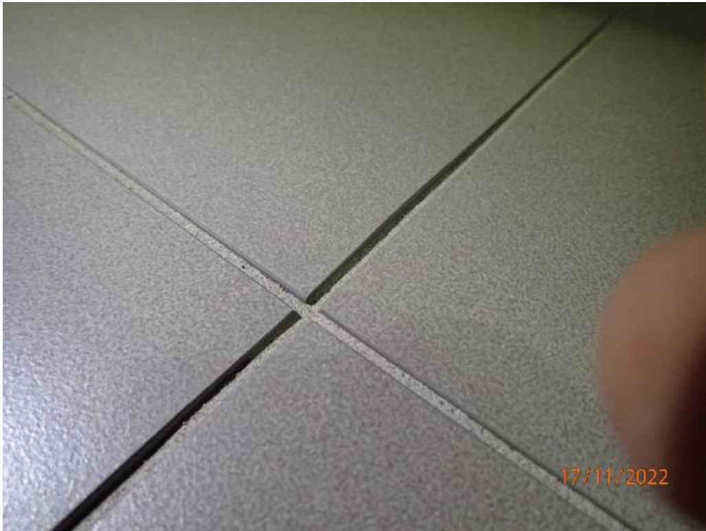
Photograph 39 - Apartment 328B bathroom shower recessed grout lines
