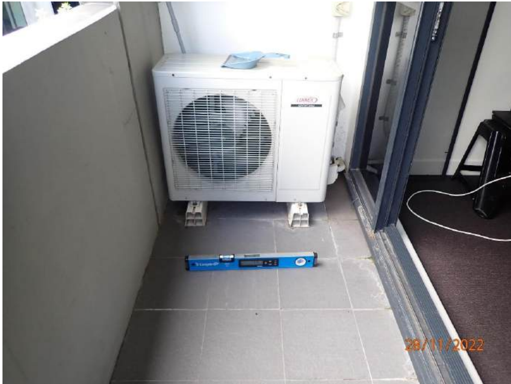
Photograph 95 - Apartment 431B balcony cross fall
