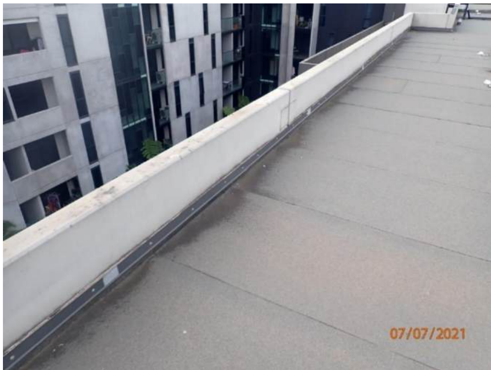
Photograph 130 - Butynol waterproofing sheets which are loose under foot
