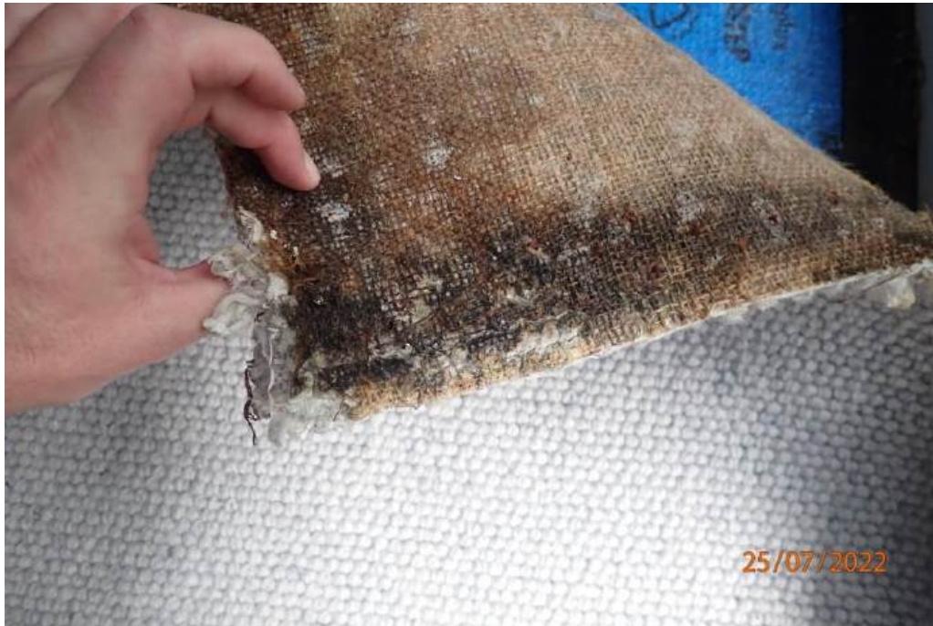
Photograph 179 – Lot 324B/Apartment 336B, north west corner of living area, carpet staining to underside of carpet
