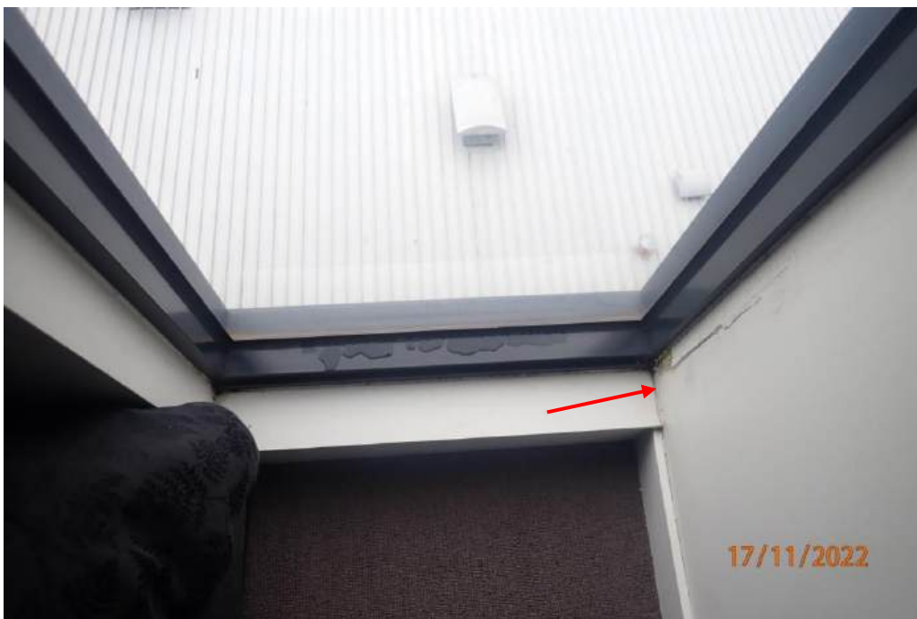
Photograph 124 – Apartment 607B, bedroom window, plaster damage
