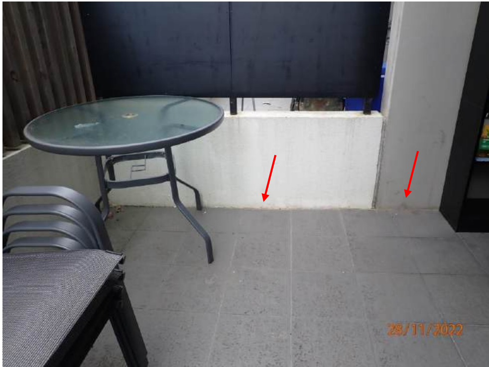
Photograph 103 - Apartment 123B balcony, omission of waterproofing upturns
