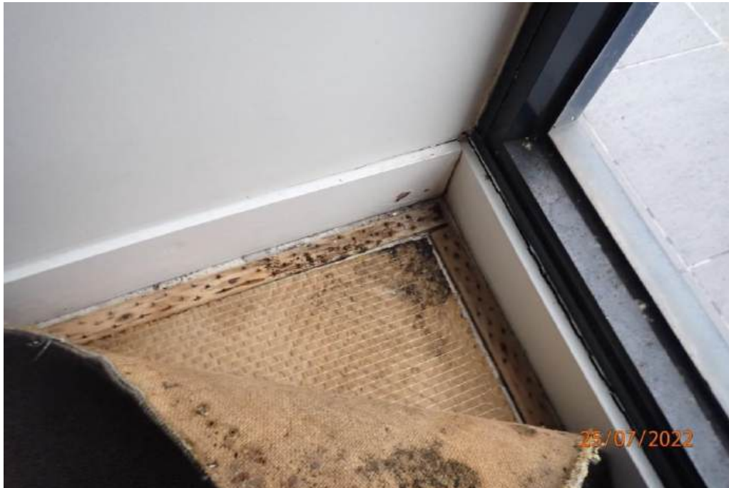
Photograph 201 - Lot 607B/Apartment 605B, south end of west wall opening to the balcony, damage to carpet
