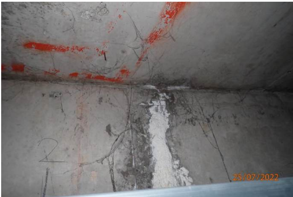
Photograph 150 - No evidence of a drainage point
