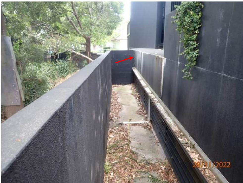
Photograph 142 - Ground level common property to west elevation of north building, gap in block wall in view
