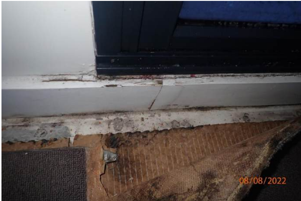
Photograph 213 - 704B/Apartment 703B, living sliding door opening to balcony water and mould damage to underside of carpet
