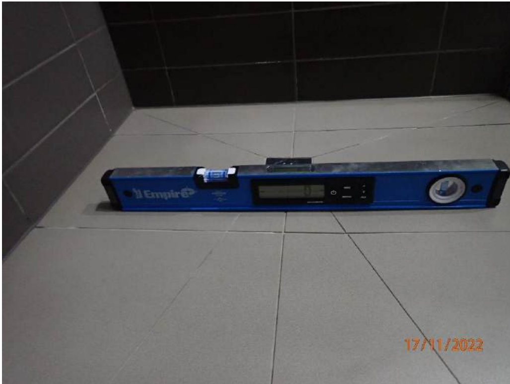
Photograph 37 - Apartment 328B bathroom shower fall
