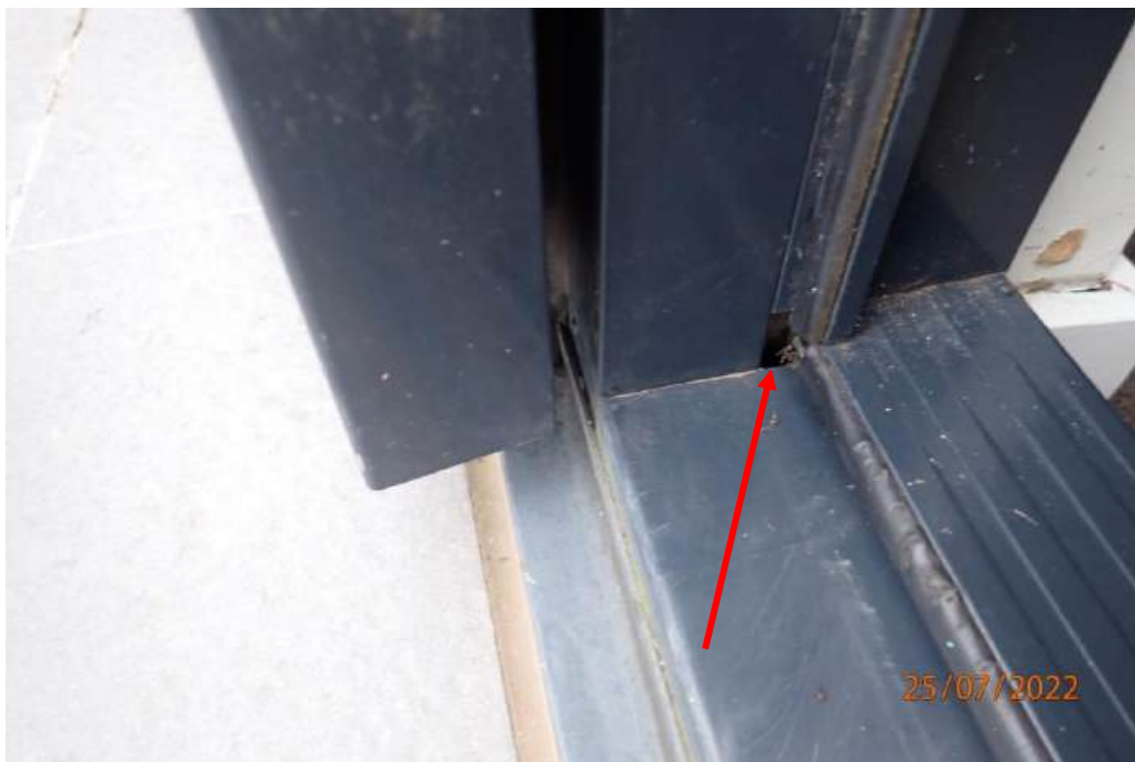
Photograph 198 - Lot 607B/Apartment 605B, north end of west wall opening door to the balcony, gap in sill
