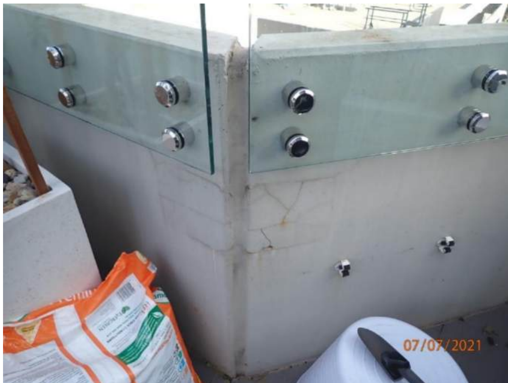
Photograph 114 – Fill is cracking away at tension plates
