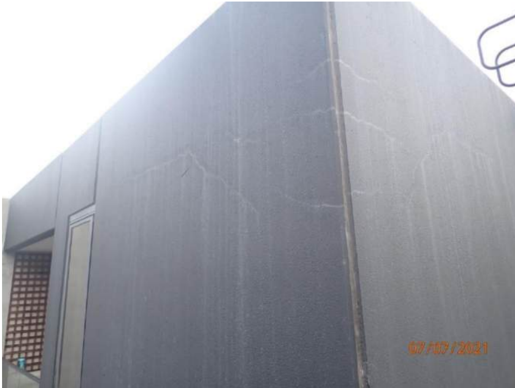
Photograph 103 – Cracking to concrete wall panels to north elevation of building A
