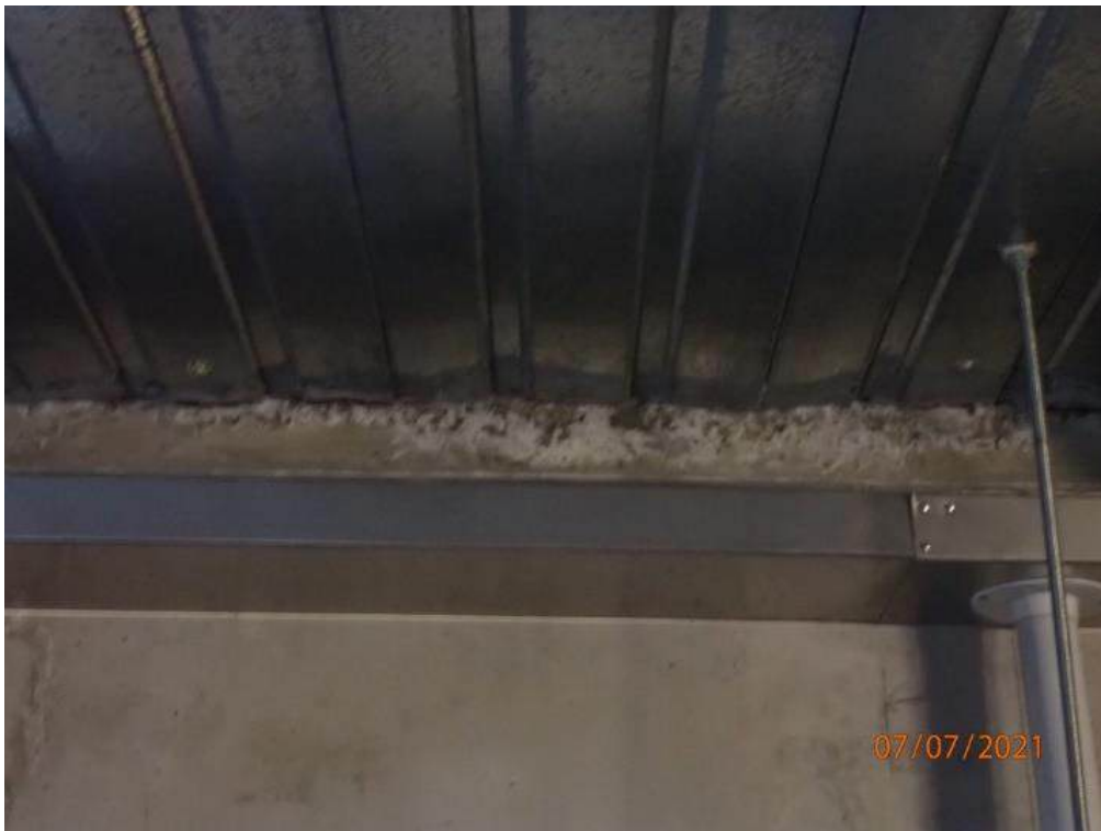
Photograph 46 - Efflorescence and calcium build up
