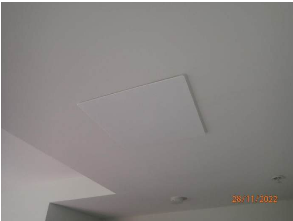
Photograph 66 - Apartment 614B living area ceiling
