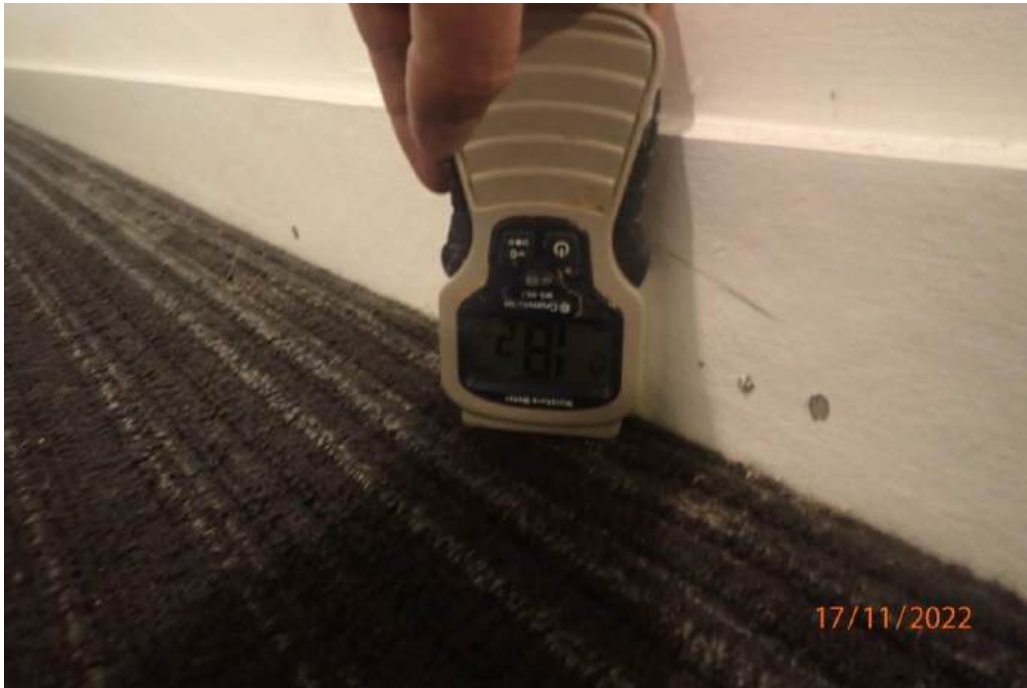
Photograph 119 - Apartment 521B external passageway, elevated moisture levels in carpet and underlay
