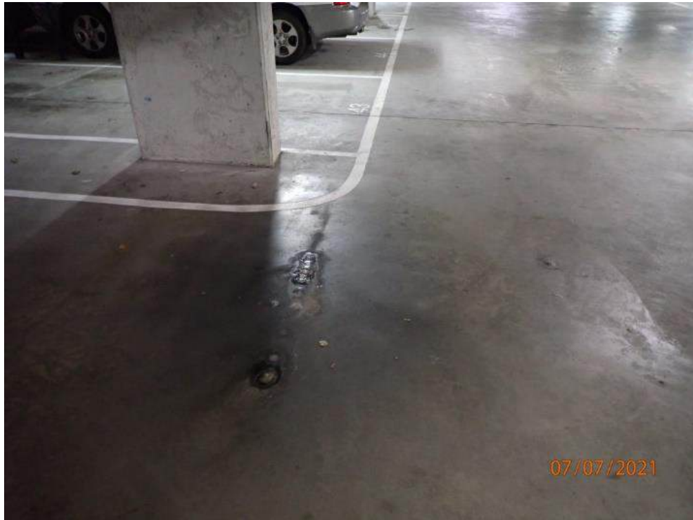
Photograph 59 - Calcium build up to concrete basement floor
