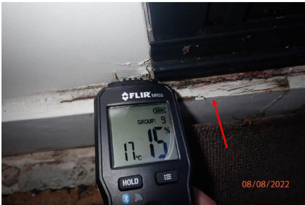
Photograph 216 - 704B/Apartment 703B, water ingress to living sliding door from water testing
