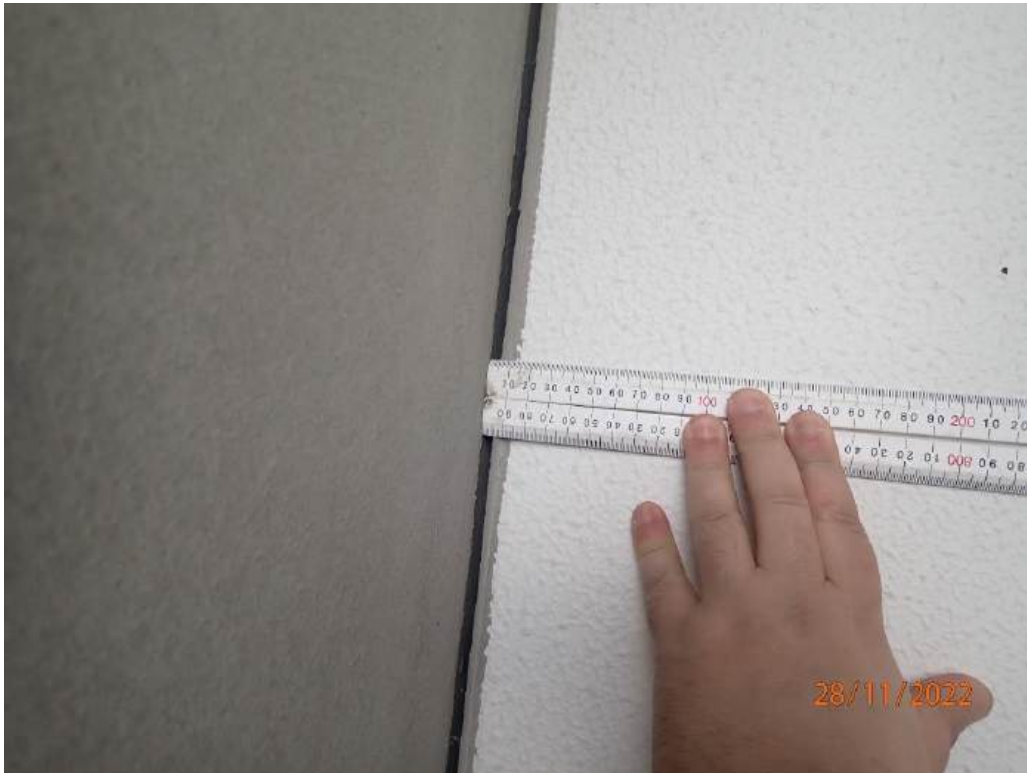
Photograph 79 - Apartment 517B gap between east and north balcony walls
