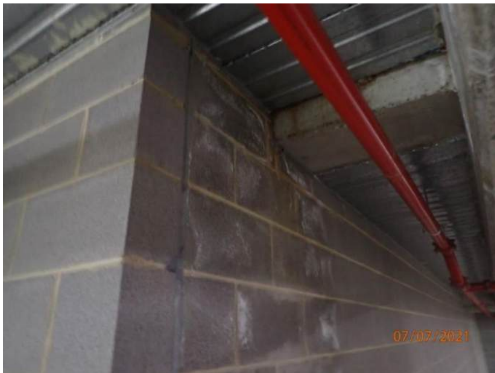
Photograph 88 – Efflorescence to the block walls adjacent the water tanks
