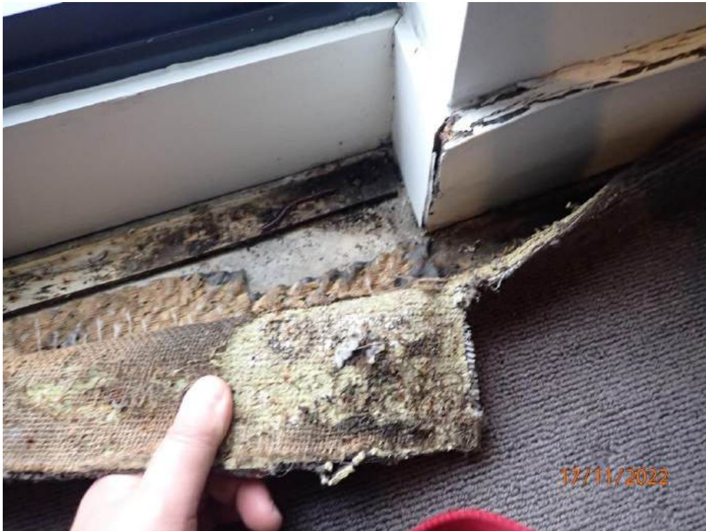
Photograph 53 - Apartment 417B bedroom 2 moisture damage to skirting trim and carpet
