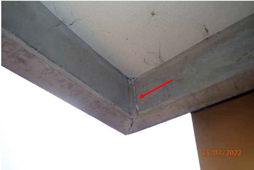
Photograph 193 - Lot 418B/Apartment 428B, south west balcony soffit, efflorescence visible from Lot 321B/Apartment 333B
