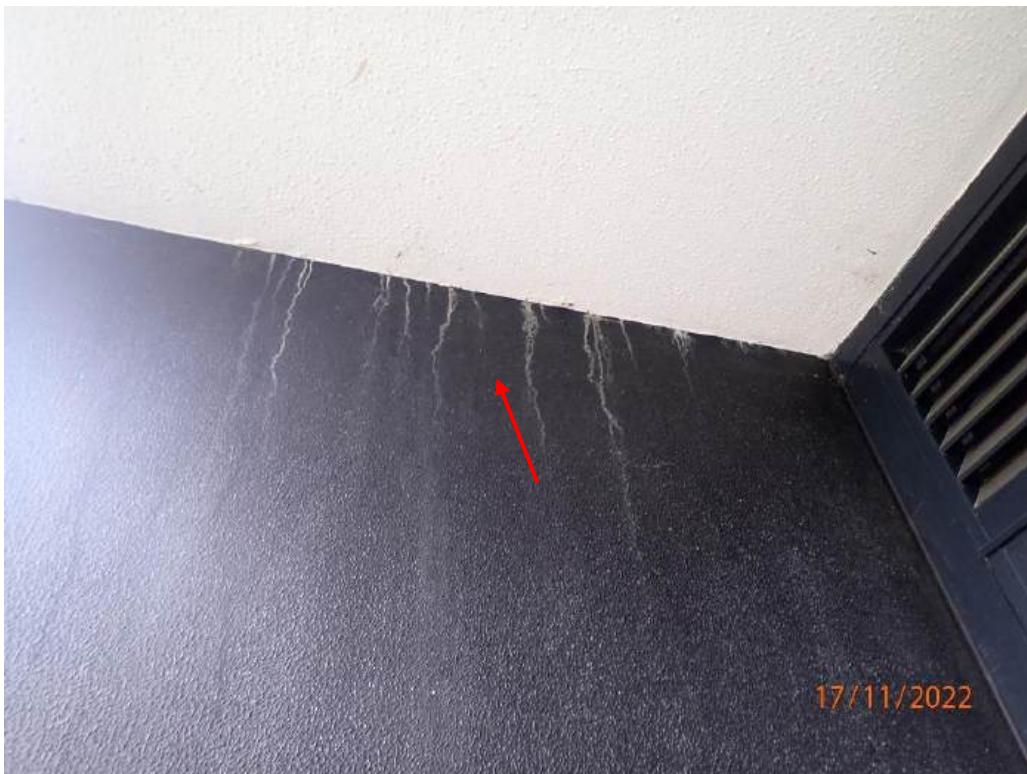
Photograph 22 - Apartment 308A balcony west wall efflorescence discharging from soffit junction
