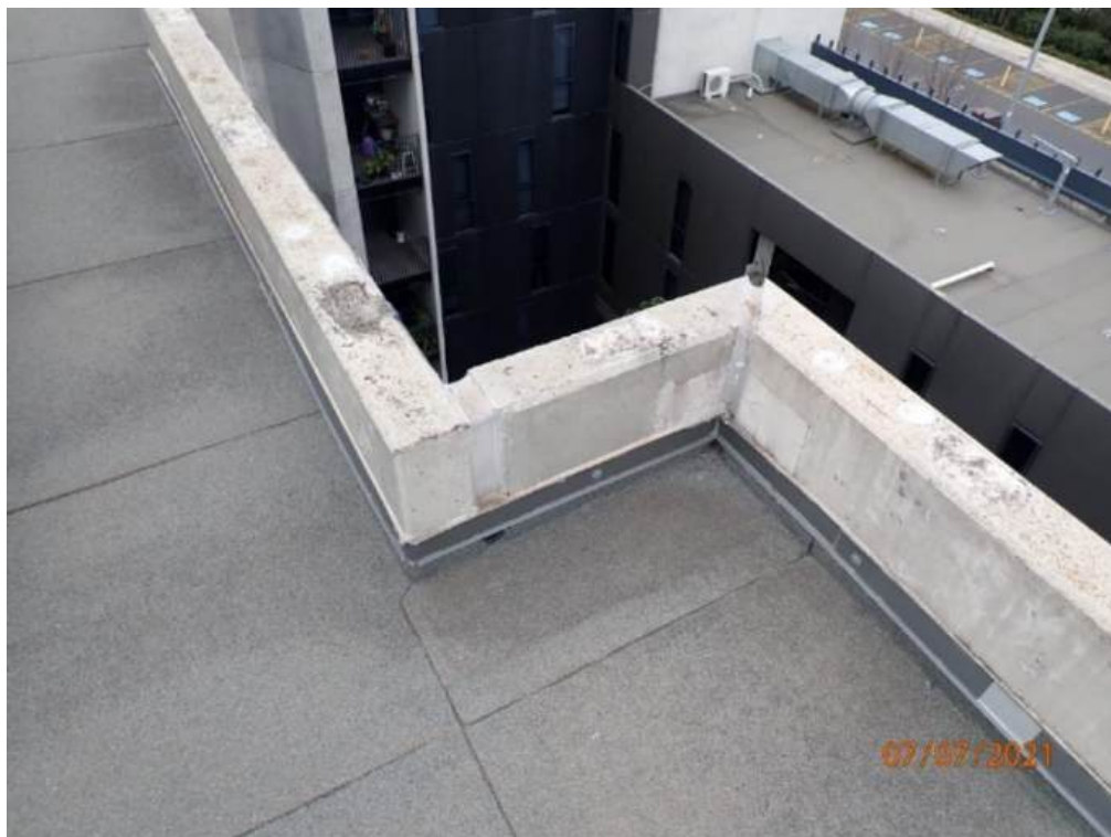
Photograph 116 – Gaps between concrete wall panels exceeding 50 mm to building B
