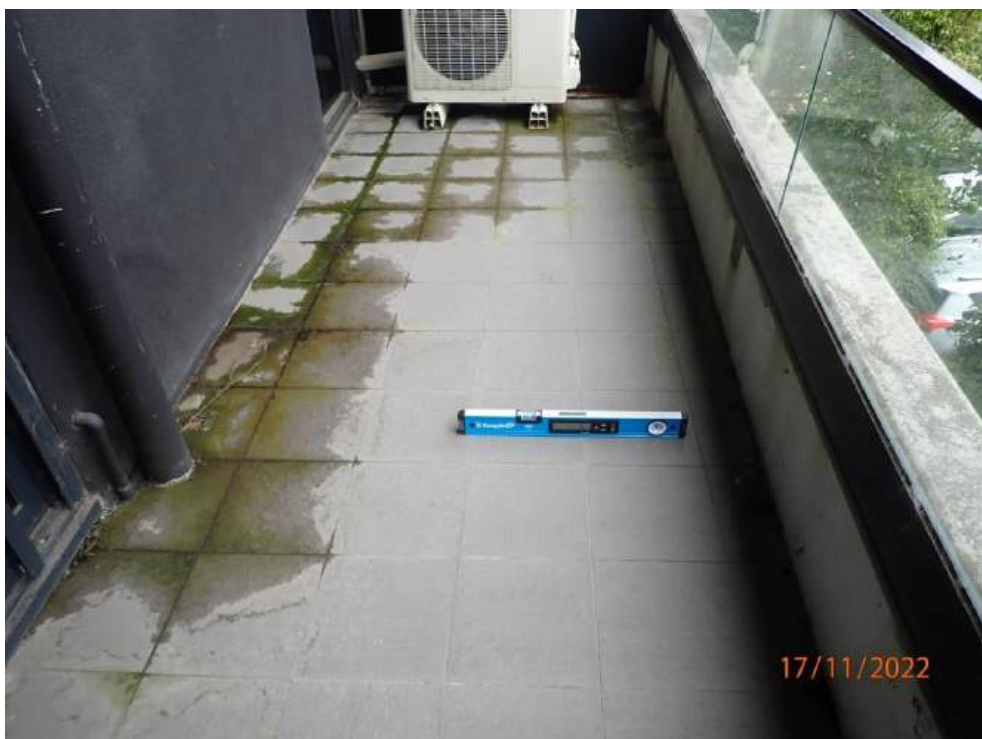
Photograph 14 - Apartment 308A balcony fall
