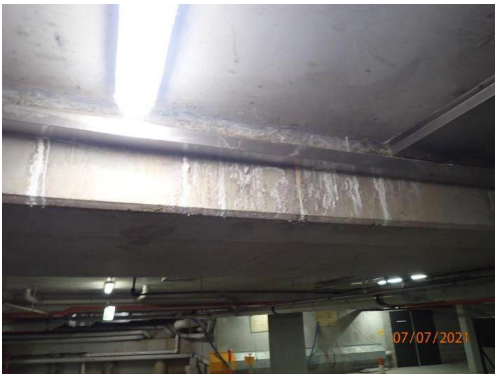
Photograph 30 – Efflorescence and calcification near carpark 48 including surrounding carparks
