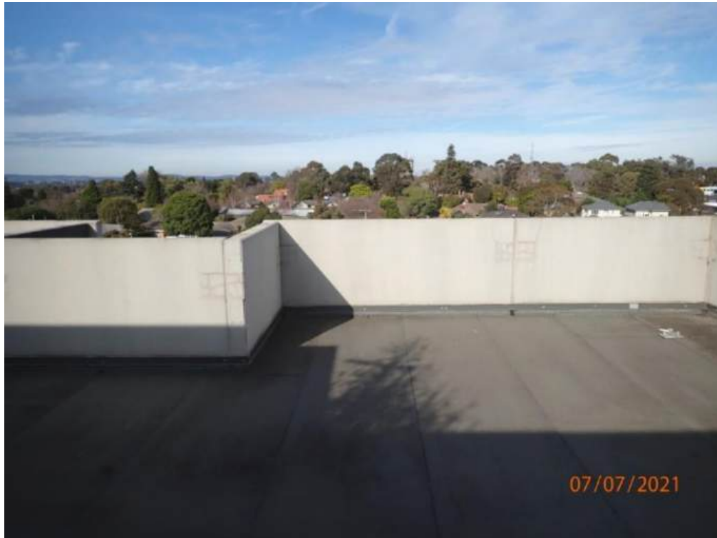
Photograph 111 – Fill is cracking away at tension plates
