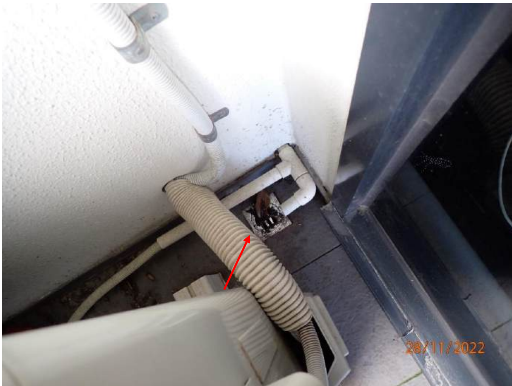
Photograph 88 - Apartment 431B balcony, drainage outlet
