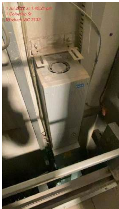
Internal lift shaft, slurry to lift drive
