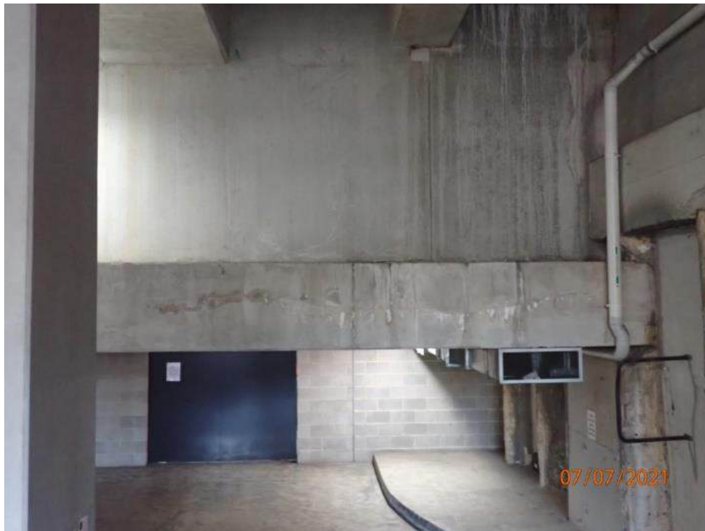
Photograph 68 - Efflorescence and calcium build up to the east end of basement carpark
