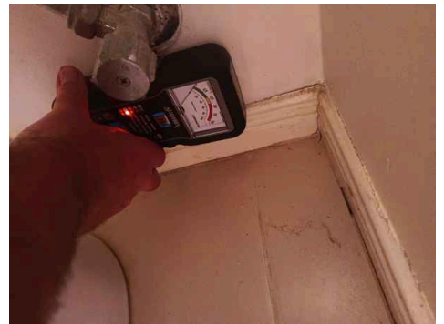
Toilet: Moisture reading to wall at toilet water supply tap
