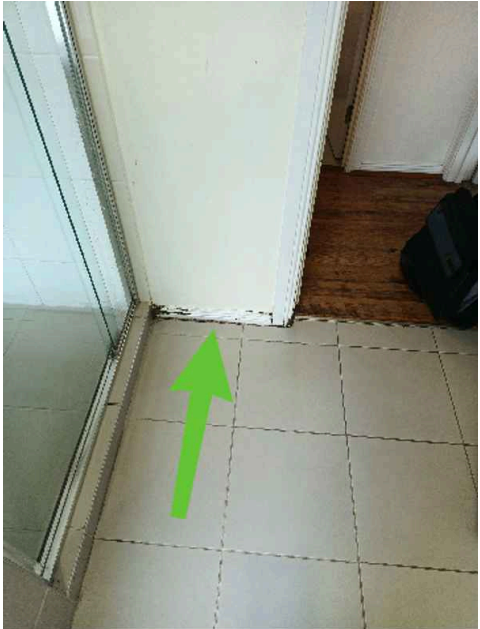
This wall will need to be repaired
